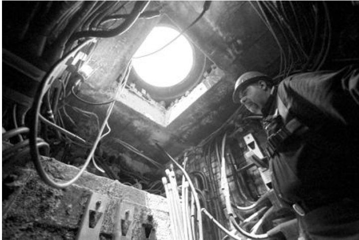
Figure 2 This image was taken inside a manhole on lower Broadway in Manhattan in 2009. Source: (Little 2009).
