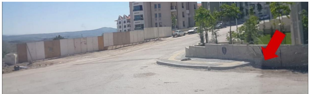
Figure A.7. Misapplication of tactile paving for partially sighted people.
