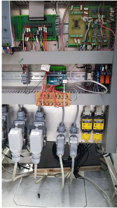
Figure 3.22: Front view of the rack cabinet
