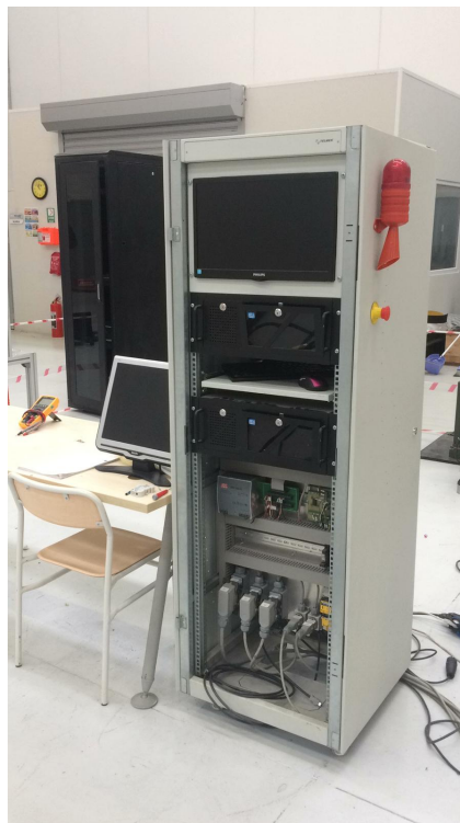
Figure 3.24: Photo of the rack cabinet
