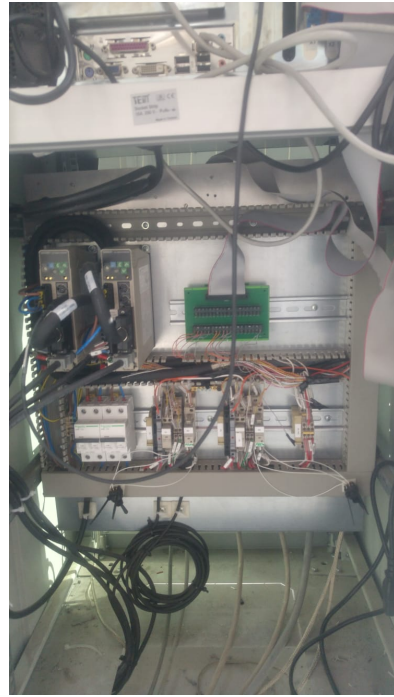
Figure 3.23: Rear view of the rack cabinet
