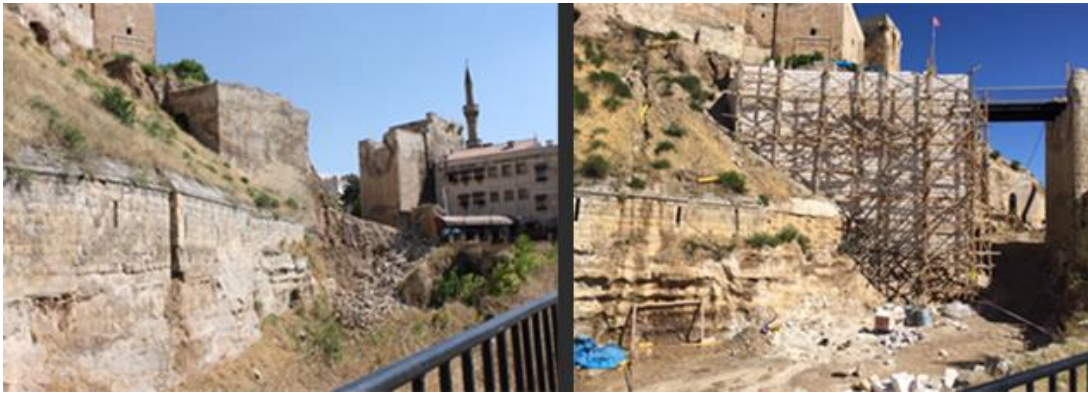
Figure 4.13. Gaziantep Castle before the Renovation (left) and During the Process (right) (Source: Kültür Varlıkları ve Müzeler Genel Müdürlüğü, 2019)
