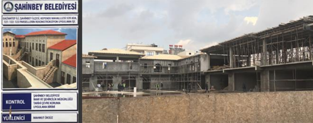
Figure 4.70. Ongoing Construction of Commercial Entity with Underground Car Park (Photos taken by the author, 2019)
