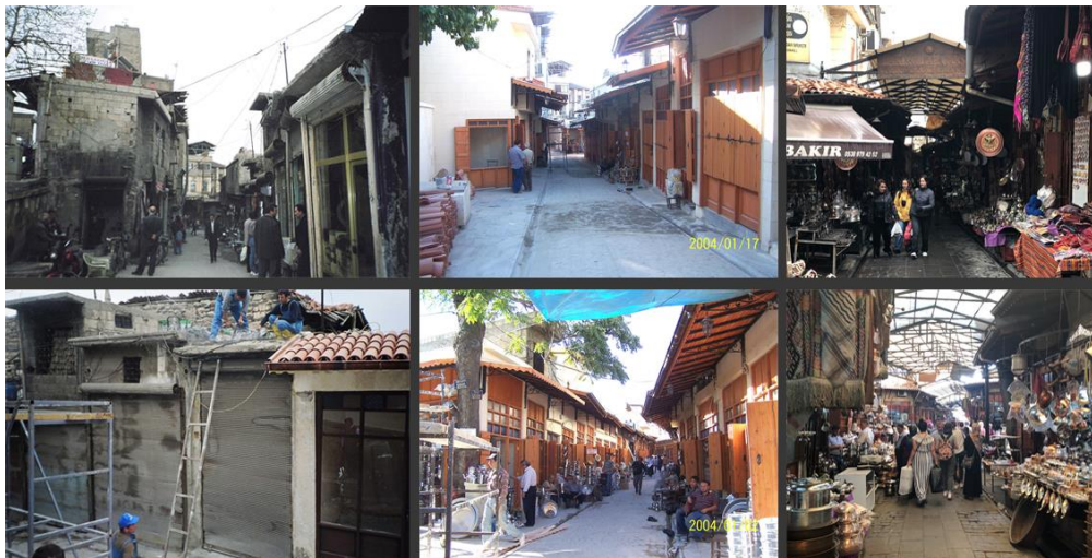
Figure 4.30. Adaptive Reuse of Traditional Structures as a Bakırcılar Bazaar; before the intervention (left), during the process (middle) (Kutay İnşaat, 2019) and after the process (right) (After period photos taken by the author, 2019) Under the Leadership of Gaziantep Metropolitan Municipality
