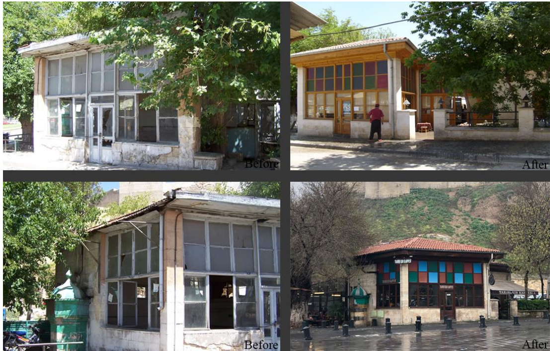
Figure 4.24. Renovation of Historical Coffee House (Source: Kutay İnşaat, 2019 and right bottom photo taken by the author, 2019)
