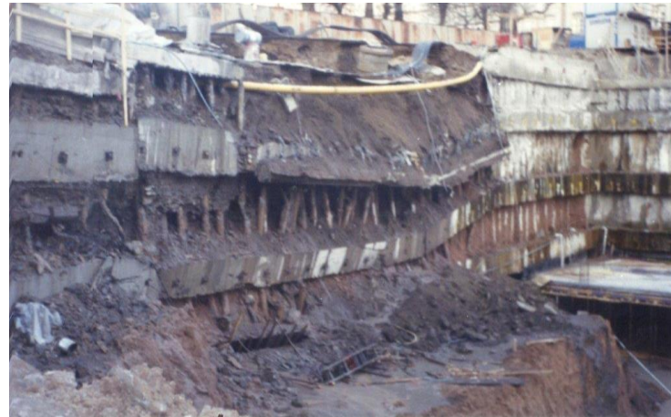
Figure 1.2. Deep Excavation Failure in Ankara a). Before the Failure b). After the Failure (Çalışan, 1994)
