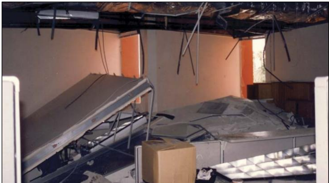
Figure 1.2. Out-of-plane Failure of Office Drywall Partitions in the 1994 Northridge Earthquake (Reitherman, 2010)
