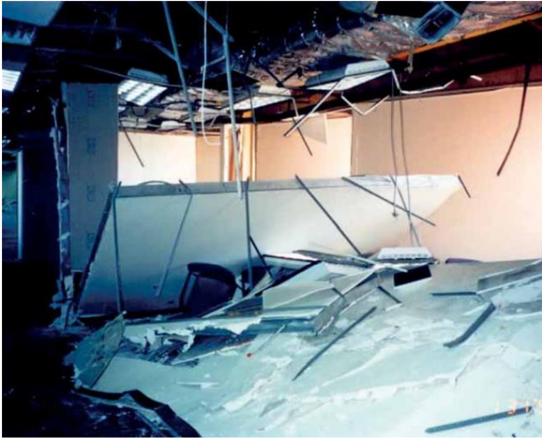
Figure 2.9. Out-of-plane damage owing to inertial forces (Reitherman, 2010)
