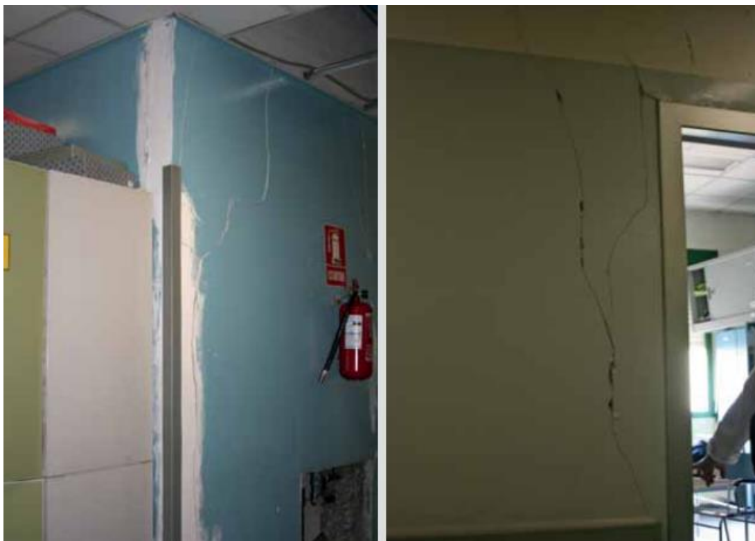
Figure 2.8. In-plane damage owing to building deformation (Fiorino et al. , 2015)
