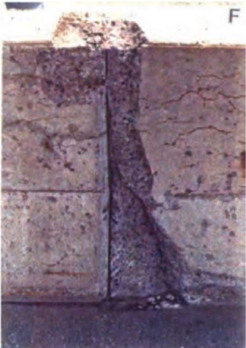
Figure 13. Cracks in joint of concrete members as a result of the high stress concentration occurrence because of ASR [6]
