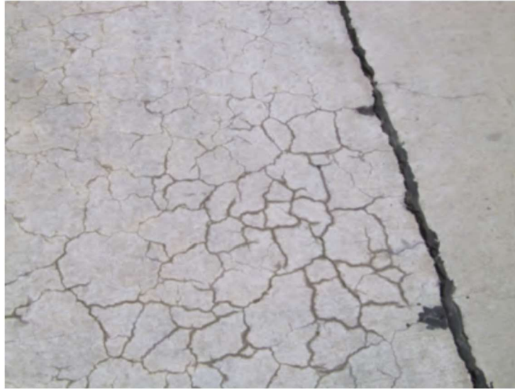
Figure 14. Popped out sealing material at the pavement joint [6]
