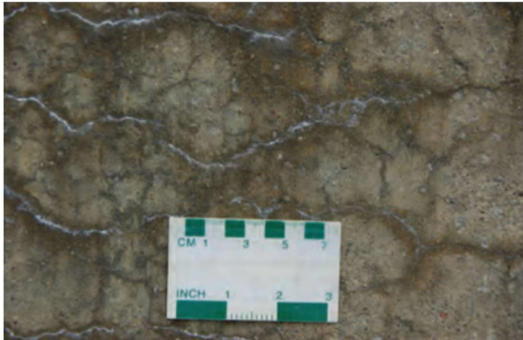
Figure 16. ASR gel exudation and discoloration on the surface of concrete [6]
