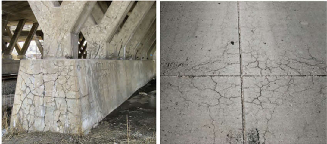
Figure 6. ASR damaged concrete photographs [6]
