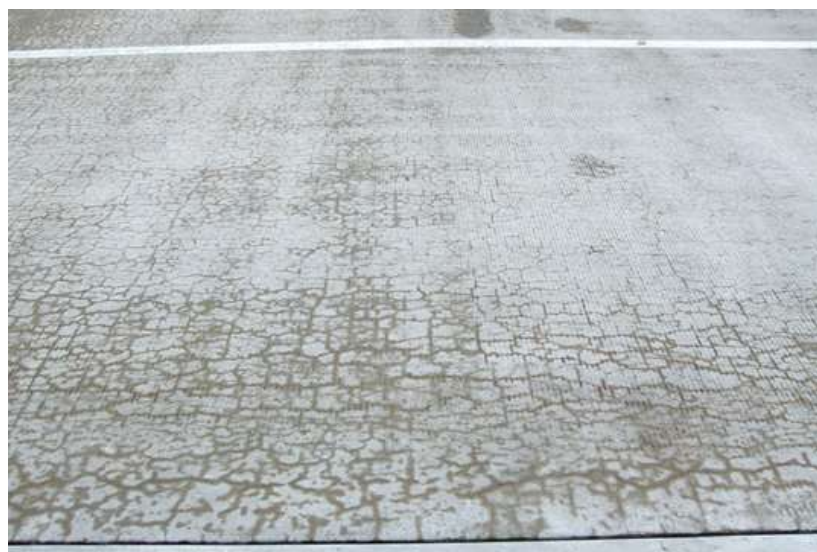
Figure 11. Concrete airfield pavement map cracks with discoloration [13]
