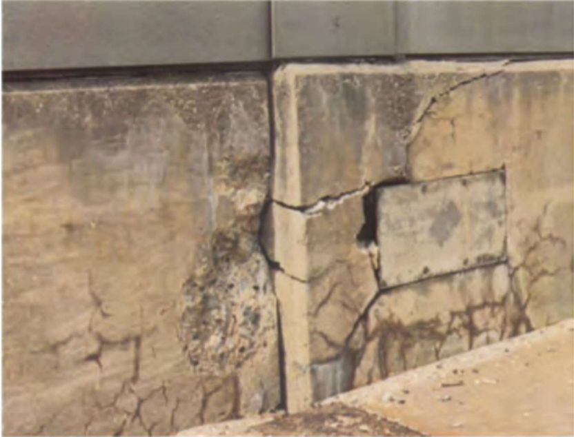
Figure 12. Movement of concrete members because of ASR [6]
