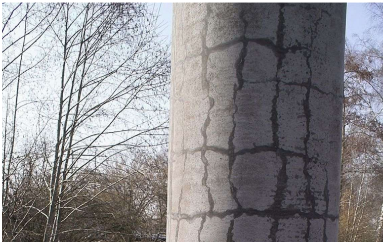
Figure 5. ASR damage on the drying concrete surface of bridge pylon [5]
