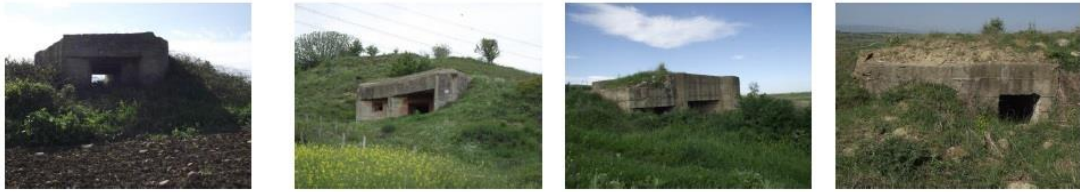
Figure 3.3 Vertical movement of the bunkers, Photographed by author on 05/2019
