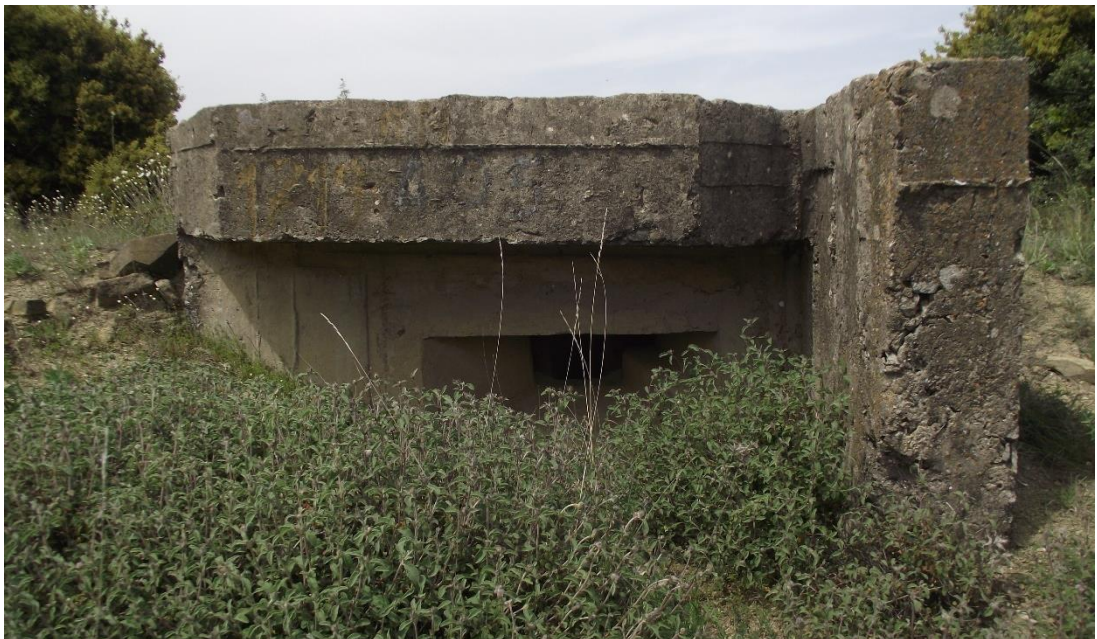
Figure 4.10 Bunker Type 2, side view photo with eaves, extension and side entrance Photographed by the author on 27/04/2019
