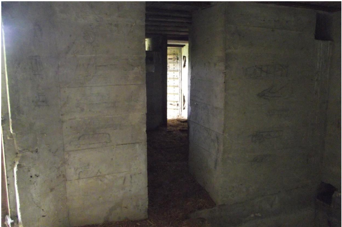
Figure 4.21 Bunker Type 4, entrance from the main hall, Photographed by the author on 25/04/2019
