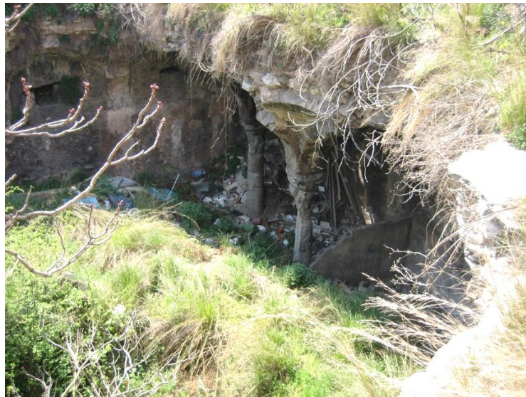
Figure 56: The Current Condition of the Subterranean Cistern Nearby the Stoudios Monastery (Credit: © Jesse W. Torgerson, Wesleyan University. 2007)
