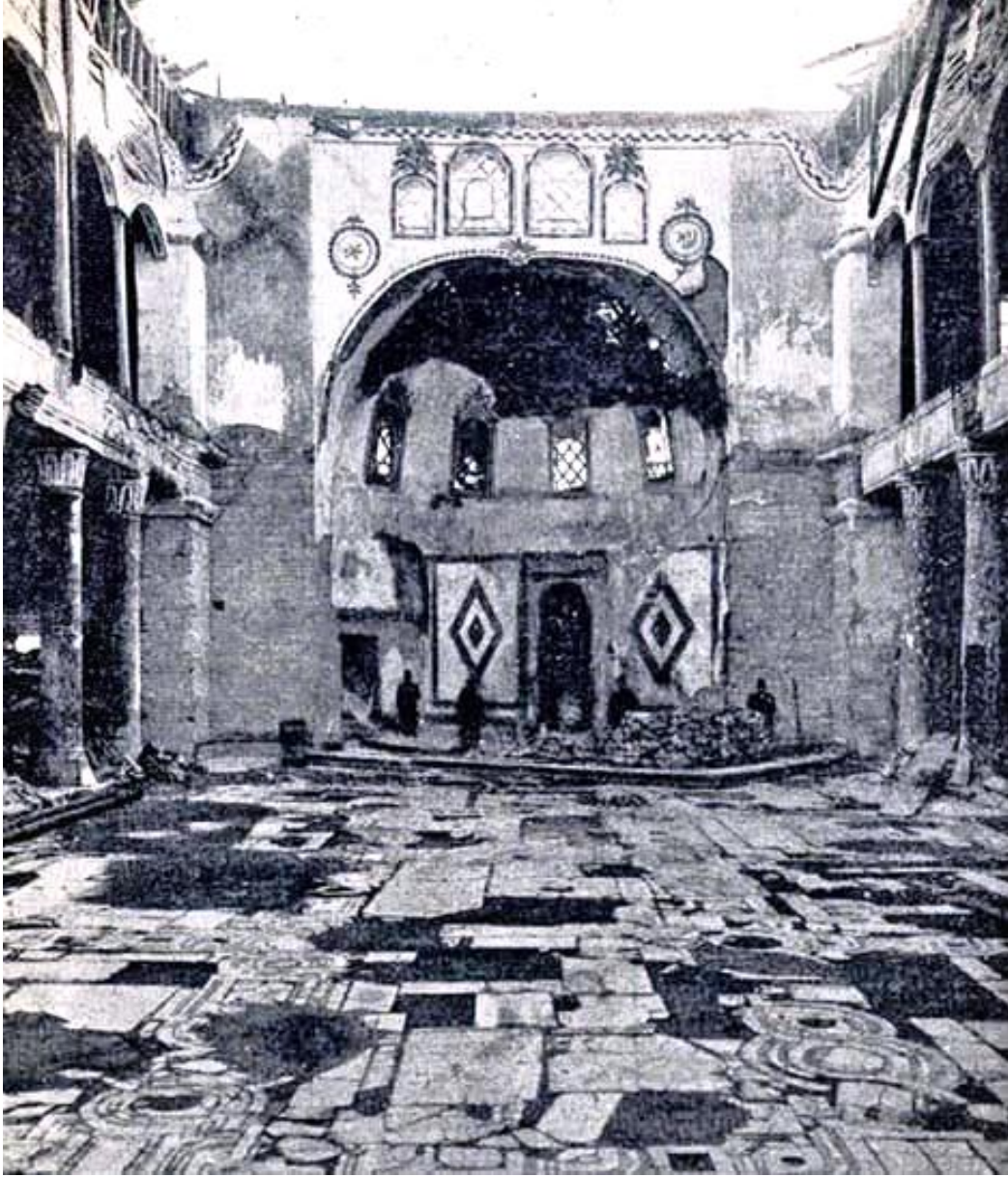
Figure 7: The View of the Apse from the Nave, After the Roof Collapsed, 1920 (Source: Köse, 2012, 37)
