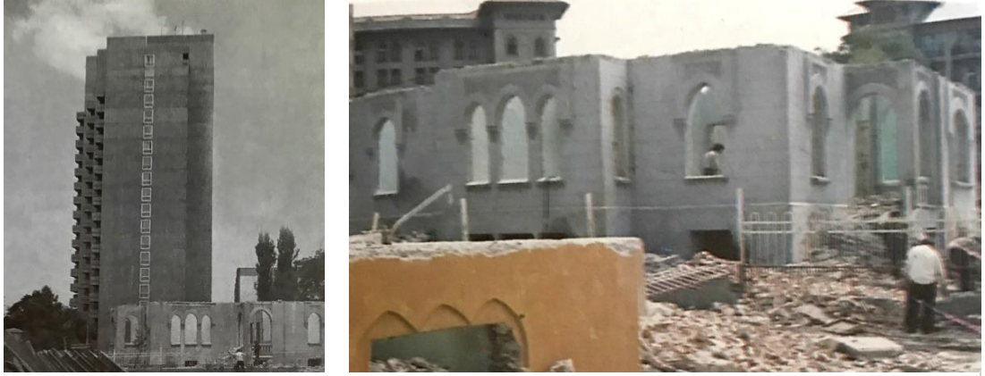
Figure 3.44: Demolition of Pious Houses before construction of Turkish Central Bank Headquarters, Summer of 1973.
