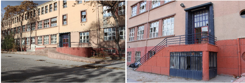
Figure.E.2. The exterior stairs of the G Block, 2013 (Source: Azize Elif Yabancı's personal archive)
