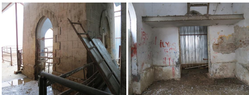
Figure 3.132. Exterior and interior damages of the water tower
