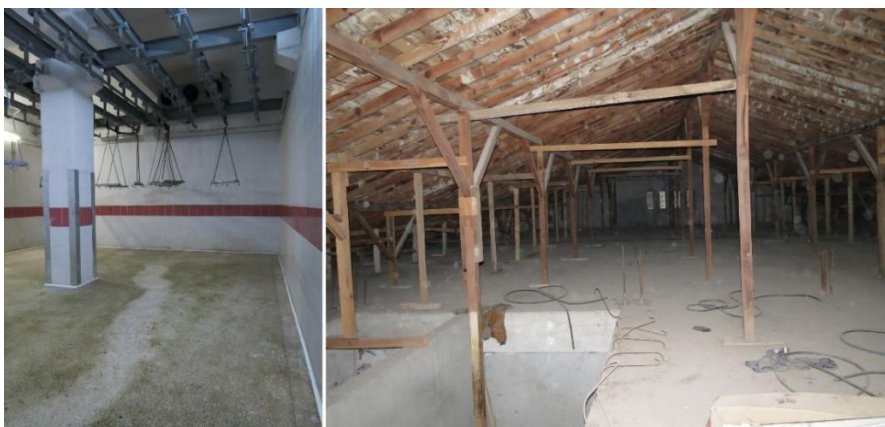
Figure 3.119. Interior of the depot (on left) timber frame structure observed in the attic (on right)
