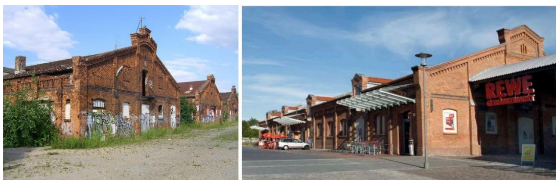
Figure 2.24. Before and after the restoration of the cattle barns of Berlin slaughterhouse (Source: http://www.leisering-berlin.de/referenzen/zentral-vieh-und-schlachthof-berlin )
