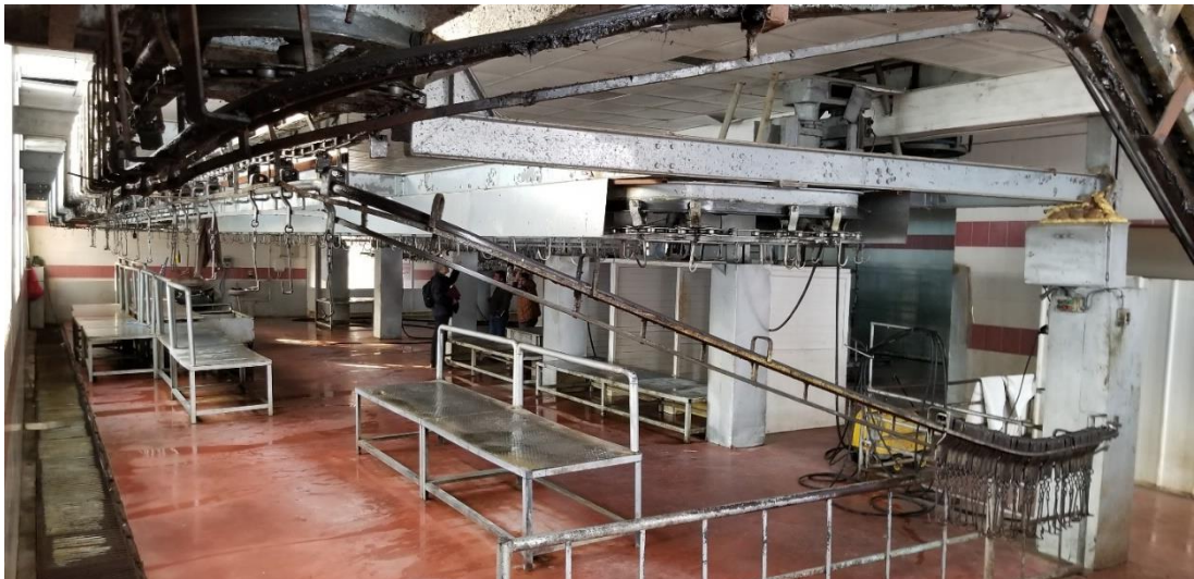
Figure 3.110. Interior view of the slaughterhouse showing ovine monorails
