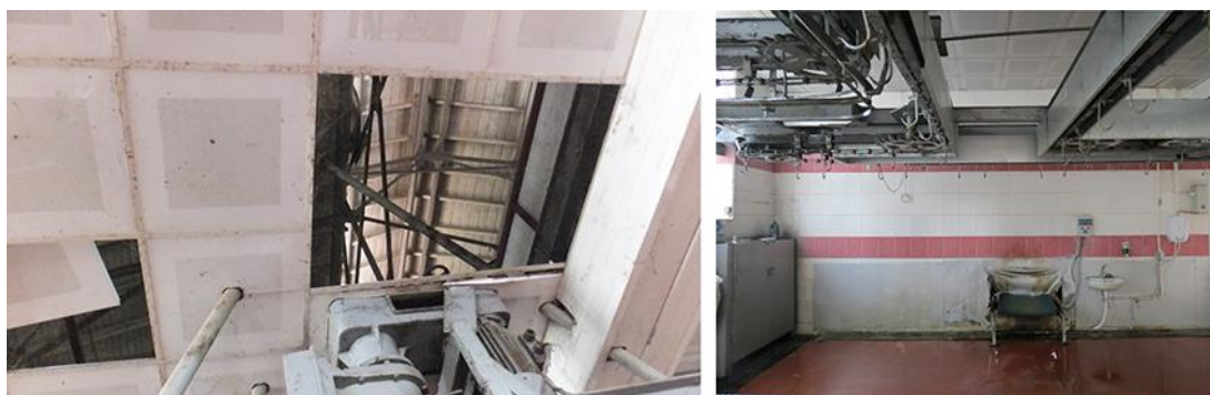
Figure 3.91. Original roof construction visible behind the suspended ceiling (on the left) and the conveyor on the west wall (on the right)
