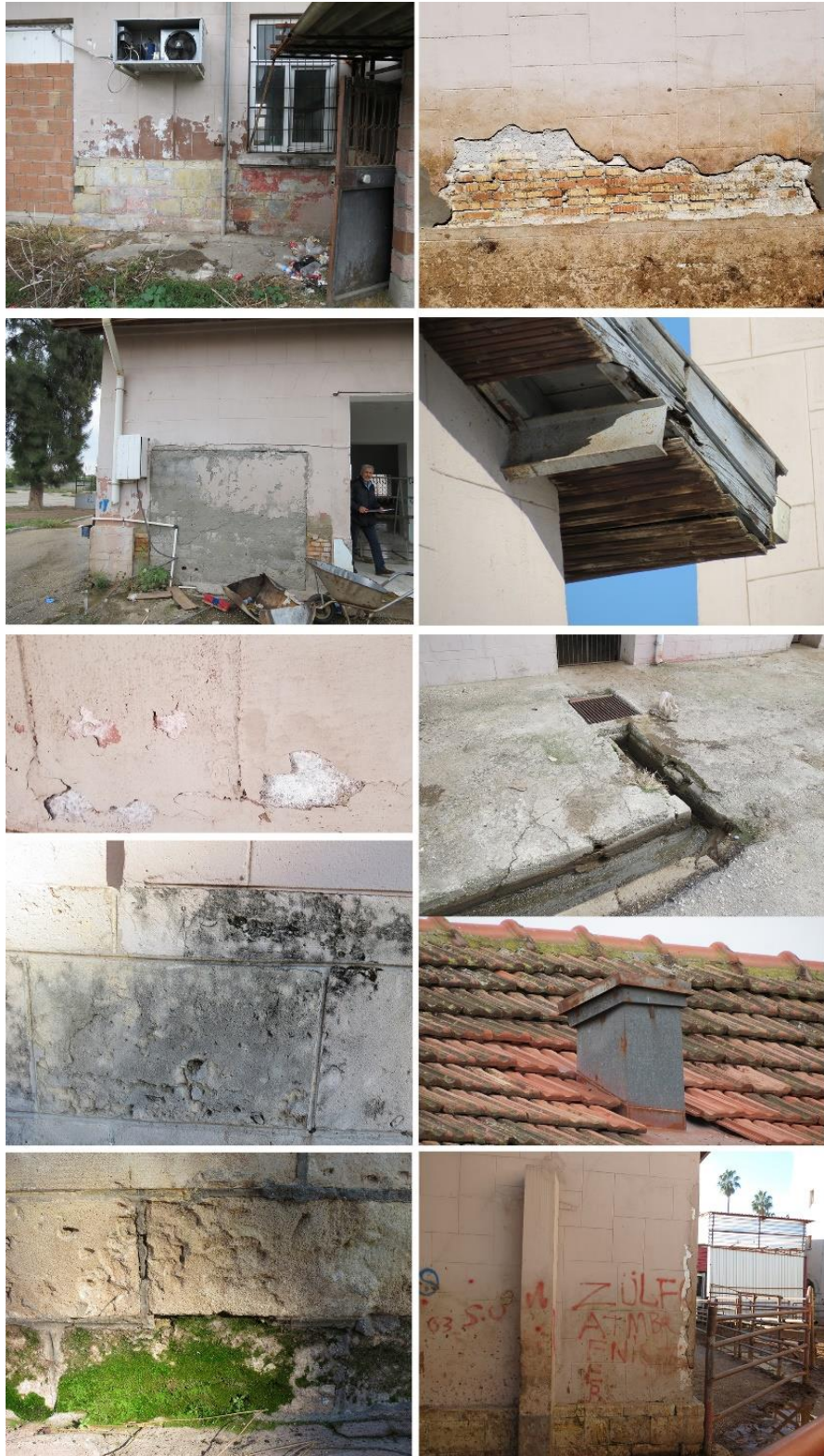
Figure 4.13. Most common problems detected inside the complex
