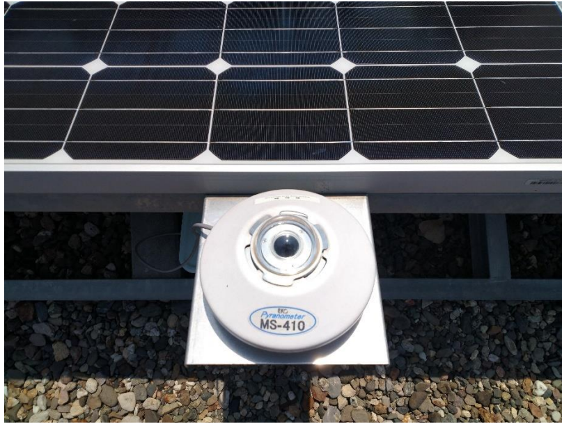
Figure 4-3. Pyranometer Used in Representative Site
