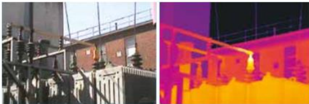
Figure 1.3. Detection of unwanted high resistance connections in transformer substation with using LWIR camera [3]
