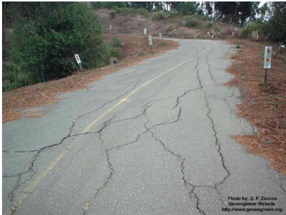
Figure 1-3. Soil and pavement cracks in swelling ground ( https://www.geengineer.org )
