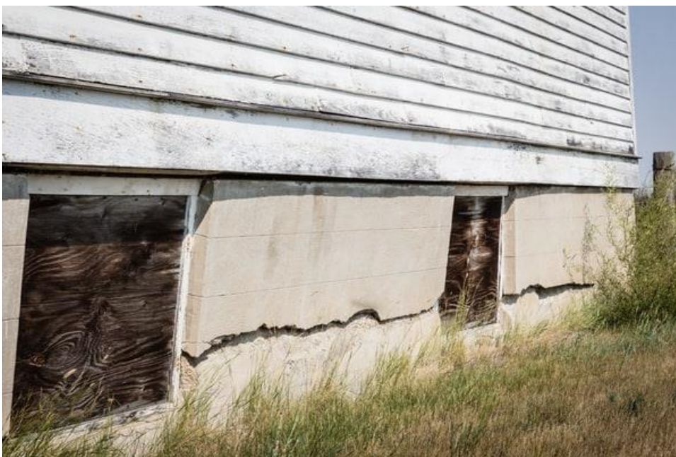
Figure 1-2. Expansive soils and foundation damage ( https://www.njdrybasements.com/ )
