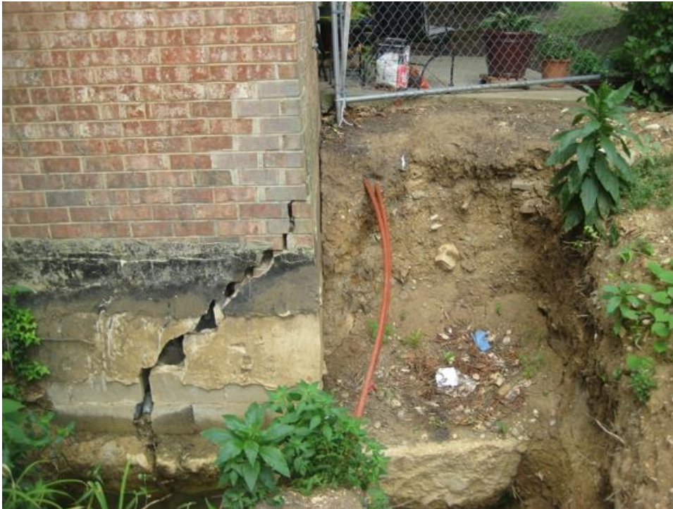
Figure 1-1. Cracked foundation ( http://www.etc-web.com/screw-it/ )
