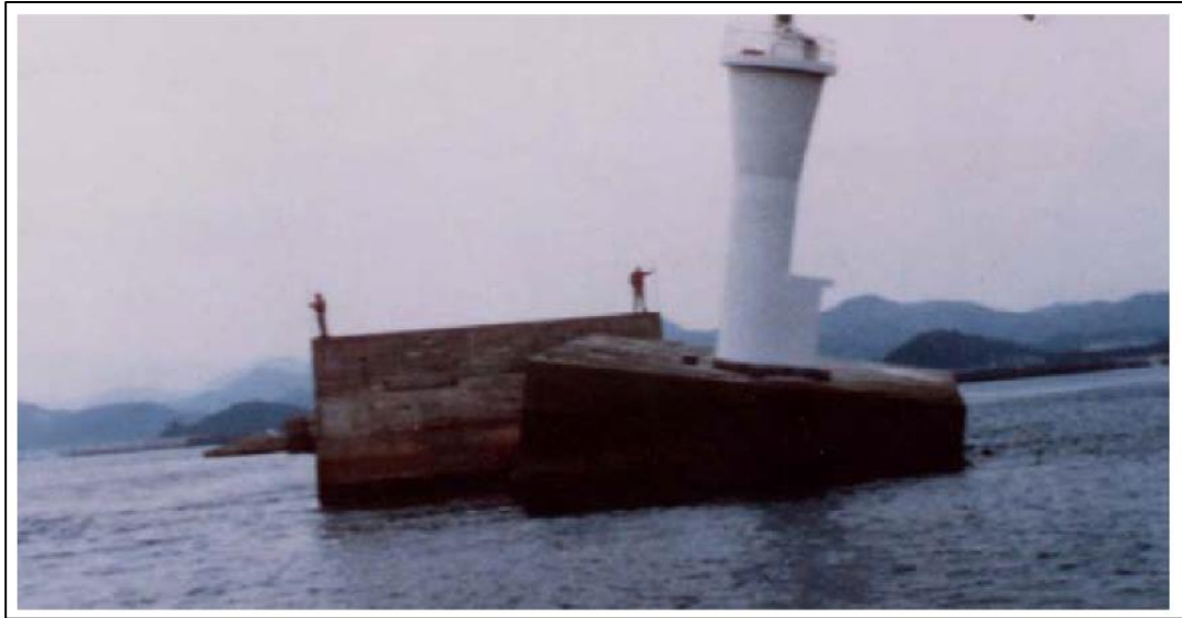
Figure 2.2. Damaged breakwater head of Sendai Port under Typhoon 9119 (19th typhoon in 1991) (Kim 2009)
