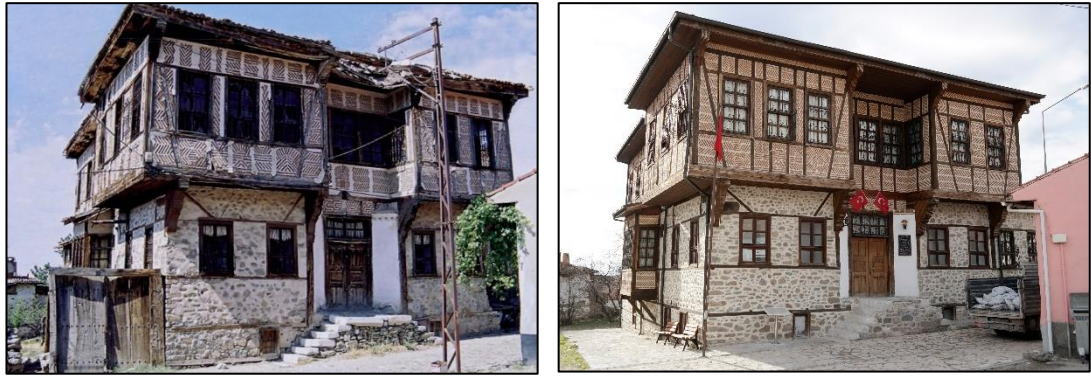
Figure 4-59 Zaimağa Mansion before the Restoration (left) (www.sivrihisar.web.tr retrieved in December, 2019), Zaimağa Mansion after the Restoration (right) (Author, December, 2017)
