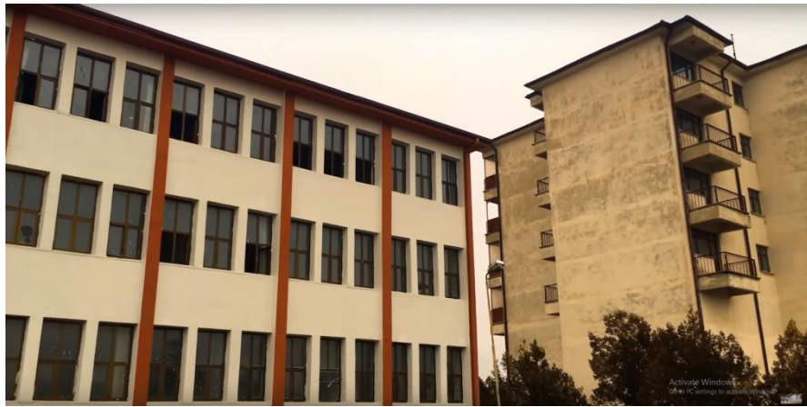
Figure 4-25. First stages of the renovation process Source: Chamber of Architects Ankara Branch archive (2018)
