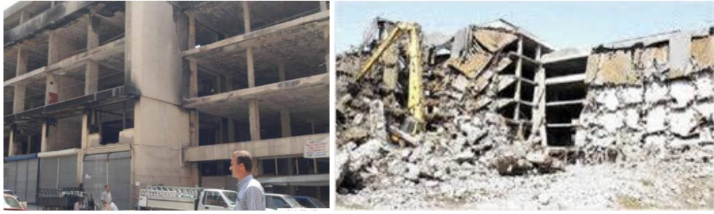
Figure 2.12. The condition of Modern Çarşı after the fire (left) and the demolition of the structure (right) (Source: (left) https://www.labmedya.com/show_file.php?attachid=41 , (right) https://tuncerurban.files.wordpress.com/2013/03/1.jpg )
