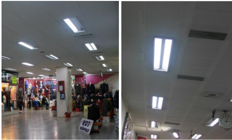
Figure 3.54. The suspended ceilings and the air grating panels on the ceilings (Author, 2018)
