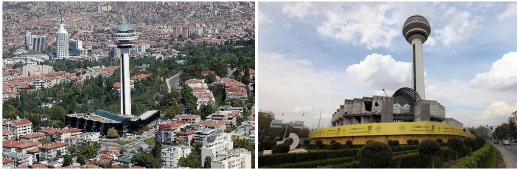
Figure 2.13. Atakule before the demolition of the shopping block (left) and the demolition works (right) (Source: (left) https://www.sabah.com.tr/ekonomi/2018/10/09/300-milyon-liralik-yatirimla-yenilenen-atakule-29-ekimde-acilacak , (right) http://www.hurriyet.com.tr/yeni-ruhsata-yeni-dava-27455780 )
