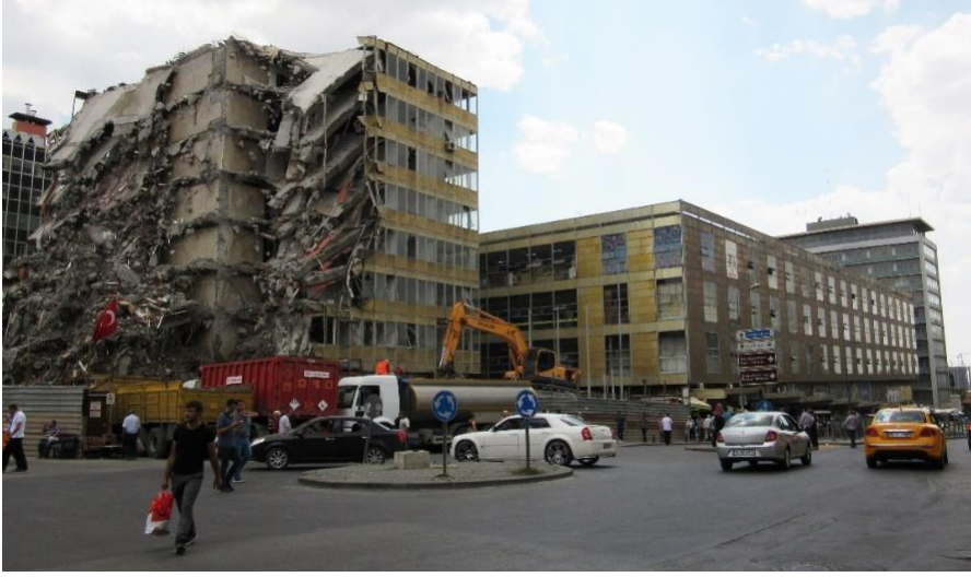
Figure 1.1. The demolishment of the high-rise office block of Anafartalar Çarşısı Complex (Author, 2018)
