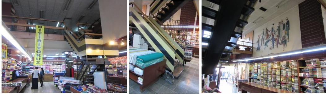
Figure 3.33. The original elements in the shops that have entrance from the street; the mezzanine, timber railings and staircase, floor finishing and suspended ceiling (Author, 2019)
