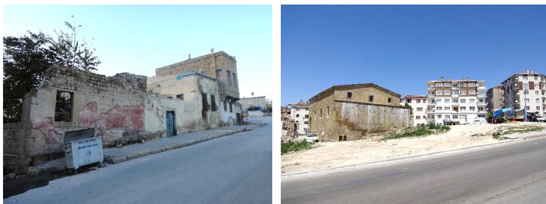
Figure 3.14. Demolition of the traditional fabric around H. Stephanos Church (before and after photographs taken at the same location in 2010s, Personal Archive)
