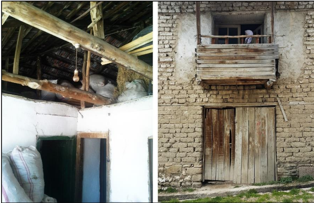
Figure 150: The discoloration problem on the timber elements. The photo on the left is taken from H5 and the photo on the right is taken from the H15.
