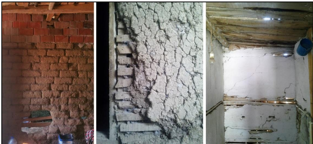
Figure 149: The material loss on the mud brick masonry and timber-framed walls. From left to right, the photos are taken from H3, H4 and H15.
