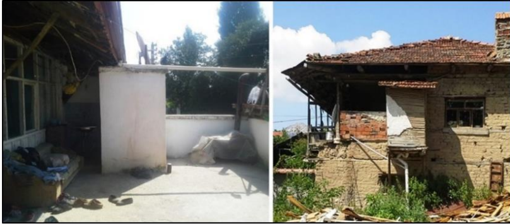
Figure 46: The photo, taken in the H6, shows the additional toilet constructed on the 'saçak'; the photo, taken in the H16, shows the additional toilet constructed adjacent to the 'sofa'.
