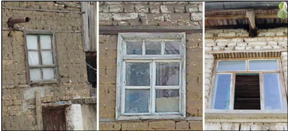
Figure 67: The most frequently used original window types. The image on the left is produced by utilizing the study ‘Understanding a Historic Rural Landscape in Relation with an Archaeological Site: Ağlasun/ Sagalassos’ 12 ; the photo in the middle is from the H8; the photo on the right side is from the H15.
