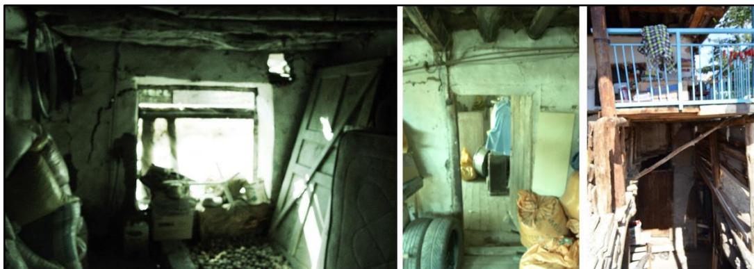
Figure 48: Photos, taken in the H7, shows the spaces on the mezzanine. The photo on the left and the one in the middle shows the room which was used as a guestroom and production space. The photo on the right shows the entrance door of the room used as a storage.
