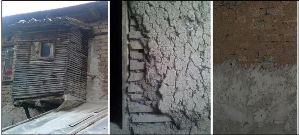
Figure 84: The first photo from H11, shows the 'bağdadi' covering system over the timber frame structure; second one from H4, shows the mud brick plaster on the 'bağdadi' covering; the last one from H2 shows the cement plaster application on the mud brick masonry wall.
