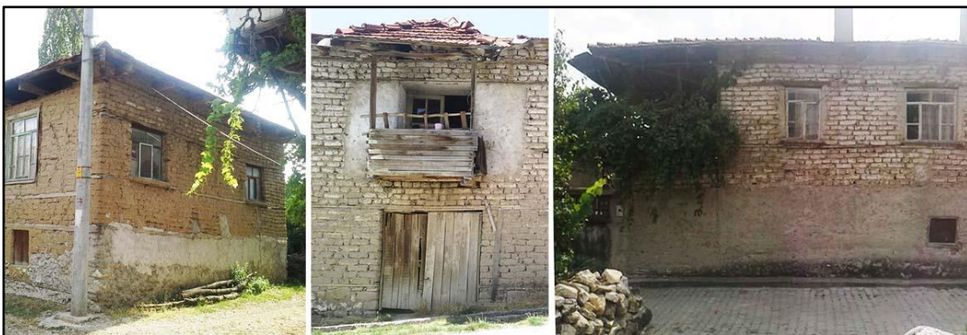
Figure 77: The photos from H4, H15 and H9 show partial plaster on their facades.
