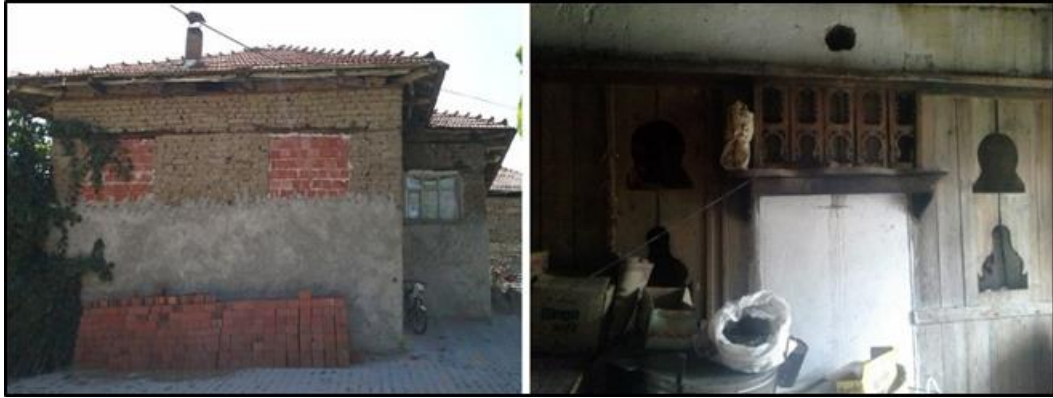
Figure 127: The photo from the H2 on the left shows the removal of the window frames and closing the openings with hollow bricks; the photo from the H7 shows the closed traditional fireplace.
