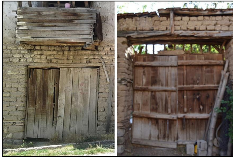
Figure 64: On the left, the entrance door to the ground floor of the main building in the H15; on the right, the entrance door to the courtyard of the H7.
