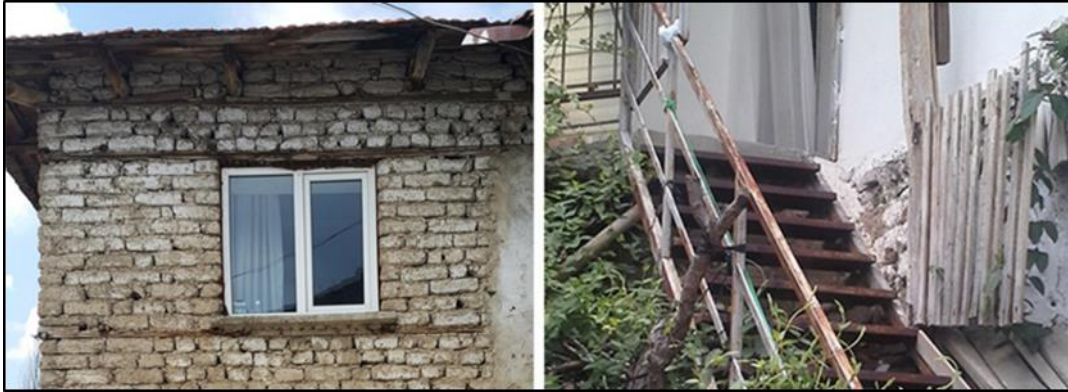
Figure 129: The photo on the left from H15 shows the replacement of the wooden frame window with the PVC. The one on the left one from H14 shows the structural and material change of the wooden staircase with the steel one.
