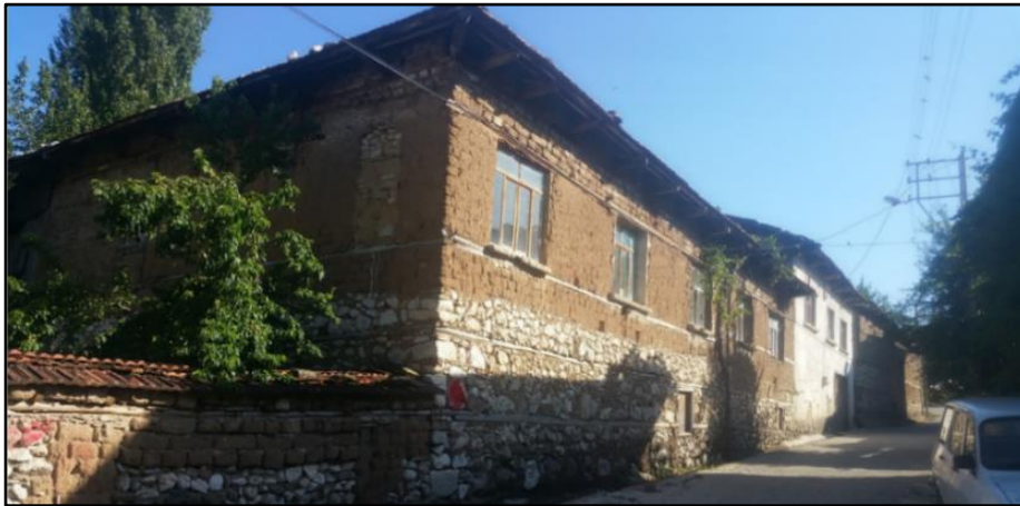
Figure 17: The street view showing traditional mud brick masonry houses, located adjacently, in Ağlasun and the house with the stone masonry, constructed up to the first floor level.
