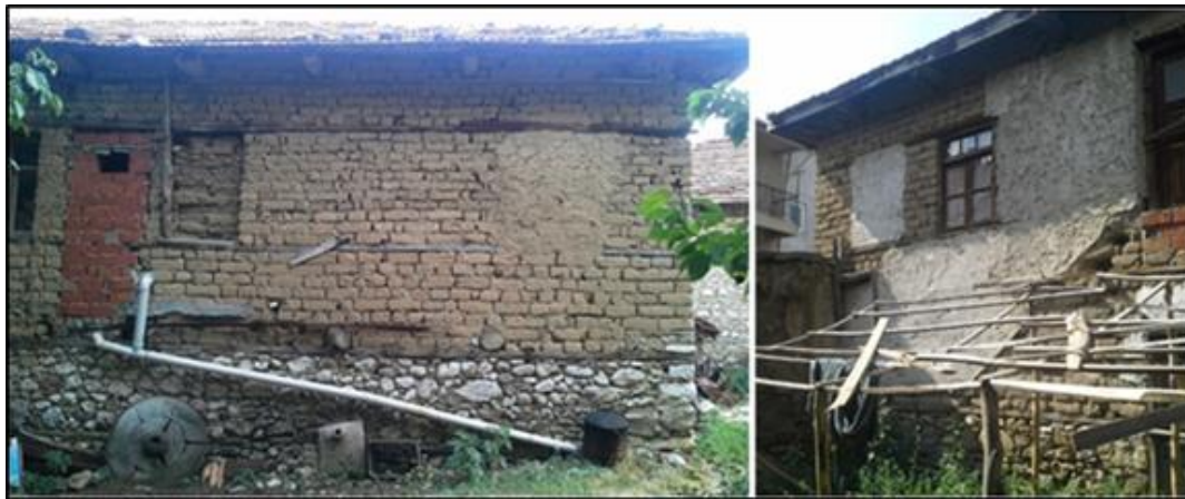
Figure 130: The photo on the left from H5 shows the decommissioning of two window openings and a door opening by using both hollow bricks and mud bricks as infill materials. The one on the right from H8, shows partial cement plaster on the facade.
