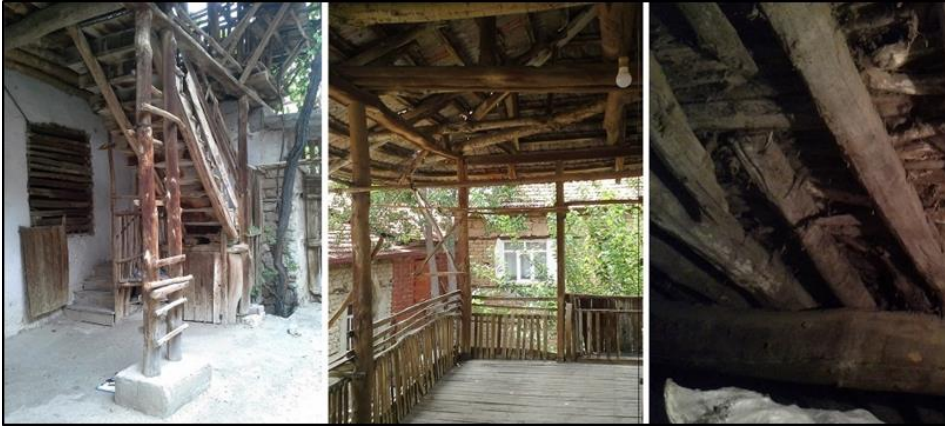
Figure 82: From left to the right, the timber posts carrying the 'sofa'; timber posts carrying the roof structure; timber elements of the flooring system named 'döver', 'mertek' and 'pargı' from bottom to top (H19).
