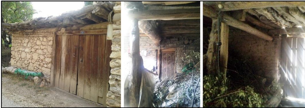
Figure 57: The photos from the H4 show the authentic entrance door of the original 'saçak' and views from inside of it.
