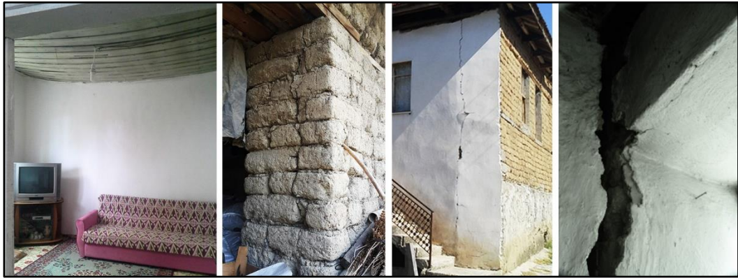
Figure 148: The photo on the left shows the sagging on the ceiling. The others show the structural cracks on the masonry walls. From left to right, the photos are from H14, H15, H3 and H7.
