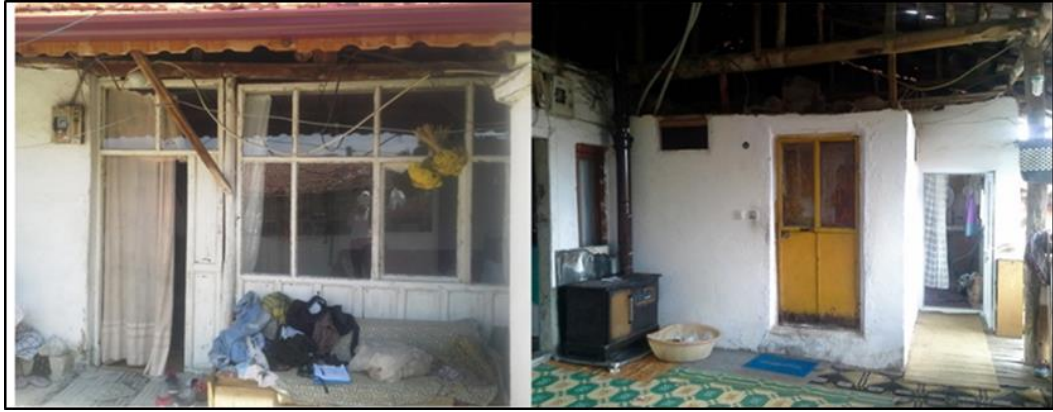
Figure 135: The photo from H6 on the left shows the 'sofa' which was closed later. The one on the right from H13 shows the toilet in front of the kitchen, which are both constructed with additional walls on the open 'sofa'.
