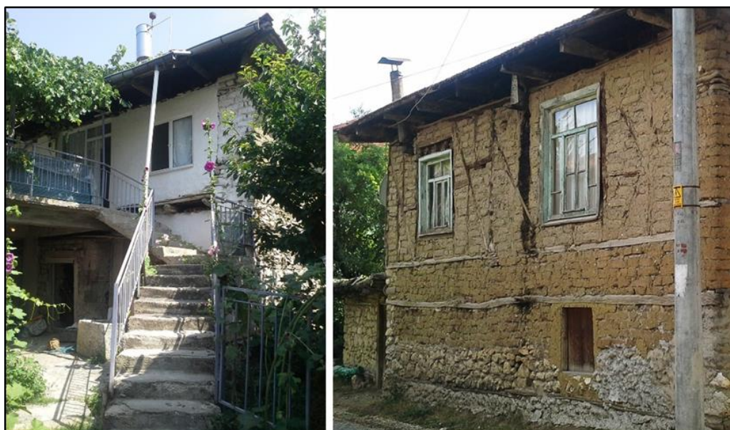
Figure 123: The photo from the H12 on the left shows the reinforced concrete 'saçak' structure and the stairs which were constructed after the removal of the earthen 'saçak' structure and the wooden staircases; The photo from the H4, shows the timber-framed wall constructed after demolition of the mud brick masonry wall on the first floor of the house.
