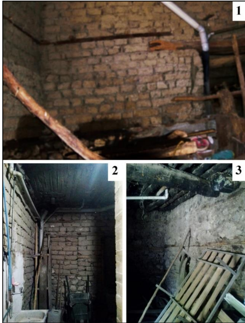
Figure 151: The first photo from the H19, shows the mud brick masonry wall exposed to water leakage from the pipe; the second photo from the H9 shows the condition of the drainage piping system and its physical relation with the mud brick masonry wall and reinforced concrete slab; the third one shows the relation between the water pipe and the traditional flooring system.
