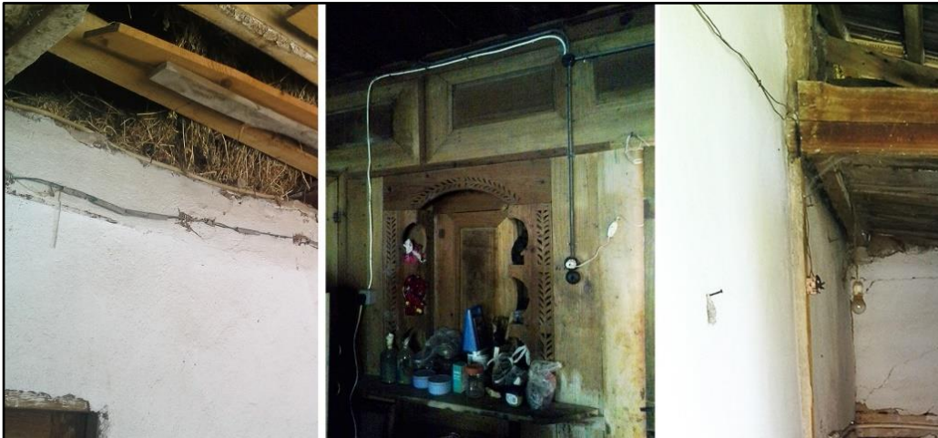
Figure 152: The photos show the electric cables in poor condition without any isolation. From left to right, the photos are from H5, H7 and H15.
