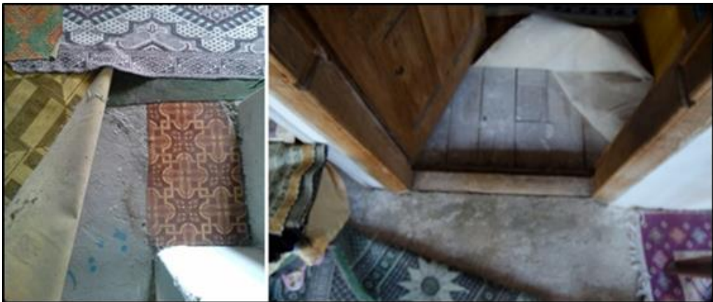
Figure 128: Both two photos shows the additional screed layer on the floorings. The one on the left is from H15; the one on the right is from H19.
