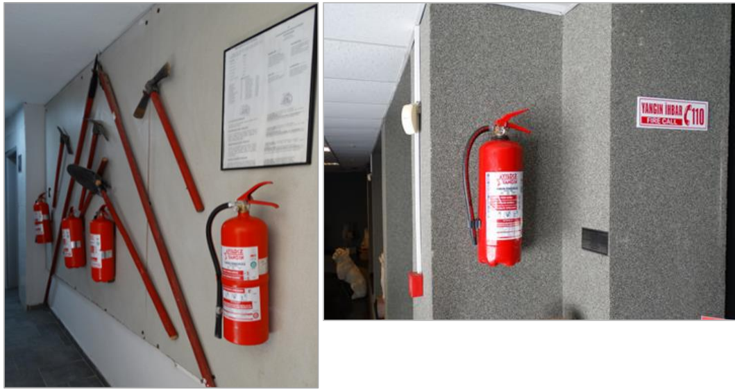
Figure 4.16 Fire instructions and equipment on the outer wall of the museum and fire alarm system in the museum (taken by the author at Bergama Museum, 2019)
