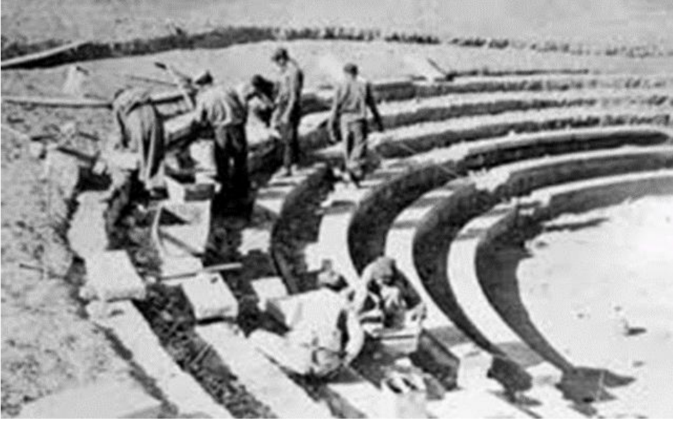
Figure 5.12. While students from Kepirtepe High Village Institutes were participating in production process of amphitheater
