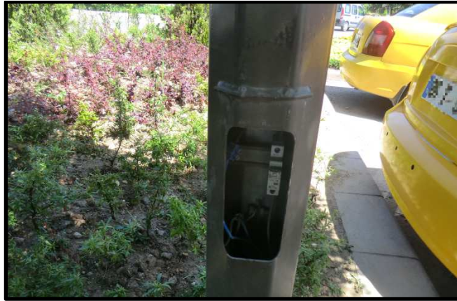
Figure 4.35. Damaged Electric Pole
