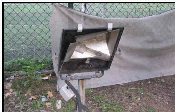
Figure 4.34. Broken Lighting Element
