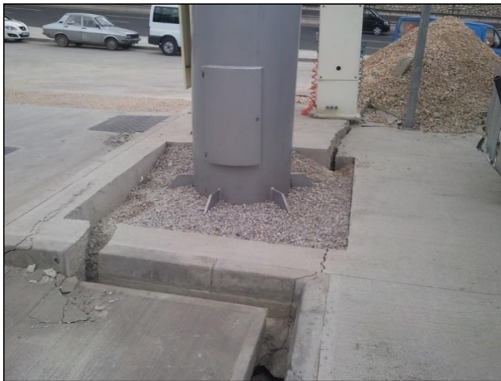
Figure 4.9. Crack formations observed in the gas station due to the ground deformations caused by the foundation excavation (Bakır, 2011).
