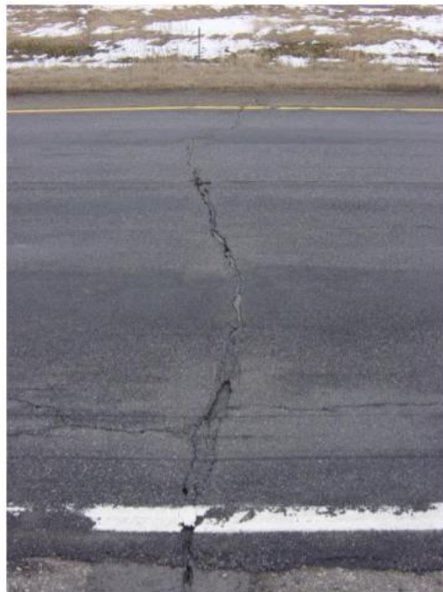
Figure 2.4. Example of large transverse crack (Molenaar, 2007)
