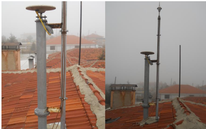
Figure 2.8. Lightning rod mounted on the mast of the GPS antenna at EMIR station.
