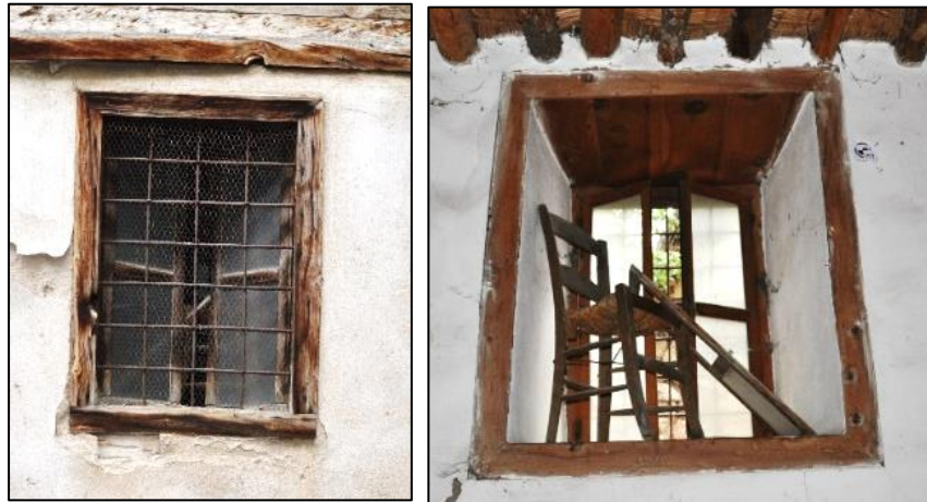
Figure 3.165. Window opening located on stone masonry wall; Type 1 (Kılıç N. b. block-lot: 170-44)
