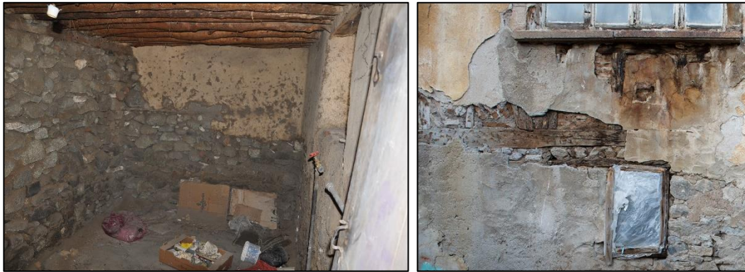
Figure 3.55. Timber floor beams that are located on wall plate of stone the masonry wall; interior view (left), exterior view (right) (Kılıç N. b.block-lot:170-19)
