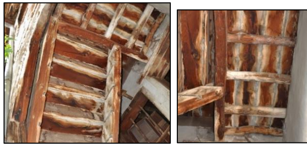
Figure 3.136. Timber step boards that are located on stringers (left), connection detail of stringer and timber beam (right)-Type2A (Kılıç N. b. block-lot: 170-44)
