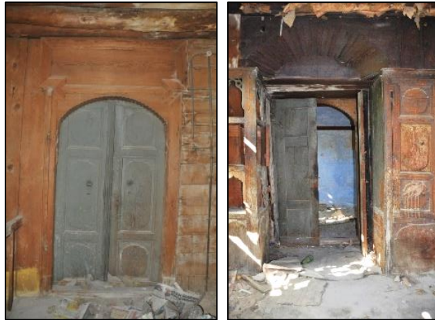
Figure 3.161. Interior double wing arched panel door located on timber framed wall, Type 5; exterior view (left), interior view (right) (Cumhuriyet N. b. block-lot: 433-3)
