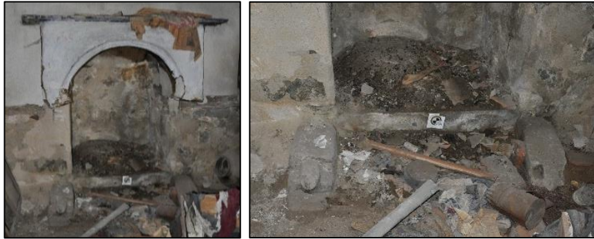
Figure 3.209. Fireplace with projected front face and raised from ground (Type 2B); general view (left); close view at the bottom part of fireplace (right) (Kılıç N. b. block-lot: 170-44)
