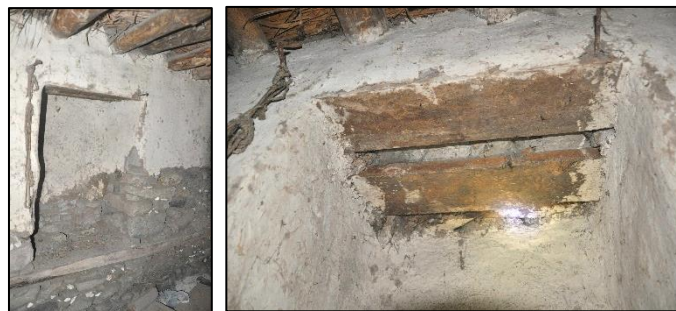
Figure 3.216. Timber lintels located at bottom and top level of niche Type 1A (Cumhuriyet N. b. block-lot: 433-2)
