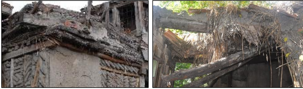
Figure 3.77. View of roof, Type 1 (left, Kubbeli N. b.block-lot: 186-36; right, Cumhuriyet N. b.block-lot: 433-2)
