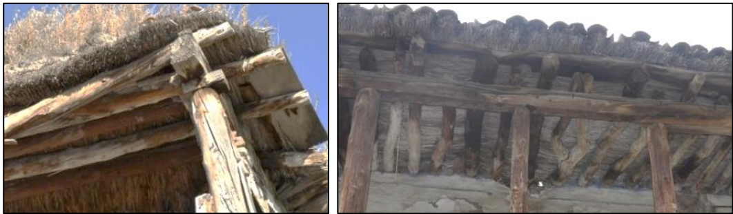
Figure 3.75. View of timber floor beams and reed infill on top of beams in the roof, Type 1 (Kılıç N. b.block-lot: 170-44)
