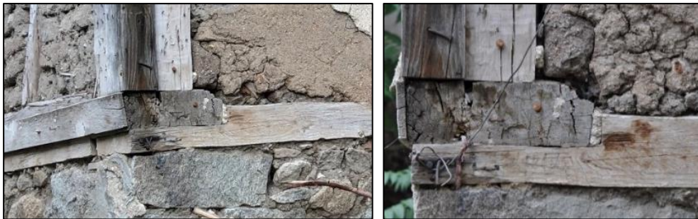
Figure 3.104. Connection detail 2, connection of timber foot plates by half lap joints and nails (Kılıç N. b.block-lot: 170-44)
