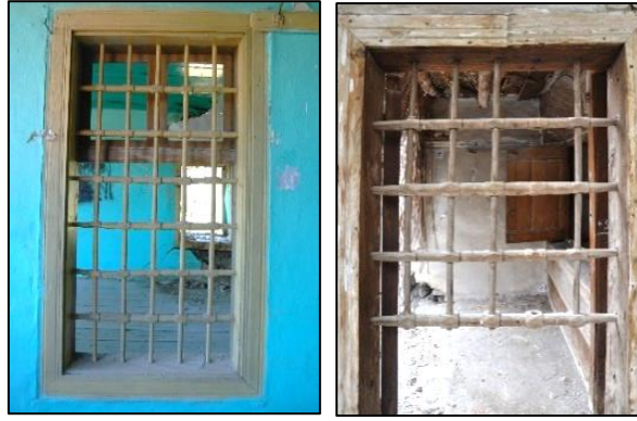
Figure 3.189. Examples of timber railings formed by using lokma (left, (Yenice N. b. block-lot: 11-16; right, Kılıç N. b. block-lot: 170-44)
