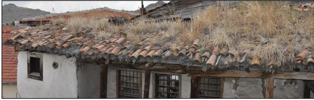
Figure 3.74. View of roof, Type 1 composed of reed infill, earth infill and over&under roof tiles on top of them (Kılıç N. b.block-lot:170-44)
