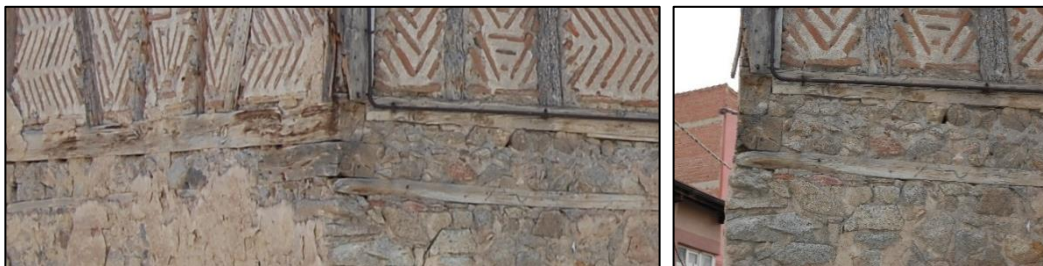
Figure 3.102. Connection detail 2, view of floor beams located over the masonry wall and timber framed wall of upper floor built on the foot plate (Demirci N. b.block-lot:448-2)
