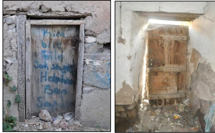
Figure 3.143. Exterior single wing batten door located on stone masonry wall; Type 1, exterior façade (left), interior façade (right) (Cumhuriyet N. b. block-lot: 433-3)
