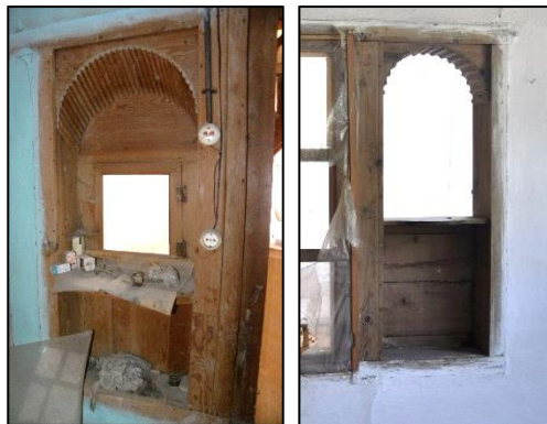
Figure 3.220. Niche with arch and window located on the timber framed wall (left, Camikebir N. b. block-lot: 196-1; right, Kılıç N. b. block-lot: 170-19)
