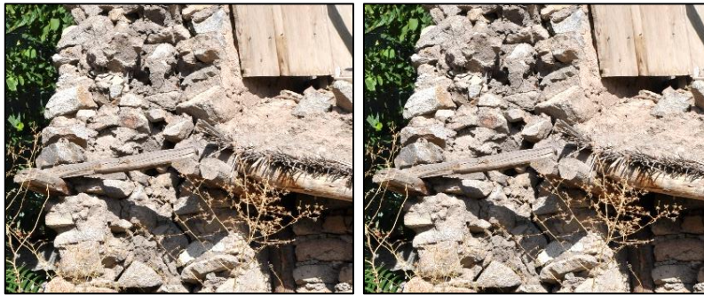
Figure 3.96. Connection detail 1-view of floor beams inserted into wall approximately the thickness of wall plate (Gedik N. b. block-lot: 362-19)
