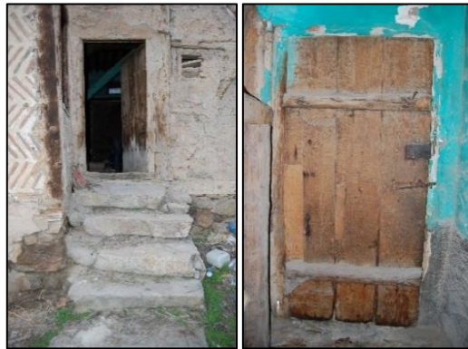
Figure 3.153. Exterior single wing batten door located on timber framed wall, Type 4; exterior façade (left), interior façade (right) (Demirci N. b. block-lot: 448-2)
