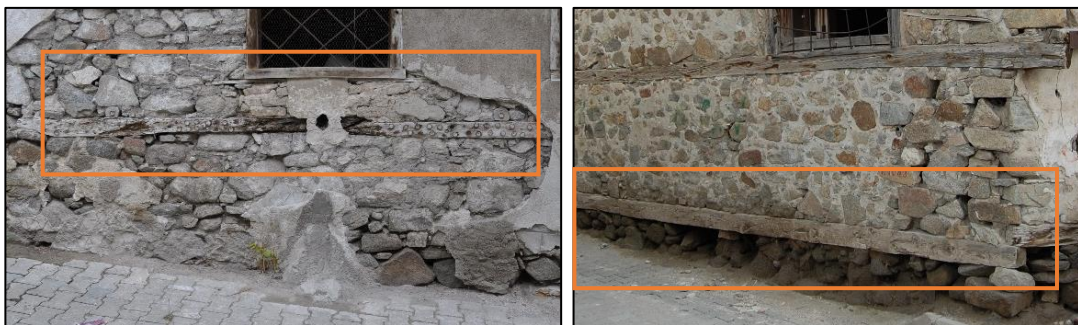
Figure 3.5. Timber lintel between the foundation wall and ground floor wall (left, Camikebir N. b.block-lot: 196-1; right, Karabaşlı N. b.block-lot: 367-13)
