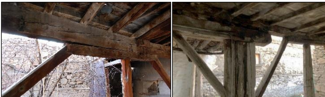
Figure 3.44. Type 2 - timber post with bolster on top (left, Camikebir N. b.block:196-1; right, Kubbeli N. b.block-lot: 186-36)
