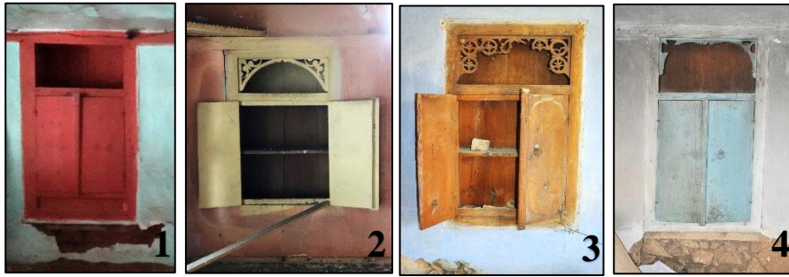
Figure 3.222. Examples of cupboard located on stone masonry wall (1-2, Kubbeli N. b. block-lot: 186-36; 3-4, Cumhuriyet N. b. block-lot: 433-3)
