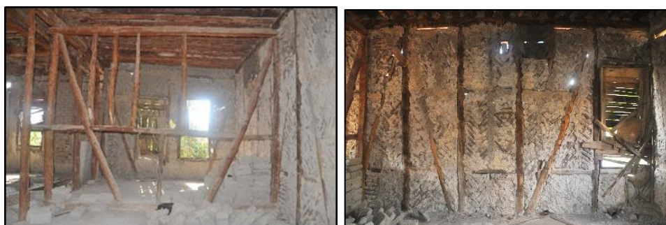
Figure 3.27. Connection detail of main braces with timber post, wall plate, and foot plate (Cumhuriyet N. b.block-lot: 433-2)
