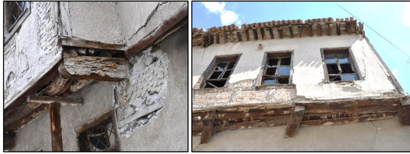
Figure 3.124. Examples of projection supported with a beam; simple projection, Type1 (Camikebir N. b.block-lot: 196-1)
