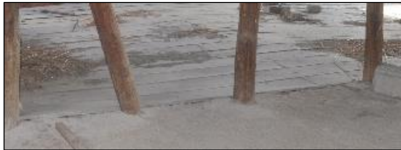
Figure 3.68. View of timber floor boards of flooring of Type 2 used in the sofa and earth infill of flooring seen in the room (Cumhuriyet N. b.block-lot:433-2)
