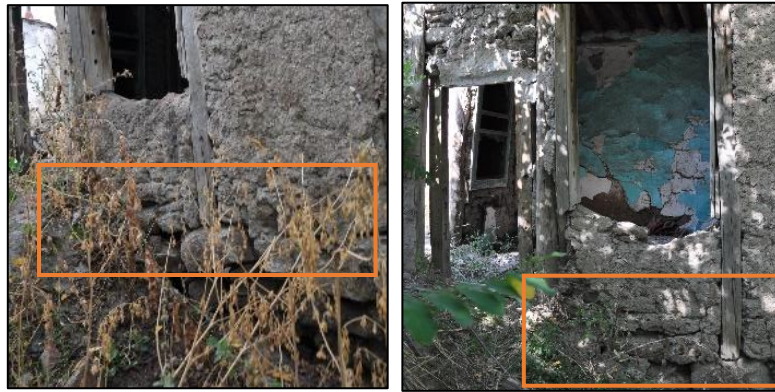
Figure 3.7. Timber framed wall located on stone masonry foundation wall without a timber foot plate (Gedik N. b.block-lot:362-19)
