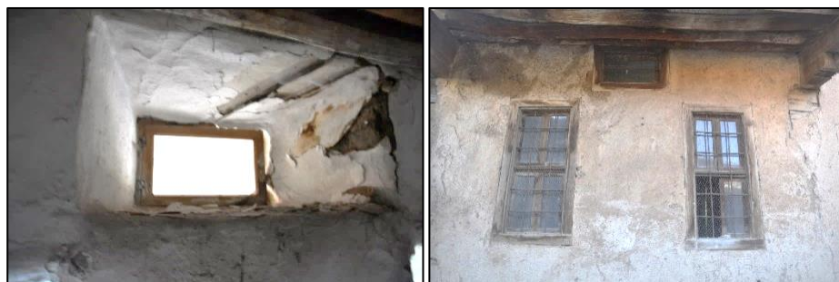
Figure 3.175. Top window opening located in the middle and above two windows on stone masonry wall; Type 4 (Cumhuriyet N. b. block-lot: 433-2)
