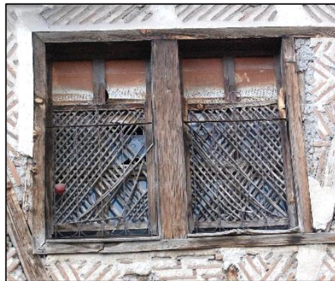
Figure 3.191. Timber lattices and iron railings located in front of the window opening (Demirci N. b. block-lot: 448-2)
