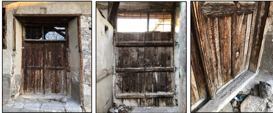
Figure 3.151. Exterior double wing framed batten door with top window located on stone masonry wall, Type 3; exterior facade (left), interior facade (middle), exterior façade detail (right) (Camikebir N. b. block-lot: 196-1)
