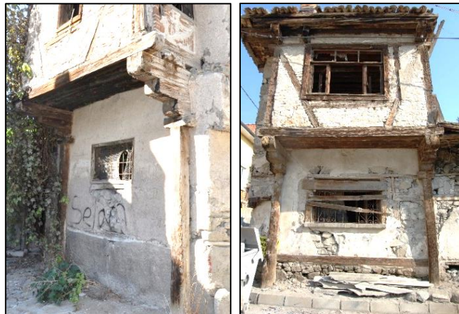
Figure 3.127. Examples of projections with overlapped beams and post; Type2 (left, Cumhuriyet N. b. block-lot: 433-3; right, Karabaşlı N. b. block-lot: 367-13)
