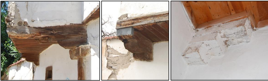
Figure 3.126. Example of projection supported overlapped beams, Type2; exterior view (left, middle), interior view of overlapped beams (right) (Yenice N. b. block-lot: 11-16)
