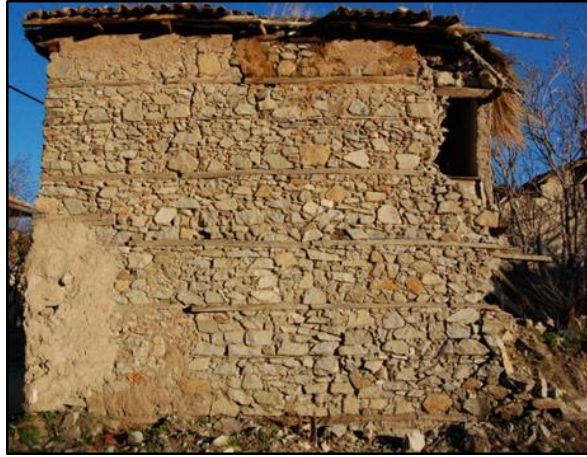
Figure 3.14. Stone masonry wall with timber lintel continue along the building height (Gedik N. b.blok-lot: 354-9)
