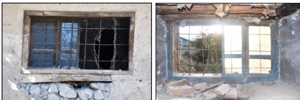
Figure 3.172. Window opening located on stone masonry wall; Type 3 (Cumhuriyet N. b. block-lot: 433-3)
