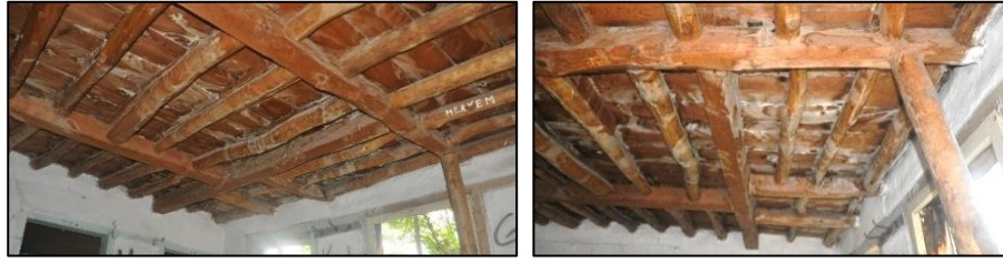
Figure 3.61. Simple timber flooring (Type 1) used in the sofa on the first floor (Cumhuriyet N. b.block-lot:433-2)
