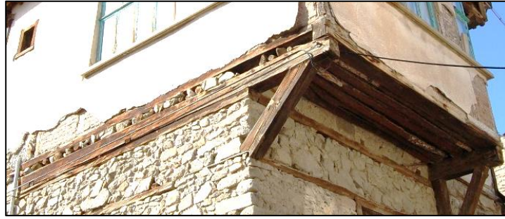
Figure 3.107. Connection detail 2, view of timber floor beams located on the wall plate of masonry wall in lower floor and foot plate located on the floor beams, extending wall plate and foot plate to form projection (Demirci N. Demirci St. N:12 b.block-lot: 443-4)
