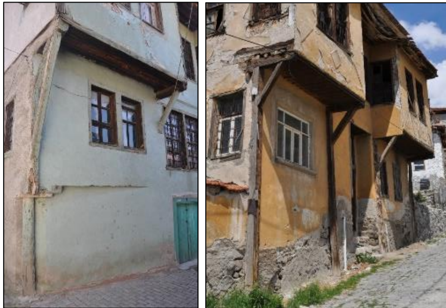
Figure 3.129. Examples of projections with timber brace, Type3 (left, Demirci N. b.block-lot: 443-13; right, Kılıç N. b.block-lot: 170-19)
