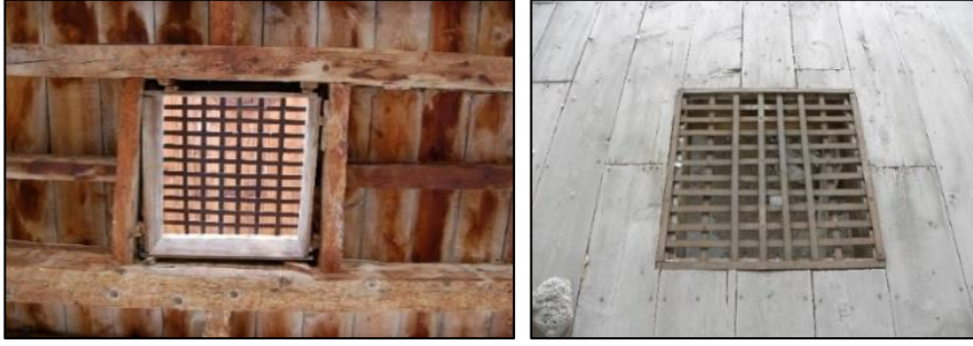
Figure 3.197. Example of simple timber flooring (Type 1) with peep hole (left, Yenice N. b. block-lot: 521-7-8 ; right, Yenice N. b.block-lot:521-12)
