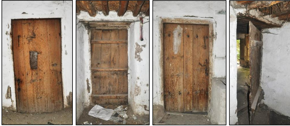
Figure 3.144. Examples of interior single wing batten doors located on stone masonry wall used in the service spaces; Type 1 (Cumhuriyet N. b. block-lot: 433-2)
