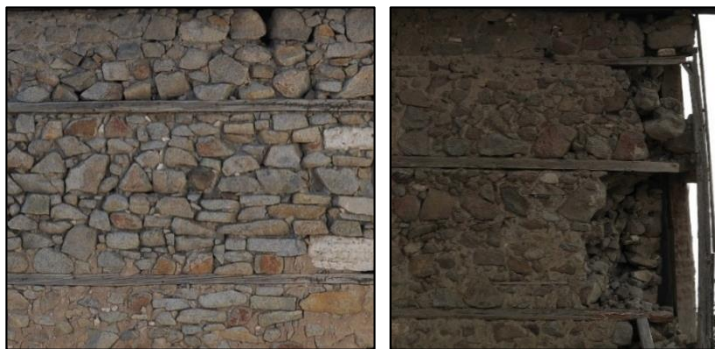
Figure 3.16. Examples of un-coursed rubble stone masonry walls (left, Camikebir N. b.blok-lot:188-4; right, Elmalı N. b.block-lot: 229-6)
