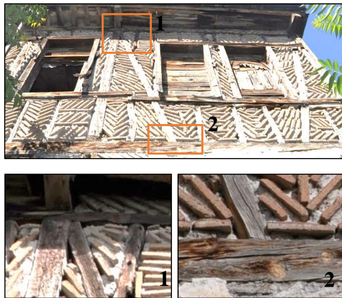
Figure 3.29. Connection detail of main braces with timber post, wall plate and foot plate (Cumhuriyet N. b.block-lot: 433-2)
