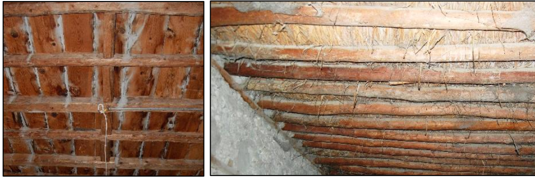
Figure 3.199. Timber ceiling that is not covered in hall, timber floor beams and timber floor boards (left, Type 1A) and timber ceiling that is not covered in kitchen in ground floor, timber floor beams and reed infill (right, Type 1B) (left, Yenice N. b. block-lot: 521-7-8; right, Camikebir N. b. block-lot: 188-4)
