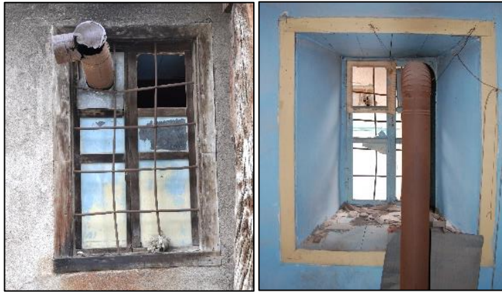
Figure 3.166. Window opening located on stone masonry wall; Type 1 (Camikebir N. b. block-lot: 196-1)
