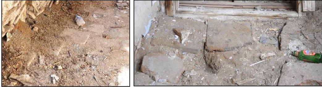
Figure 3.198. View of terracotta floor covering used in the sofa (Kılıç N. b.block-lot:170-44)
