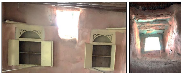
Figure 3.177. Top window opening located in the middle and above the two cupboards on stone masonry wall; Type 4 (Kubbeli N. b. block-lot: 186-36)
