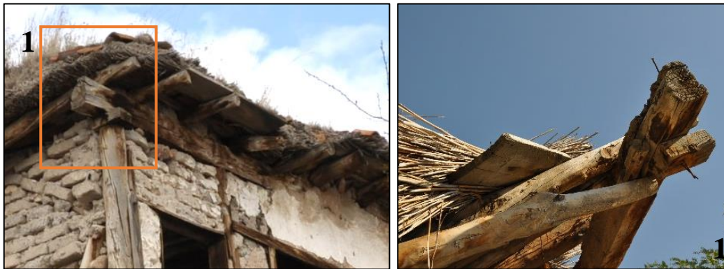
Figure 3.119. Connection detail 6, timber floor beams located on the wall plate of upper floor wall (left), connection of timber floor beam and wall plate (right) (Gedik N. b.block-lot:362-19)
