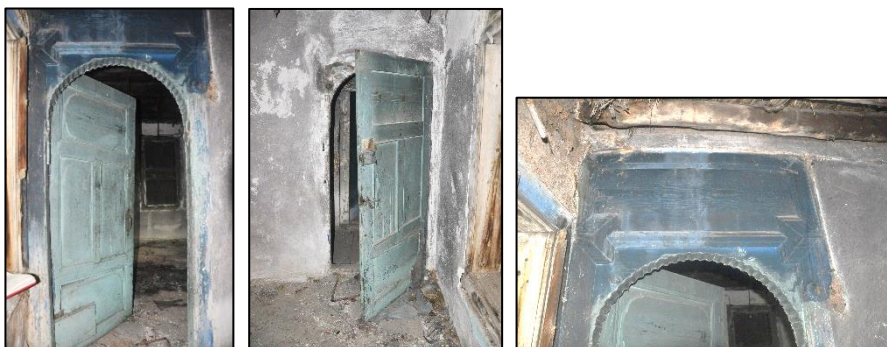
Figure 3.155. Example of interior single wing panel door with arched door frame located on timber framed wall, Type 4; exterior view (left), interior view (middle), detail from exterior view (right) (Cumhuriyet N. b. block-lot: 433-3)
