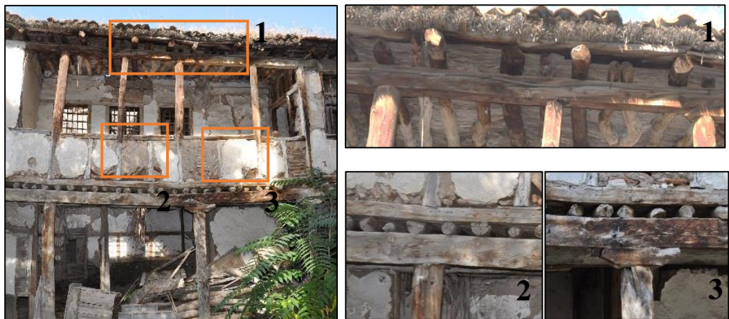
Figure 3.47. Timber posts with connection detail Type 1 and detail Type 2 used on ground and upper floor (Kubbeli N. b.block-lot: 170-44)
