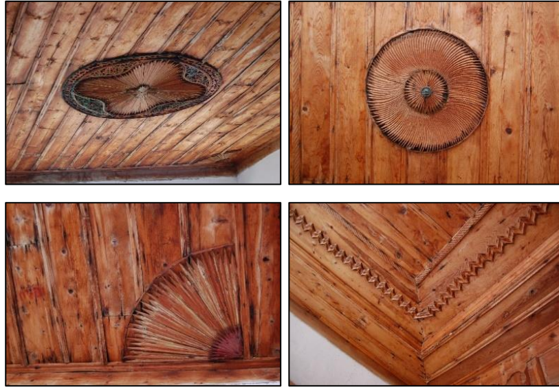
Figure 3.204. Timber ceiling covered with timber boards and timber laths, decorated with göbek and ornamentals; Type 2C (Yenice N. b. block-lot: 521-12)
