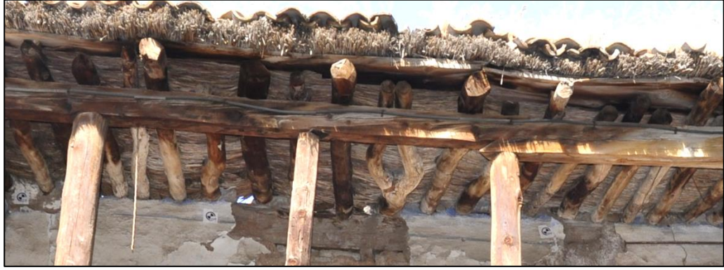
Figure 3.120. Connection detail 6, timber floor beams located on the wall plate of upper floor timber posts (Kılıç N. b.block-lot: 170-44)
