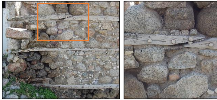
Figure 3.20. Timber lintels on the façade of stone masonry wall (left), connection of two pieces of timber lintel (right) (Camikebir N. b.block-lot: 198-11)
