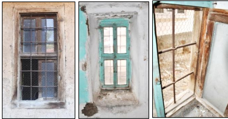
Figure 3.170. Window opening located on stone masonry wall; Type 2 (Cumhuriyet N. b. block-lot: 433-2)
