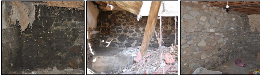
Figure 3.3. Ongoing foundation walls in the basement floor (left, Kubbeli N. b.block-lot: 186-40; middle, Camikebir N. b.block-lot: 198-11; right, Kılıç N. b.block-lot: 170-19)
