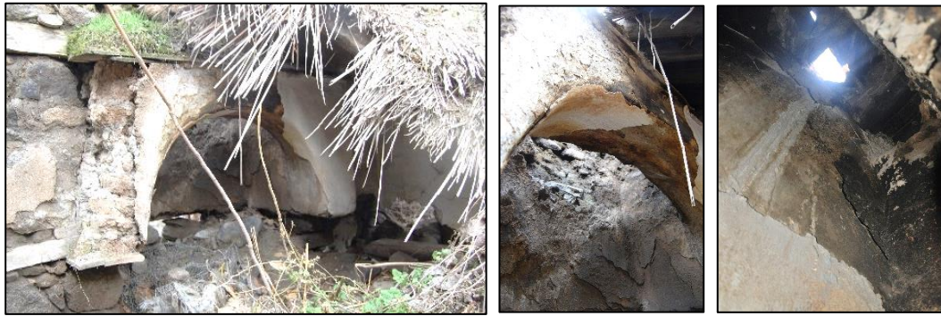
Figure 3.212. Details of fireplace; projected front face of fireplace made of brick and covered with mud plaster (left); arched opening of fireplace (middle); chimney shaft of fireplace (right) (Camikebir N. b. block-lot: 186-10)
