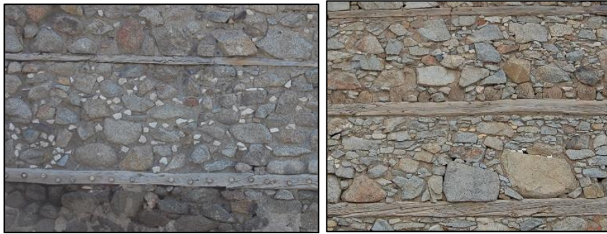
Figure 3.15. Examples of un-coursed rubble stone masonry walls (left, Camikebir N. b.blok-lot:198-11; right, Yenice N. b.block-lot: 12-29)
