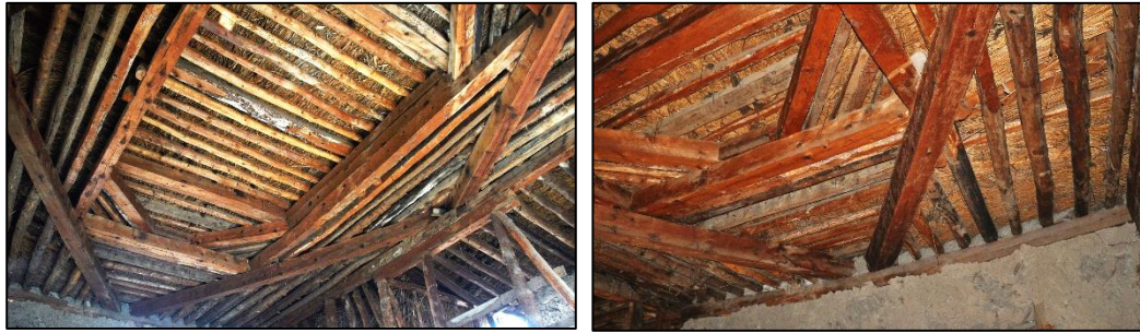
Figure 3.205. Timber ceiling constructed with overlapped beams; detail of ceiling without timber covering boards that are lost; Type 2D (Cumhuriyet N. b. block-lot: 433-2)
