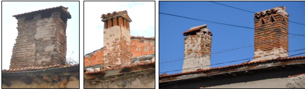
Figure 3.91. Examples of fireplace chimneys in main building (left, Demirci N. b.block-lot:443-13; middle, Yenice N. b.block-lot: 12-29; right, Yenice N. b.block-lot:12-20)
