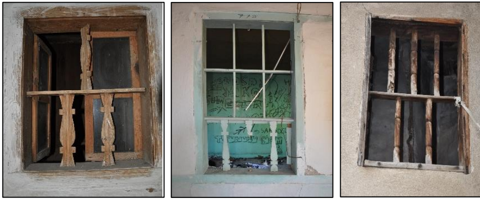
Figure 3.190. Examples of timber railings (left, middle, Cumhuriyet N. b. block-lot: 433-2; right, Camikebir N. b. block-lot: 196-1)
