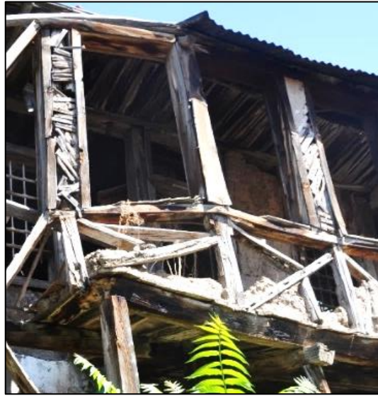
Figure 3.42. Type 1 – timber posts covered with timber laths and single timber board used on the façade of semi open sofa (Kubbeli N. b.block-lot: 186-9)
