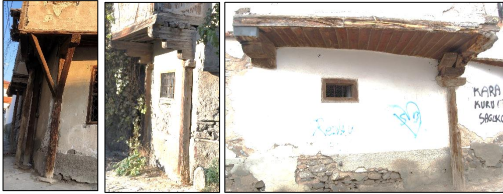
Figure 3.38. Timber posts used in the street façade under the projection (left, Camikebir N. b.block-lot:196-1; middle, Cumhuriyet N. b.block-lot: 433-3; right, Yenice N. b.block-lot: 11-16)
