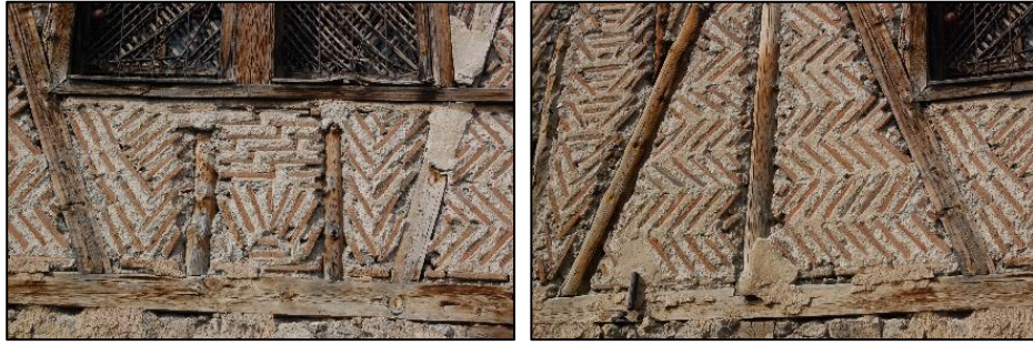
Figure 3.28. Connection detail of main braces and timber post with foot plate (Demirci N. b.block-lot: 448-2)
