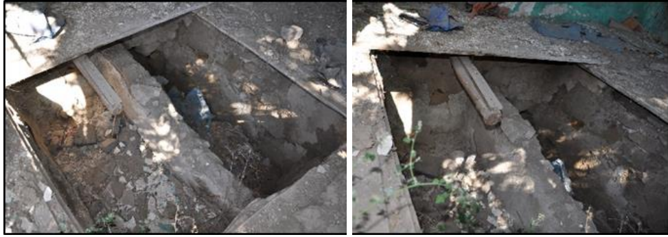
Figure 3.9. Continuous foundation with gradually decreasing width at one level at one side (Gedik N. b.blok-lot: 362-19)
