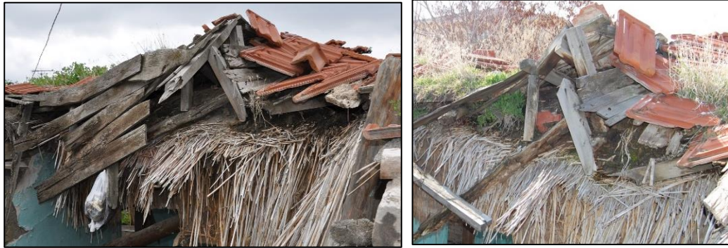
Figure 3.79. Timber roof ridge, king post and timber roof boards of timber roof structure located on earth infill of flooring (Camikebir N. b.block-lot: 198-11)
