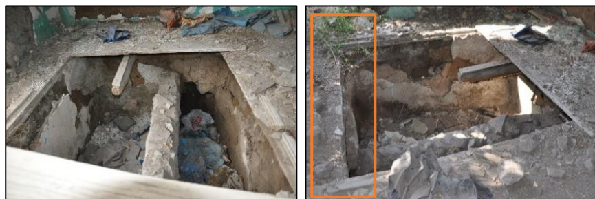
Figure 3.51. Simple timber flooring in the room of ground floor, view of enlarged stone masonry wall and wall plate of stone masonry foundation wall (Gedik N. b.block-lot:362-19)
