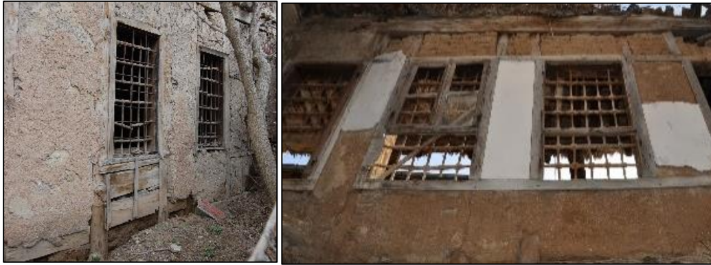
Figure 3.34. Timber framed wall with mud brick infill covered with mud plaster (left), covered with mud plaster and whitewashed (right) (left, Elmalı N. b.block-lot: 229-6; right, Kılıç N. b.block-lot:170-44)
