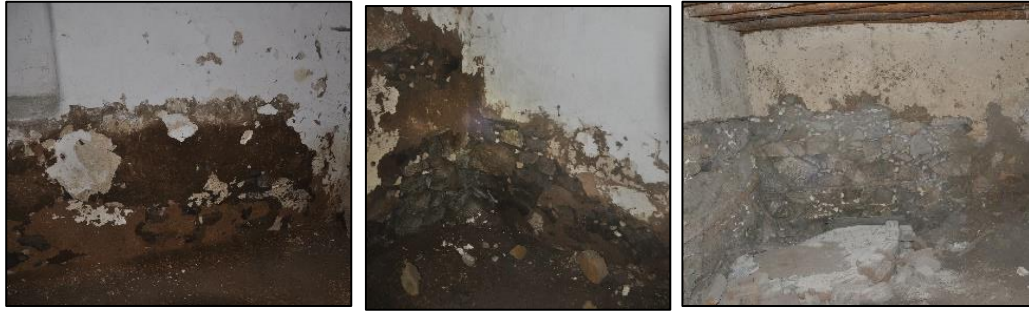
Figure 3.23. Stone masonry wall covered with mud plaster and whitewashed (Cumhuriyet N. b.block-lot: 433-2)
