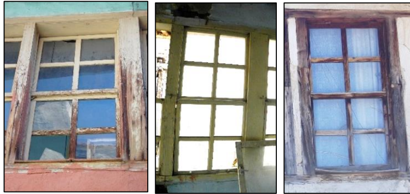
Figure 3.186. Examples of sash windows located on sofa (left, middle, Kubbeli N. b. block-lot: 186-36; right, Demirci N. b. block-lot: 444-15)
