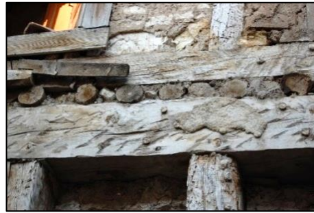
Figure 3.110. Connection detail 3, View of timber floor beams located on the wall plate of lower timber framed wall and foot plate of upper floor wall located on the floor beams (Karabaşlı N. b.block-lot: 367-13)
