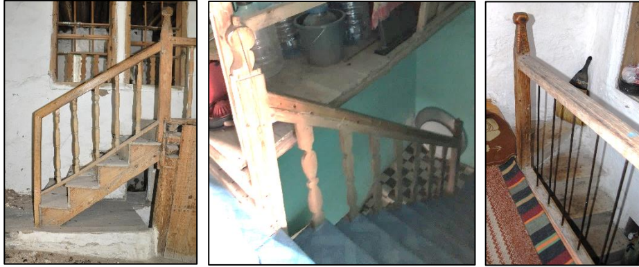
Figure 3.142. Handrail and baluster examples (left, Cumhuriyet N. b. block-lot: 433-2; middle, Yenice N. b. block-lot: 521-8; right, Demirci N. b. block-lot: 444-15)
