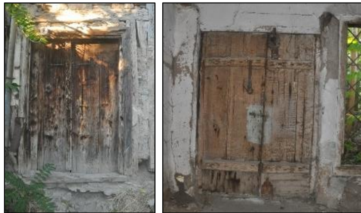
Figure 3.160. Exterior double wing batten door located on timber framed wall, Type 5; exterior façade (left), interior façade (right) (Cumhuriyet N. b. block-lot: 433-2)
