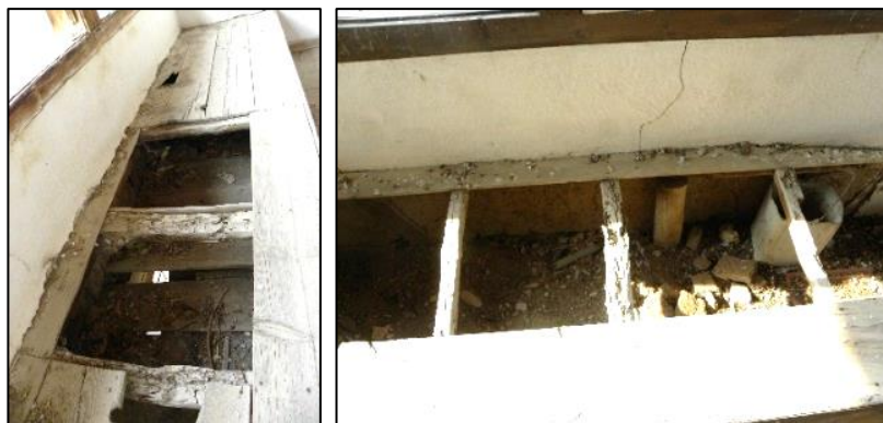
Figure 3.229. Example of I shape sedir ; detail of sedir (Yenice N. b. block-lot: 521-12)
