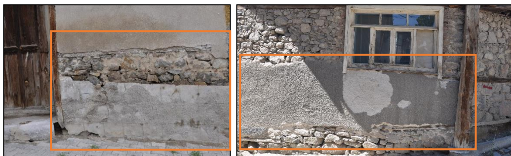
Figure 1.2. Stone wall surfaces covered with cement based plastered (left, Camikebir N. b.block-lot: 196-1; right, Kubbeli N. b.block-lot: 186-9)
