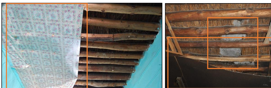
Figure 1.3. Ceiling covered with linoleum (left), ceiling covered with plywood and screed applied to the flooring seen from ceiling (right) (left, Demirci N. b.block-lot: 443-13; right, Cumhuriyet N. b.block-lot: 433-3)
