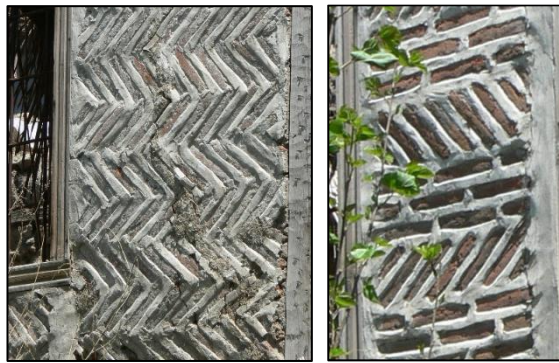
Figure 3.32. Timber framed wall with herringbone brick composition (left) and alternate use of brick in horizontal and diagonal order (right) (Kubbeli N. b.block-lot: 186-40)
