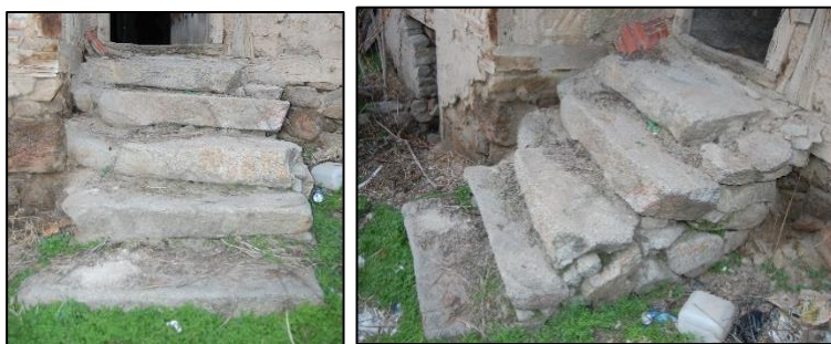
Figure 3.133. Stone stair used at the courtyard entrance; Type1 (Demirci N. b. block-lot: 448-2)
