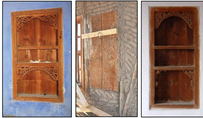
Figure 3.218. Niche located on the timber framed wall, Type 2A; (left, middle, Kılıç N. b. block-lot: 170-19; right, Yenice N. b. block-lot: 521-12)
