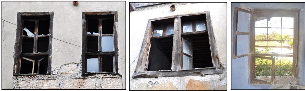
Figure 3.179. Window opening located on timber framed wall; Type 5, Casement windows, (left, middle, Camikebir N. b. block-lot: 196-1; right, Cumhuriyet N. 4 b. block-lot: 433-3)
