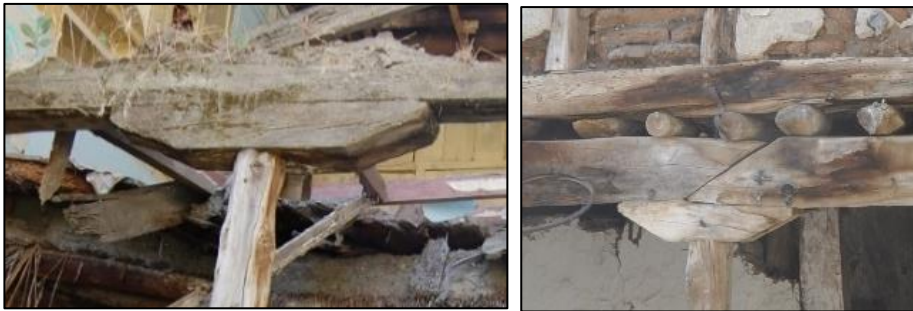
Figure 3.43. Type 2 - timber post with bolster on top (left, Kubbeli N. b.block-lot: 186-36; right, Kubbeli N. b.block-lot: 170-44)
