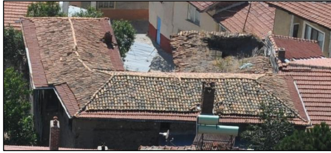
Figure 3.82. Hipped roof and collapsed one side sloping roof (Kılıç N. b.block-lot: 170-44)
