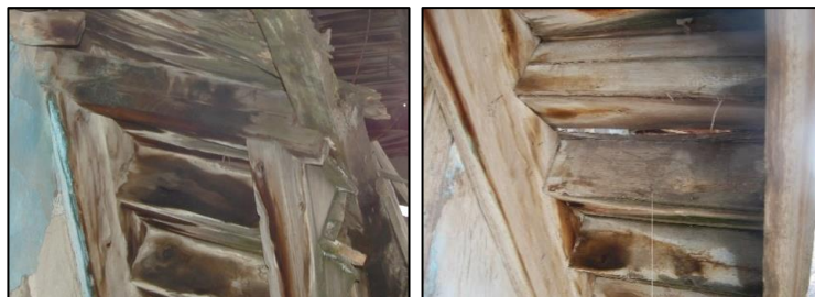
Figure 3.137. Upper connection detail of stringer (left), timber step boards are located on stringers (right)-Type2A (Kubbeli N. b. block-lot: 186-9)
