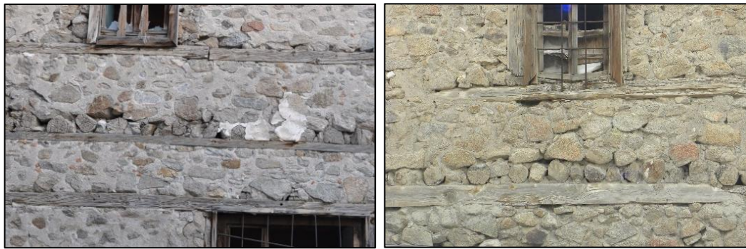
Figure 3.94. Connection detail 1, view of floor beams inserted into wall along the wall thickness (left, Karabaşlı N. b. block-lot: 367-13; right, Kubbeli N. b. block-lot: 186-40)
