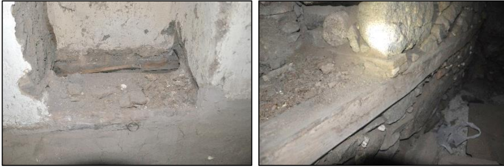
Figure 3.217. Timber lintels and tie beam located at bottom level of niche Type 1A (Cumhuriyet N. b. block-lot: 433-2)
