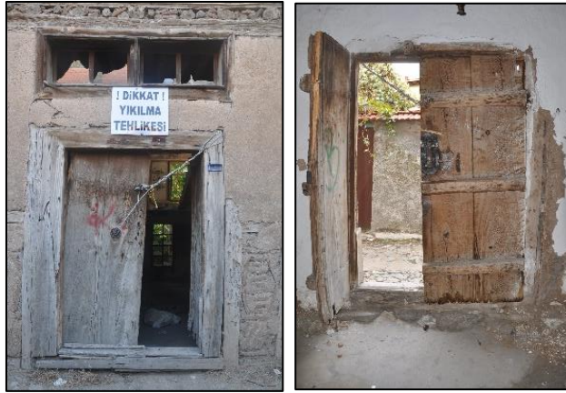
Figure 3.163. Exterior double wing batten door with top window located on timber framed wall, Type 6; exterior façade (left), interior façade (right) (Cumhuriyet N. b. block-lot: 433-2)
