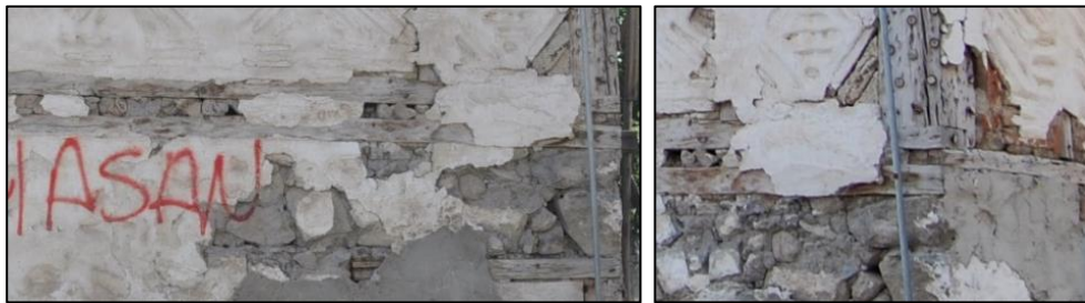
Figure 3.98. Connection detail 2, view of timber floor beams located on the wall plate of masonry wall in lower floor and foot plate located on the floor beams, corner post located on the foot plate (Kılıç N. b.block-lot:161-1)
