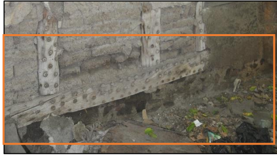
Figure 3.6. Timber beam as a foot plate of timber framed wall located on stone masonry foundation wall (Cumhuriyet N. b.block-lot:433-3)
