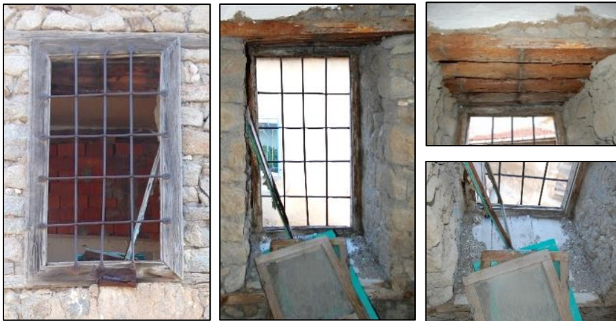
Figure 3.167. Window opening located on stone masonry wall; Type 1 (Camikebir N. b. block-lot: 188-4)
