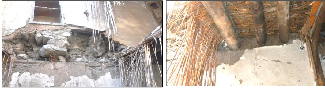
Figure 3.93. Connection detail 1, view of floor beams inserted into wall along the wall thickness (Kılıç N. b.block-lot: 170-44)
