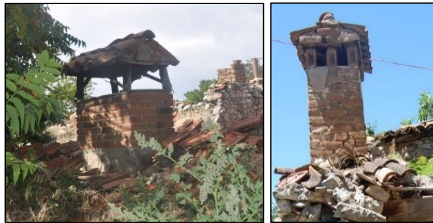
Figure 3.92. Examples of fireplace chimneys made of brick masonry in tandır evi (left, Cumhuriyet N. b.block-lot: 433-2; right, Yenice N. b.block-lot: 11-16)
