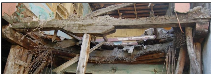
Figure 3.64. Timber flooring (Type 2) used in the room in first floor (Kubbeli N. b.block-lot:186-36)
