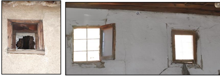
Figure 3.182. Top window opening on timber framed wall; Type 6 (Camikebir N. b. block-lot: 196-1; Kılıç N. b. block-lot: 170-44)
