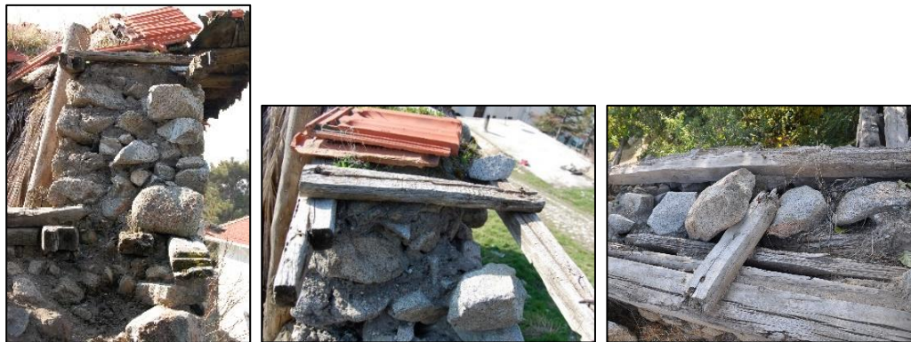
Figure 3.21. Timber lintels and tie beams of stone masonry wall (left, middle,Camikebir N. Acem St. N:4/1 b.block-lot: 198-11; right, Gedik N. Esen St.N:22 b.block-lot: 362-19)
