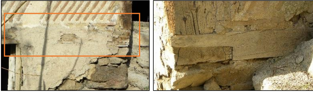
Figure 3.105. Connection detail 2, connection of timber foot plates by half lap joints and nails, (Demirci N. b.block-lot:448-2)
