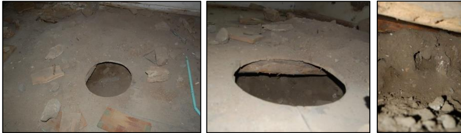
Figure 3.49. General view of simple timber flooring in the room of ground floor (left), timber floor boards and timber floor beam seen through the drilled hole (middle), air gap between timber floor beam and pressed earth (right) (Yenice N. b.block-lot:11-16)
