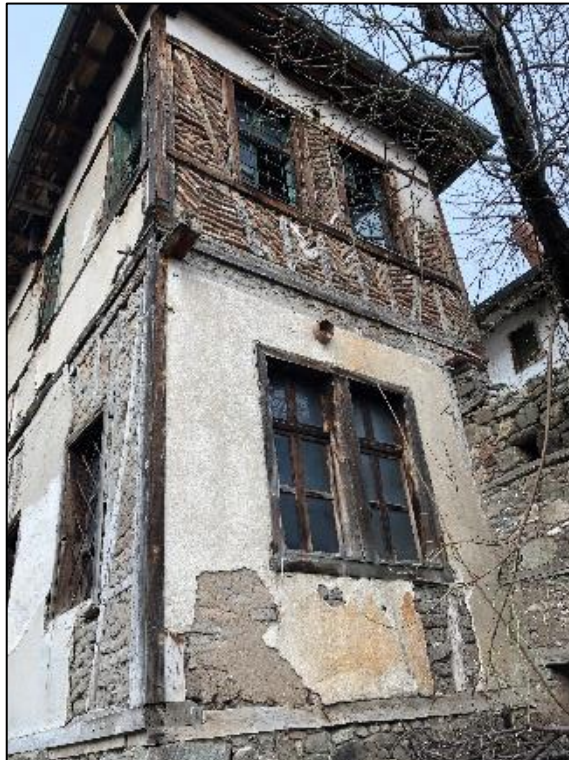
Figure 3.35. Timber framed wall covered with mud plaster and whitewashed (walls with mudbrick infill at lower floor, with brick infill at upper floor) (Kılıç N. b.block-lot:170-44)
