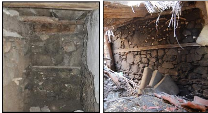
Figure 3.4. Ongoing foundation walls with timber lintel in the basement floor (left, Cumhuriyet N. b.block-lot: 433-2; right, Camikebir N. b.block-lot: 198-11)
