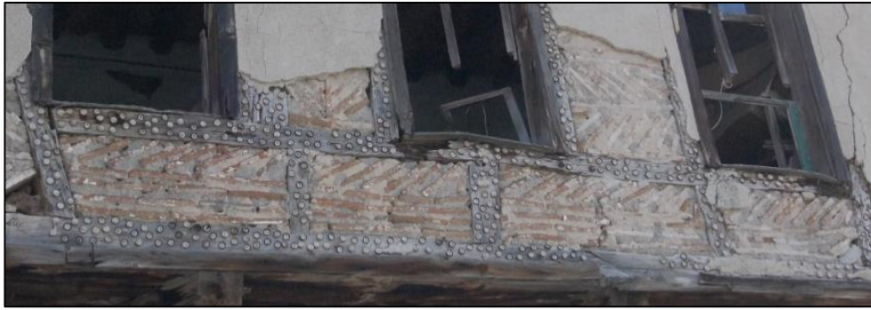
Figure 3.37. Timber framed wall with brick infill covered with mud plaster and crown caps nailed to timber elements of frame system (Camikebir N. b.block-lot: 196-1)
