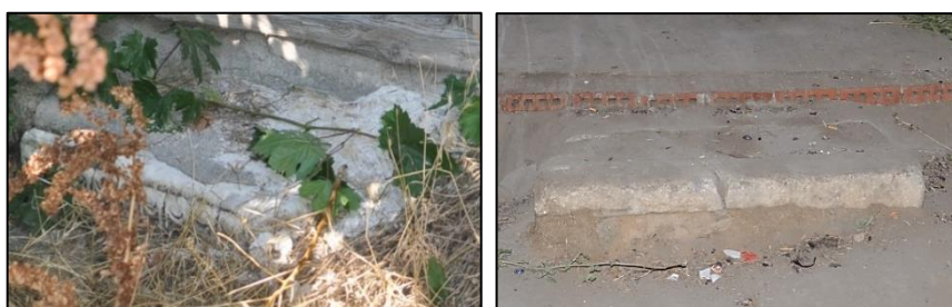
Figure 3.135. A reused stone step used at the courtyard entrance (left) and in taşlık (right) (Cumhuriyet N. b. block-lot: 433-2)
