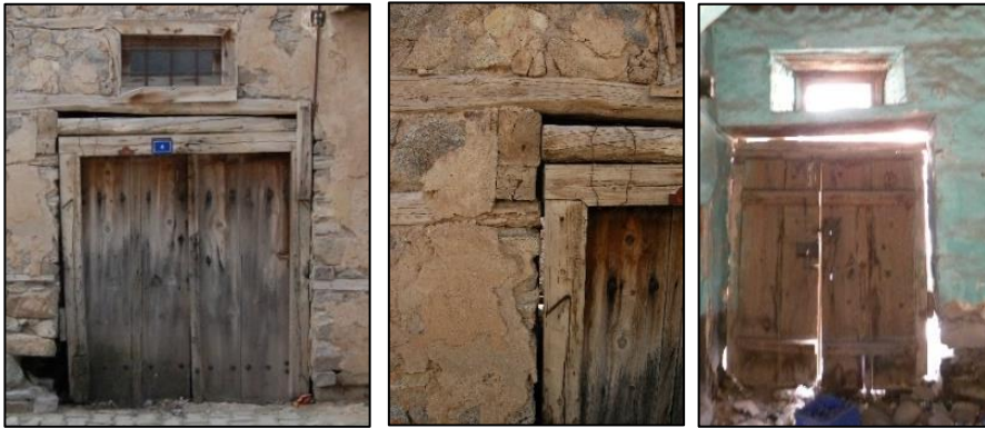
Figure 3.149. Exterior double wing batten door with top window located on stone masonry wall, Type 3; exterior façade (left), door post&door sill detail from exterior (middle), interior facade (right) (Demirci N. b.block-lot: 448-2)
