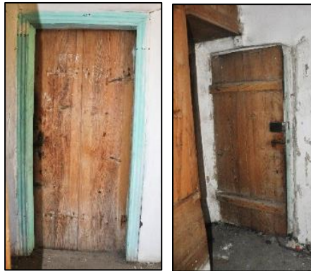
Figure 3.154. Example of interior single wing batten door located on timber framed wall, Type 4; exterior view (left), interior view (right) (Cumhuriyet N. b. block-lot: 433-2)
