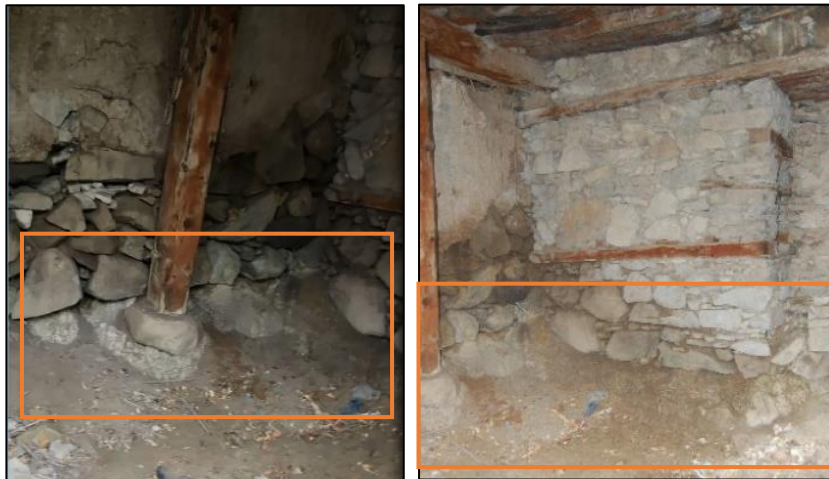
Figure 3.11. Rock as a part of foundation under the masonry wall and stone base (left) and stone masonry wall of ground floor (right) (Yenice N. b.blok-lot: 12-30)
