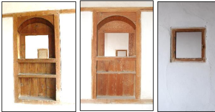
Figure 3.221. Niches with window located on the timber framed wall (Yenice N. b block-lot: 521-12)
