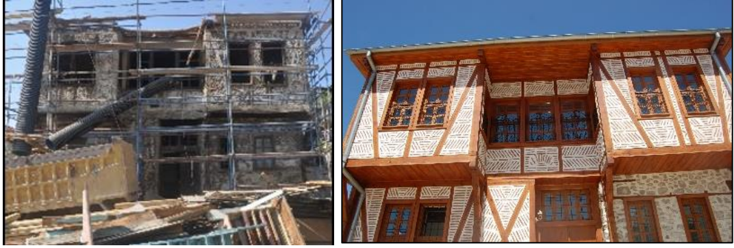
Figure 1.4. A traditional house at Hisar Street during (left) and after (right) the restoration application (Kılıç N. b.block-lot: 170-19)
