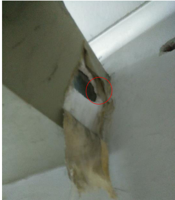
Figure 4.11. Selected area for risk assessment in Building-D [red circle shows the sampling location]
