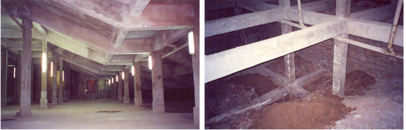
Figure 5. The most vulnerable part of Anıtkabir in terms of structural safety is the staircases.
