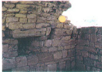
H5. Mescid Space, Interior of the East Wall and the Vault ( ● kurm.SM1)
