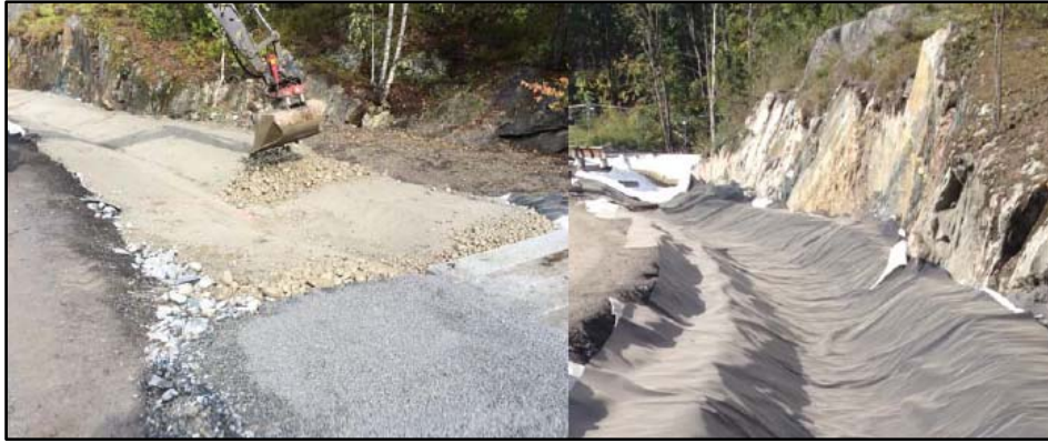
Figure 3.13. Construction of streambed for providing infiltration function, Julsberg Stream Project. [Source: Rapp, O. (2019)]
