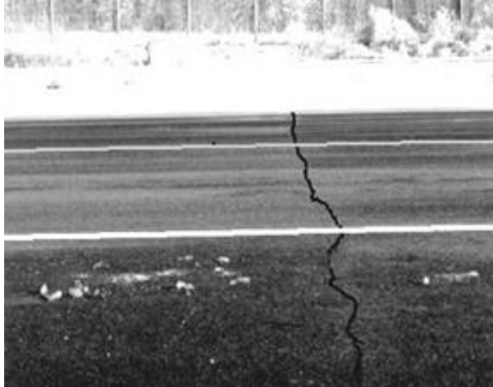
Figure 2.3. Example of low temperature cracking in asphalt concrete pavement (Minnesota department of transportation)
