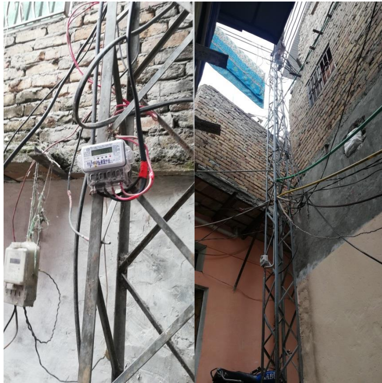
Figure 5.12: Precarious wires hanging from the main connection showing the extra wires added for temporal supply
