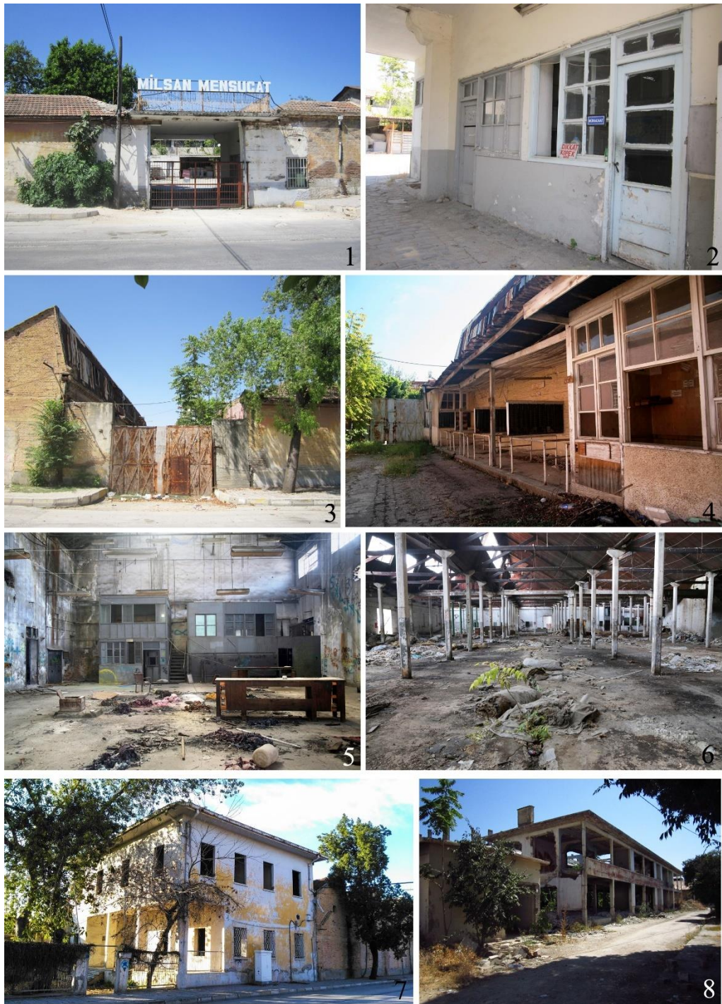
Figure 4.70. Obsolescent parts of Milli Mensucat Fabrikası [The National Textile Factory] 2018, (1) and (2) Officers' entry, (3) and (4) Workers' entry, (5) Clubhouse, (6) Single lodgings (Source: author's personal archive)
