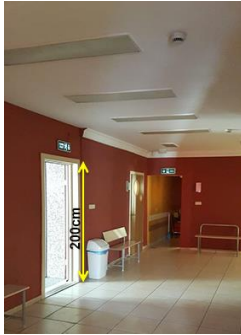
Figure 31: Removed fire door leaf and location.
