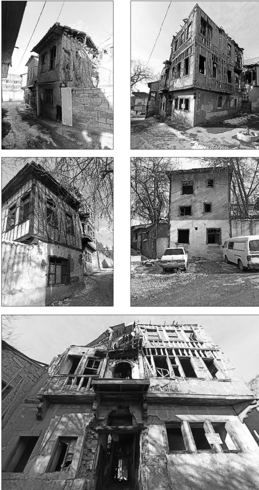
Figure 4.23. Abandoned buildings of Jewish Quarter in poor physical condition (Source: various personal field observations from December 2020 to June 2021)
