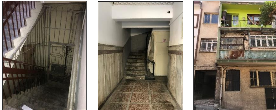
Figure 38, 39, 40, and 41: Interior and Exterior Structural Condition of the Buildings in Area B
