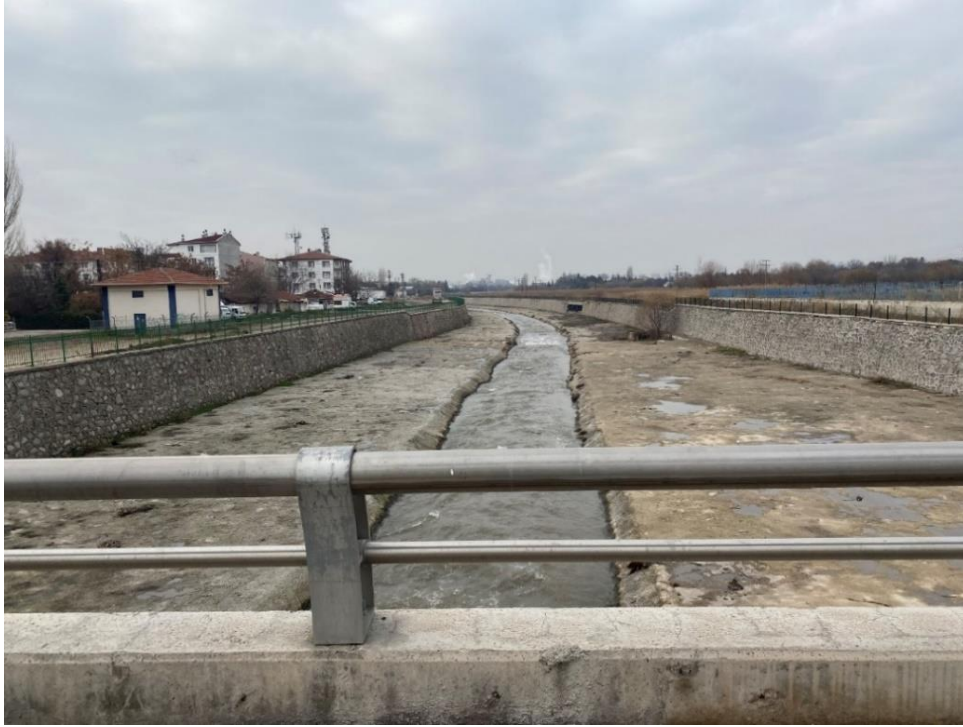
Figure 5.16. Ankara stream near the Etiler Street towards the Sugar Factory. Photo by the author, December, 2020.
