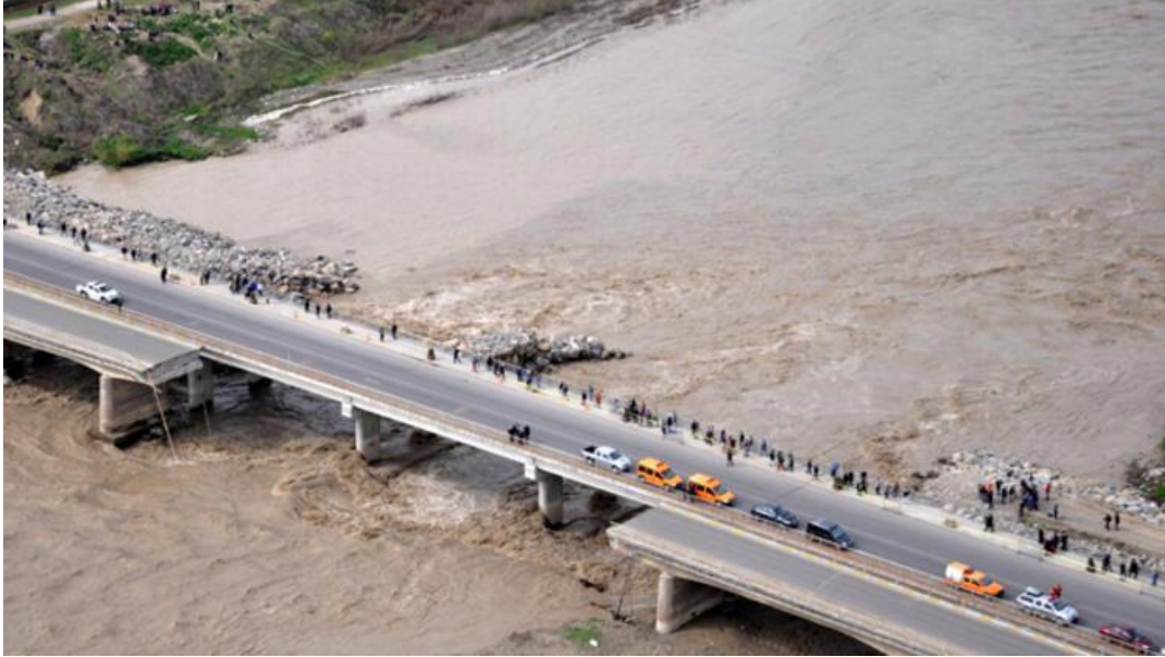
Figure 1.1 Çaycuma bridge after the collapse (Ercan & Gündoğan, 2015)
