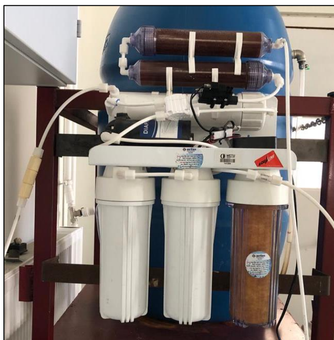
Figure 3.11. Deionized water system
