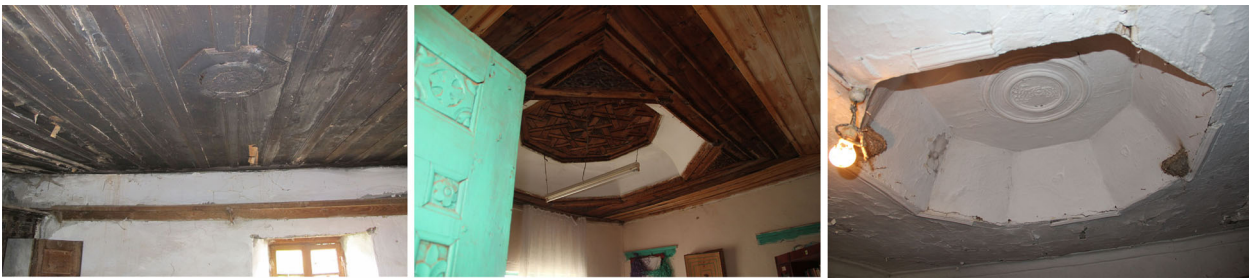
Figure 22. Protruding tavan göbeği (left), embedded tavan göbeği covered with wooden elements (middle) and embedded tavan göbeği covered with plaster and whitewash (right).
