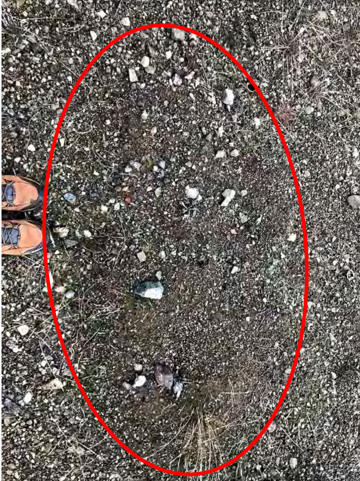
Figure 4.56. Seismic soil liquefaction-induced sand boils ( 38^{\circ}29'32.1''N 39^{\circ}21'02.0''E / 31.01.2020 / 16:58)
