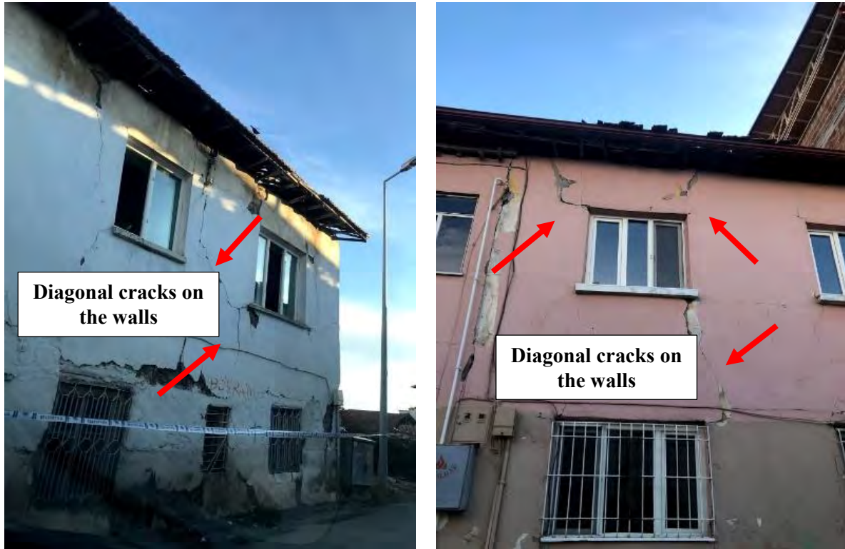
Figure 4.62. Cracks on the wall of a residential building in Battalgazi Village (38°25'21.7"N 38°21'56.9"E / 01.02.2020 / 8:30 & 38°25'24.4"N 38°21'53.6"E / 01.02.2020 / 8:28)
