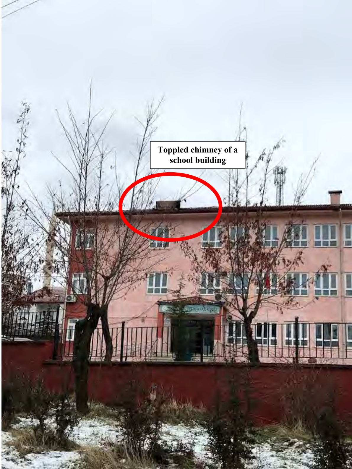
Figure 4.25. Topped chimney in Sivrice ( 38^{\circ}26'49.7''N 39^{\circ}18'33.0''E / 31.01.2020 / 13:30)
