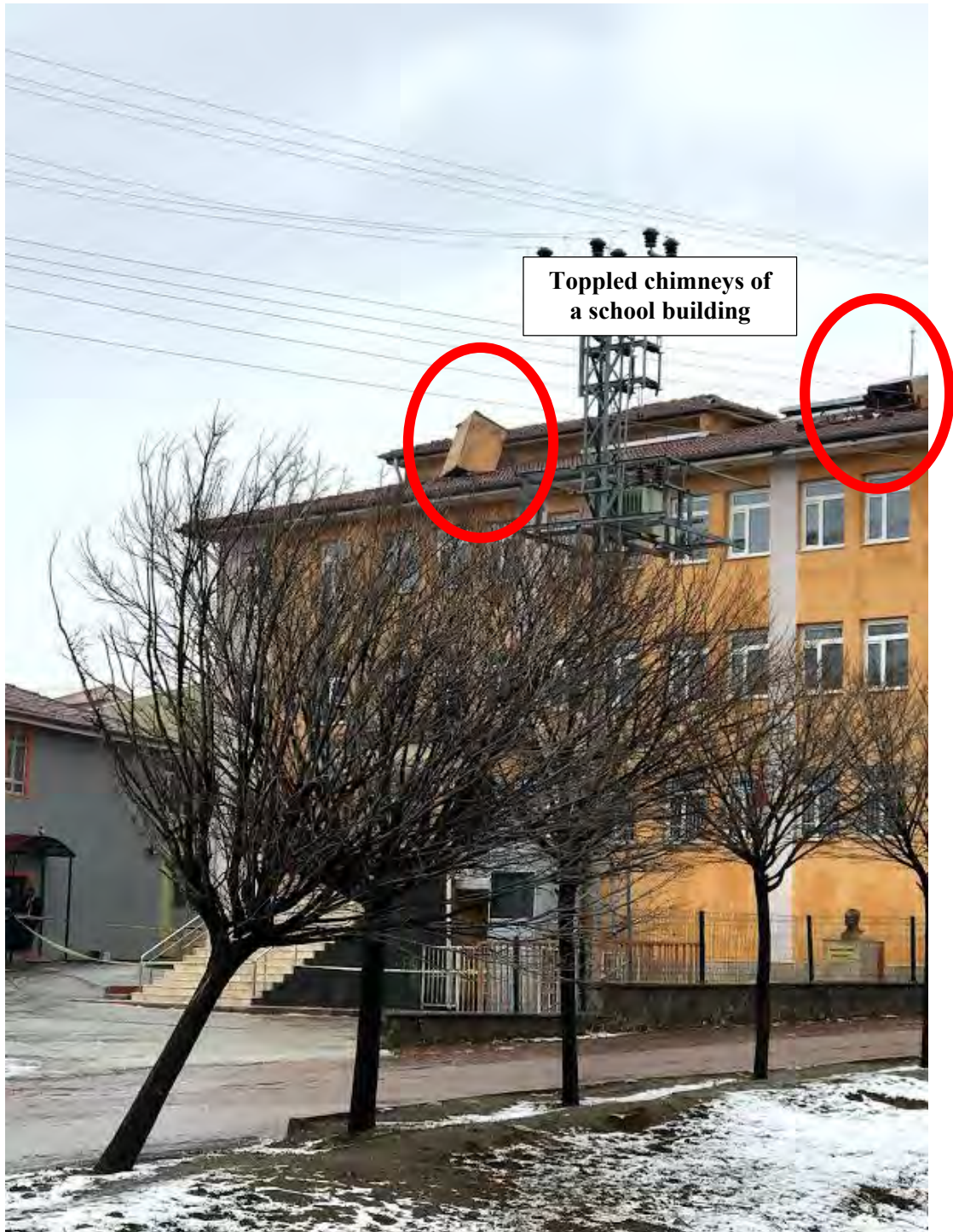
Figure 4.24. Toppled chimneys in Sivrice ( 38^{\circ}26'49.6''N 39^{\circ}18'32.9''E / 31.01.2020 / 13:29)
