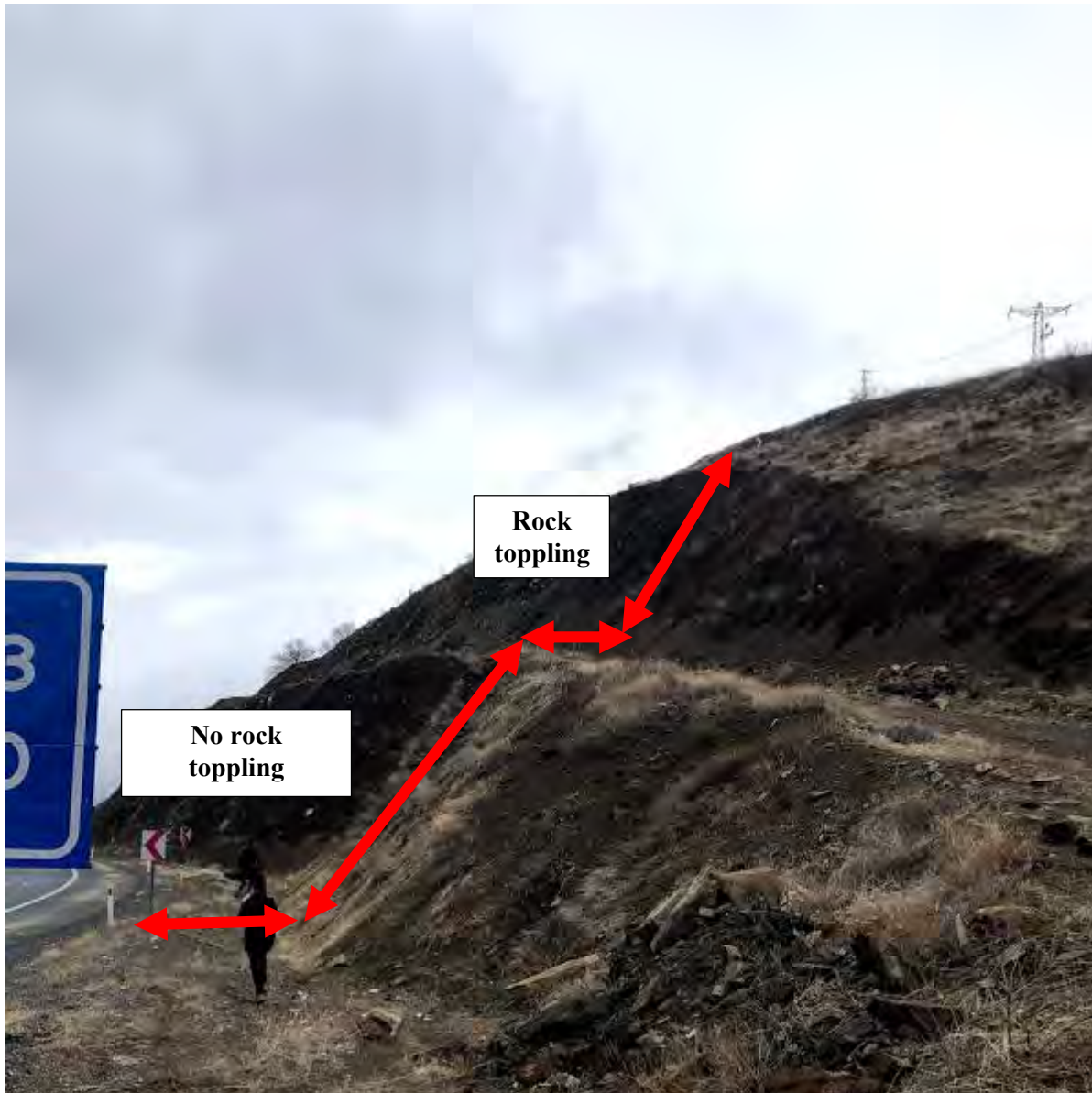
Figure 4.47. Rockfall at 13 th stop (general view) (38°31'40.3"N 39°28'02.9"E / 31.01.2020 / 16:20)
