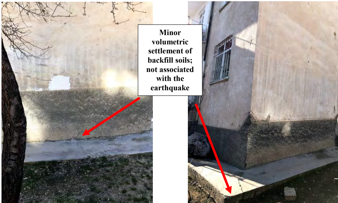
Figure 4.94. Volumetric settlement at the foundation of a residential building ( 38^{\circ}39'29.8''N 39^{\circ}08'58.4''E / 01.02.2020 / 14:29 & 38^{\circ}39'28.9''N 39^{\circ}09'01.9''E / 01.02.2020 / 14:30)
