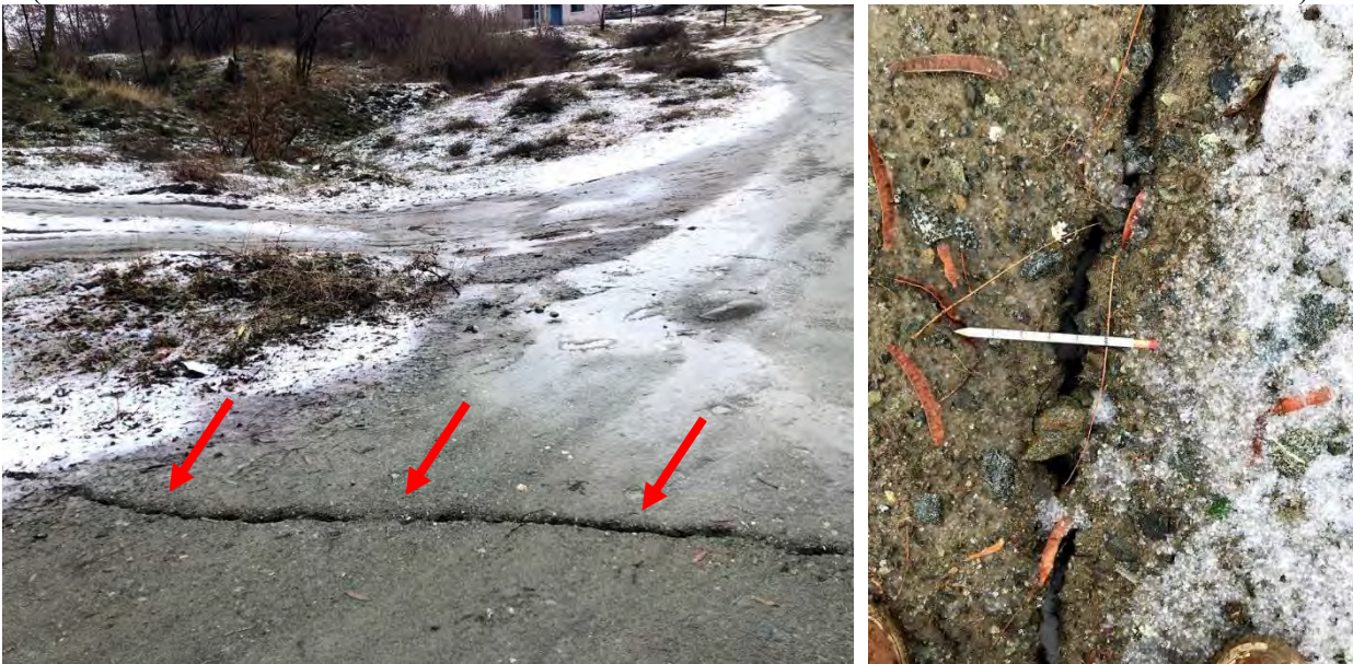
Figure 4.125. Deformations and cracks due to lateral spreading observed along Hazar Lake (2 nd stop)
