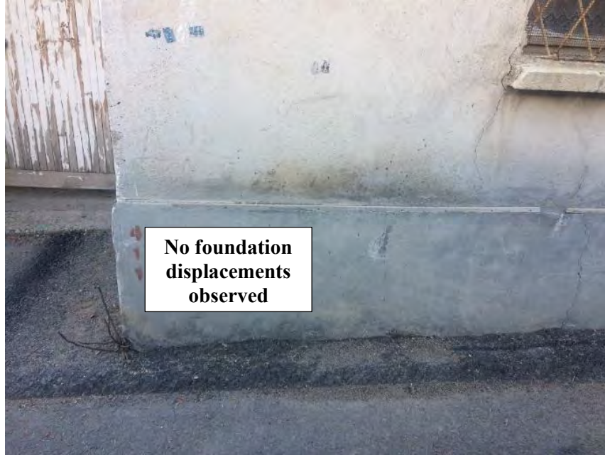
Figure 4.65. No foundation displacements observed at a residential building in Battalgazi Village ( 38^{\circ}25'20.7''N 38^{\circ}21'59.3''E / 01.02.2020 / 8:31)
