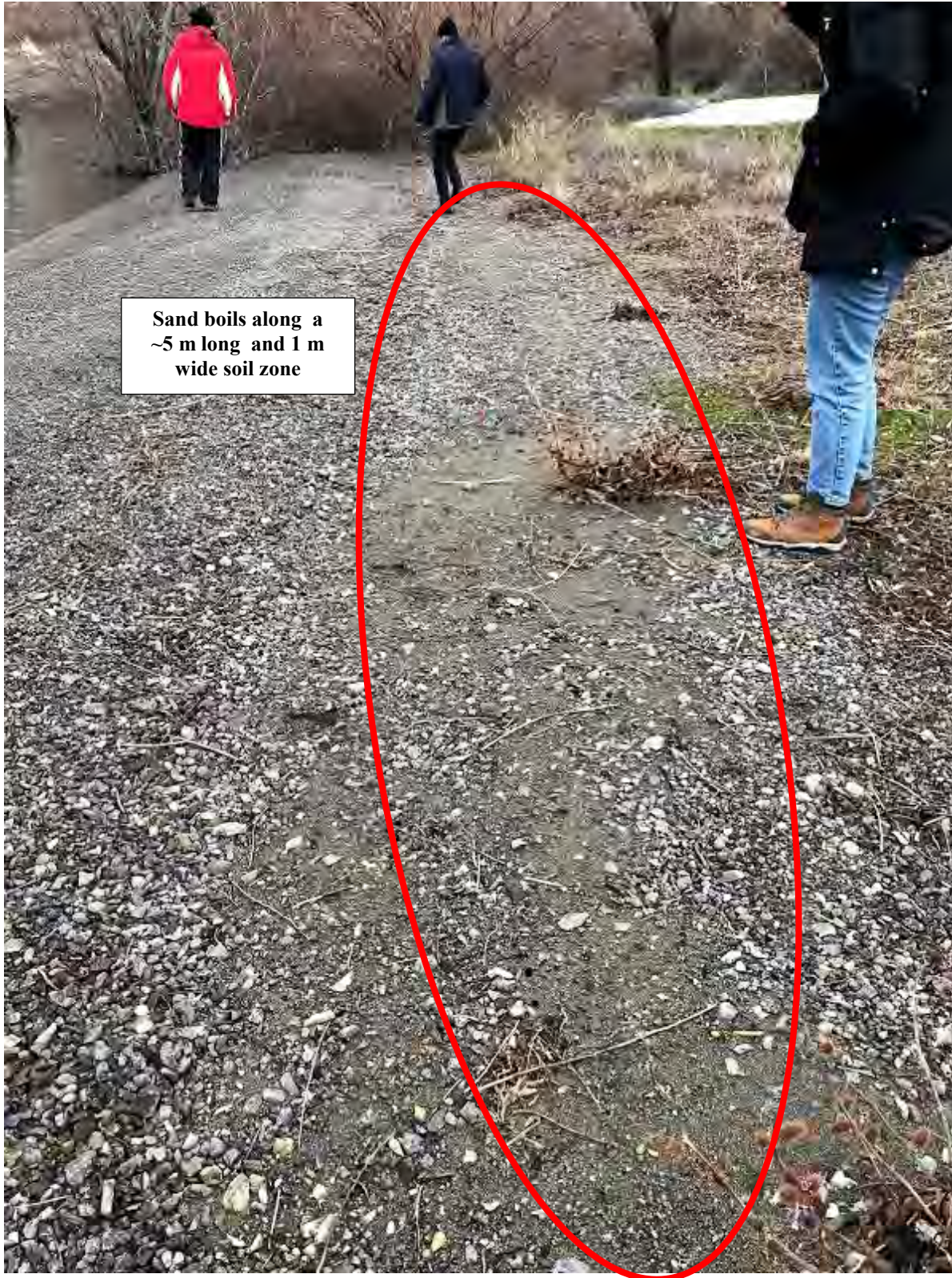
Figure 4.33. Sand boils observed in Stop 8 ( 38^{\circ}27'49.8''N 39^{\circ}24'03.0''E / 31.01.2020 / 14:14)
