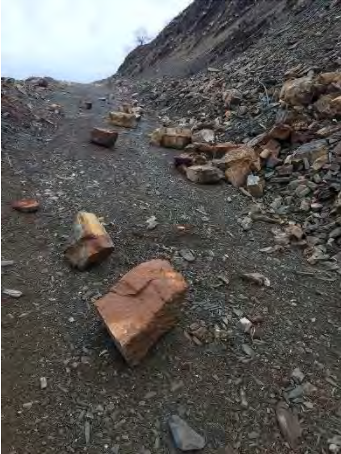
Figure 4.49. Rockfalls at 13 th stop (38°31'41.0"N 39°27'59.6"E / 31.01.2020 / 16:13)
