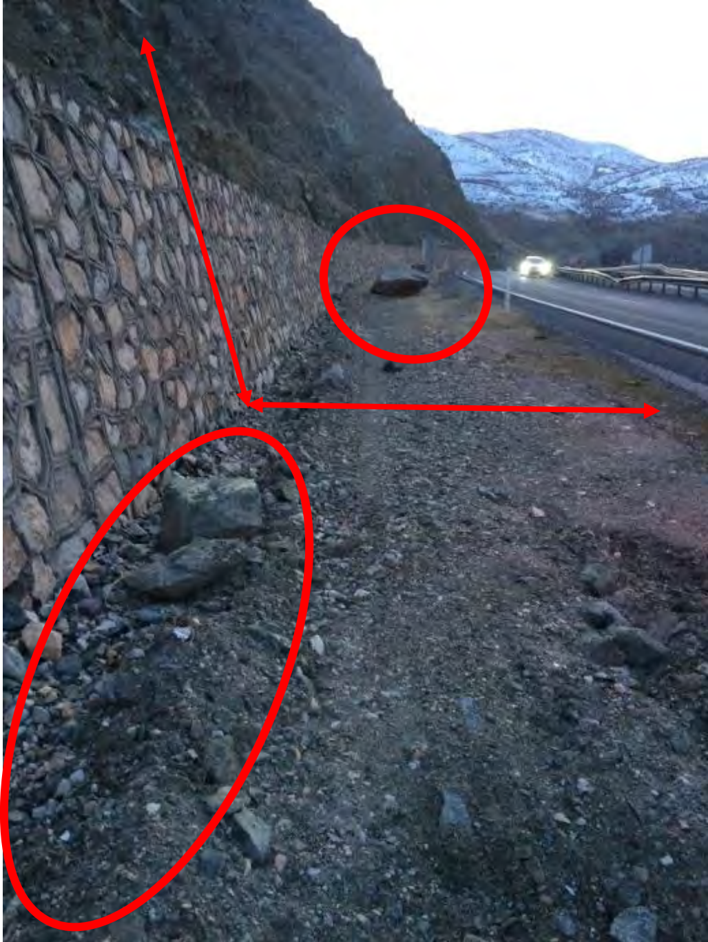
Figure 4.59. Fallen rocks on the highway (38°26'19.8"N 38°49'38.8"E / 01.02.2020 / 7:23)
