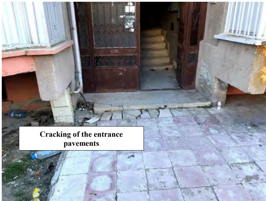
Figure 4.98. Cracking observed at the entrance of the of a residential building ( 38^{\circ}39'21.9''N 39^{\circ}09'10.4''E / 01.02.2020 / 14:50)
