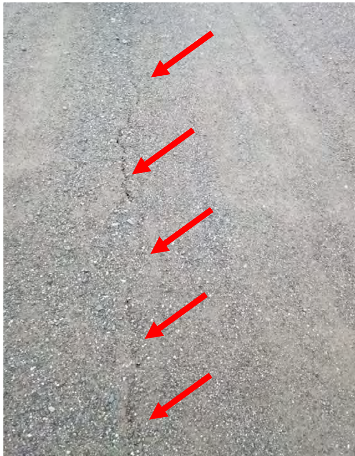
Figure 4.119. Longitudinal cracks on Dedeyolu Dam crest (DSI)
