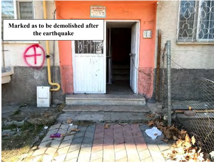
Figure 4.97. A residential building located in the Abdullah Paşa district of Elazığ city center ( 38^{\circ}39'25.2''N 39^{\circ}09'10.3''E / 01.02.2020 / 14:45)
