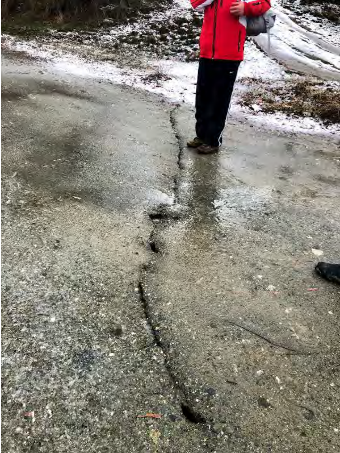
Figure 4.18. Another view of seismically-induced lateral spreading cracks ( 38^{\circ}26'50.7''N 39^{\circ}18'55.4''E / 31.01.2020 / 12:36)
