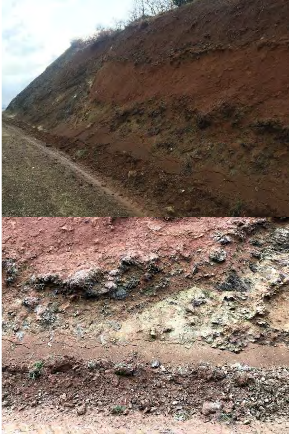
Figure 4.52. Side view of the slope (38°30'11.7"N 39°23'33.4"E / 31.01.2020 / 16:34 & 38°30'11.8"N 39°23'33.3"E / 31.01.2020 / 16:34)
