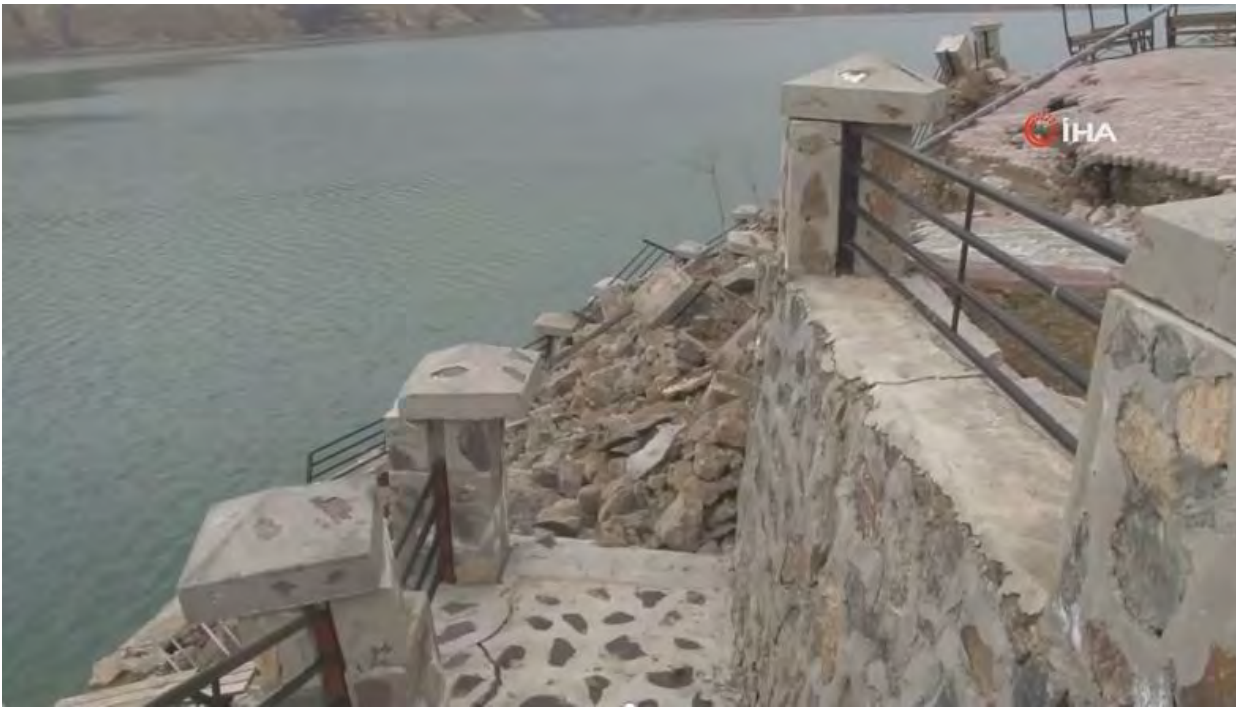
Figure 4.58. Doğanyol Port Failure adapted from IHA report (38°33'34.6"N 39°04'10.6"E)
