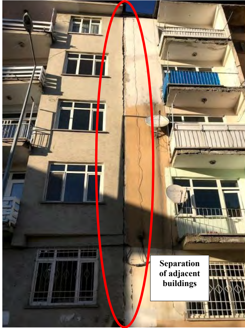
Figure 4.109. Longitudinal cracks observed on a building located in the Mustafa Paşa district (38°40'15.9"N 39°13'59.9"E / 01.02.2020 / 16:34)
