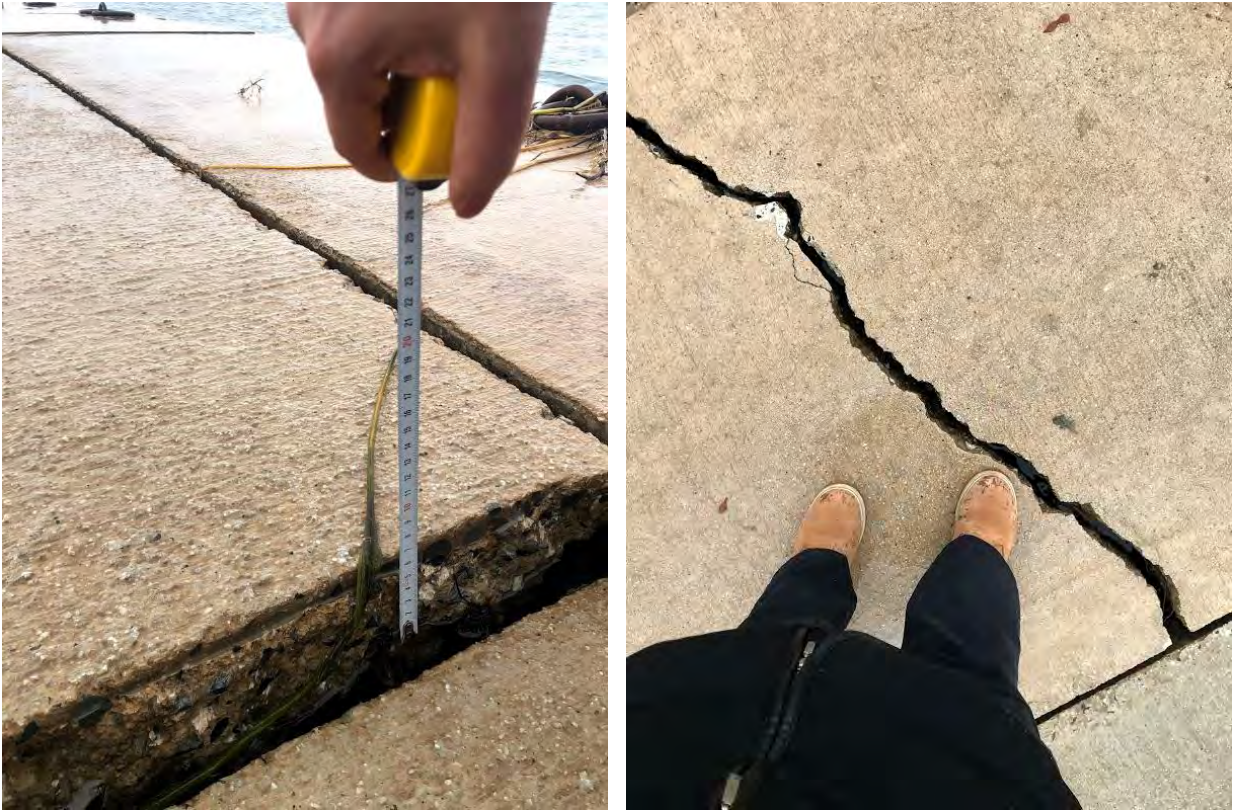
Figure 4.13. Measurements of seismically-induced volumetric settlement in the dock of Hazar Lake ( 38^{\circ}26'53.1''N 39^{\circ}18'53.6''E / 31.01.2020 / 12:16 & 38^{\circ}26'53.2''N 39^{\circ}18'52.9''E / 31.01.2020 / 12:13)
