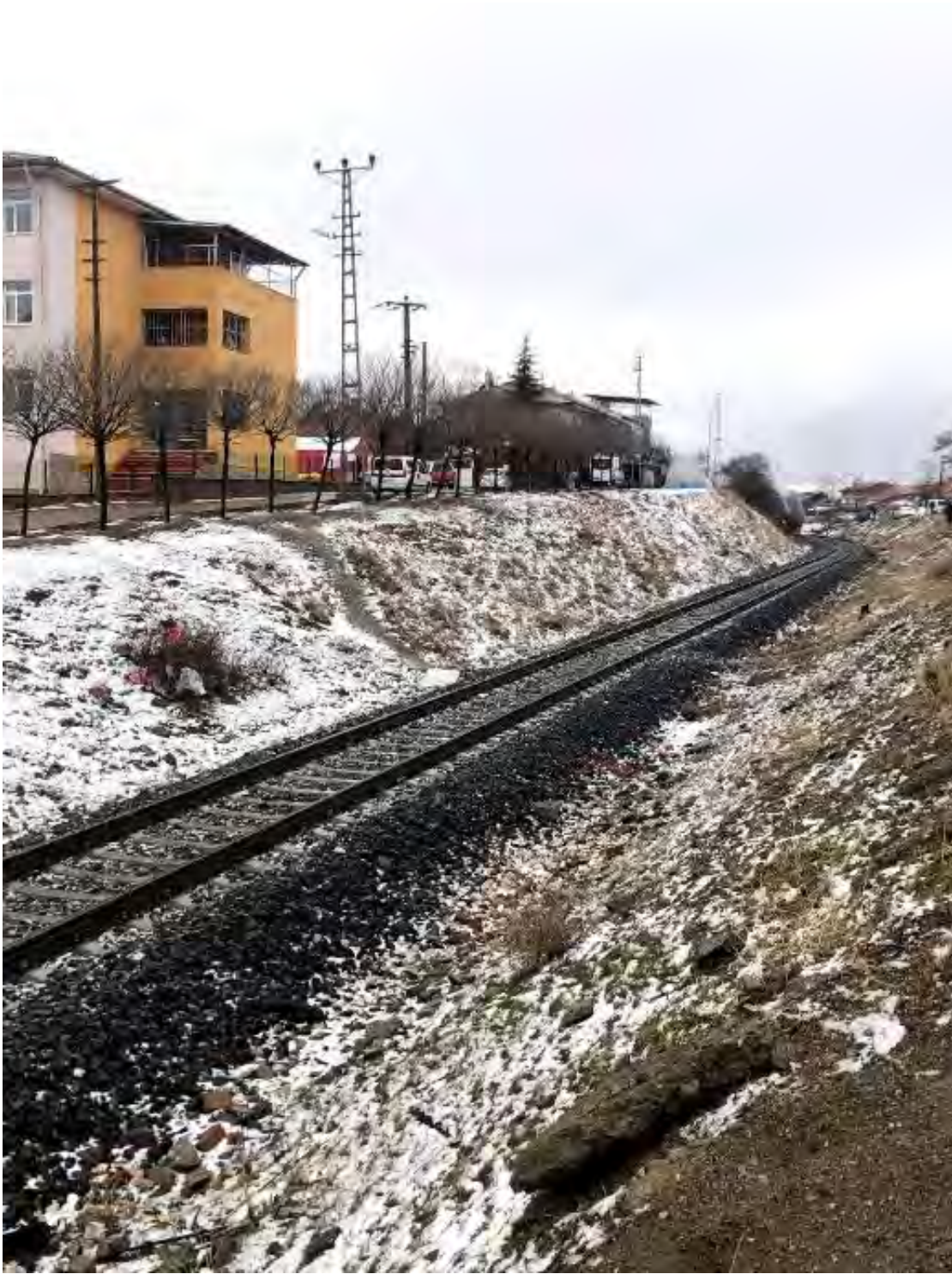
Figure 4.23. A view of railway tracks without any damage at Sivrice ( 38^{\circ}26'49.5''N 39^{\circ}18'33.4''E / 31.01.2020 / 13:29)
