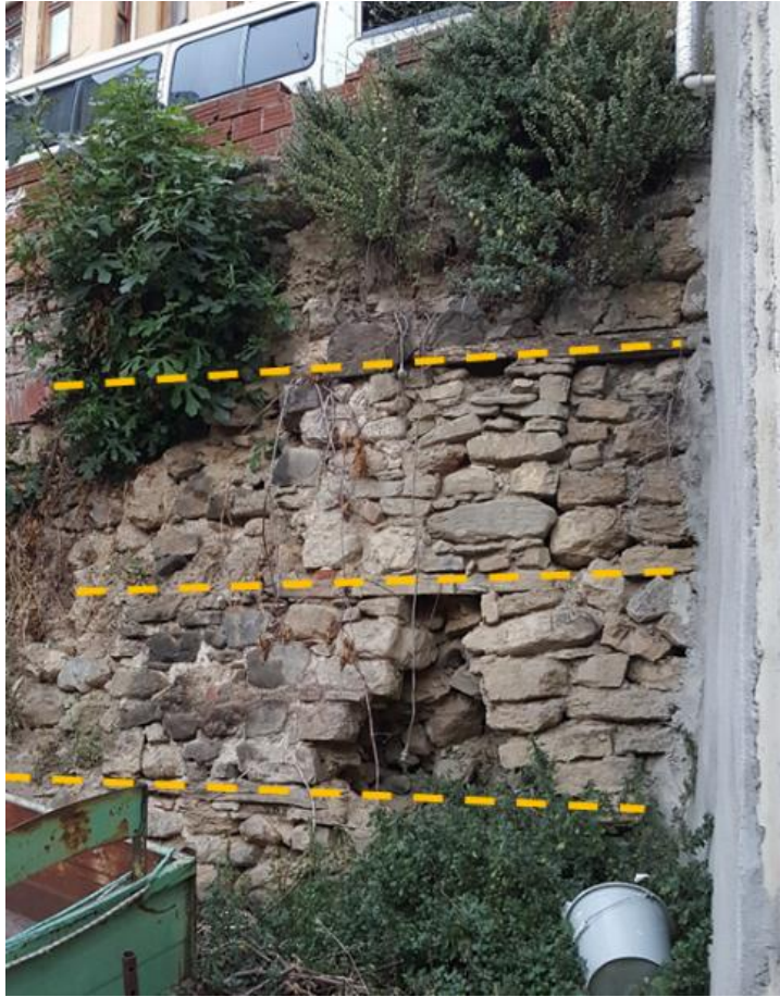
Figure 3.13. Timber lintel levels on the highly deteriorated stone masonry wall (Cami street Lot no: 2186/2)
