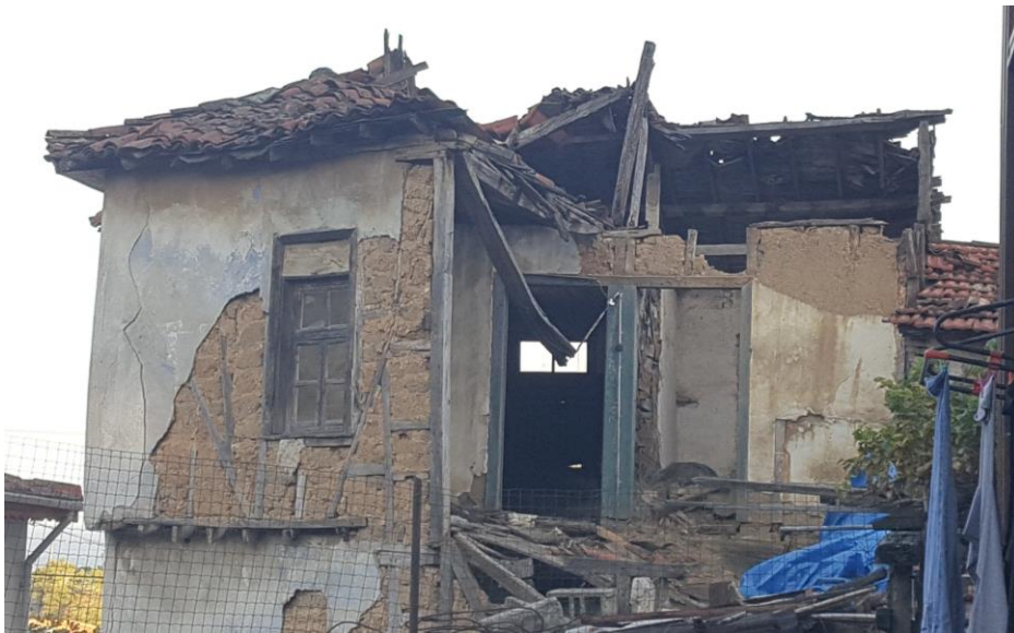
Figure 3.41. An example of the deteriorated 3-sided roof structure
