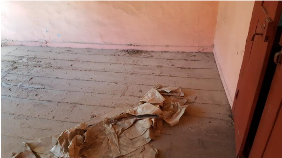
Figure 2.74 Timber floorboard covering at the mezzanine floor M2 space of the studied houses no 4
