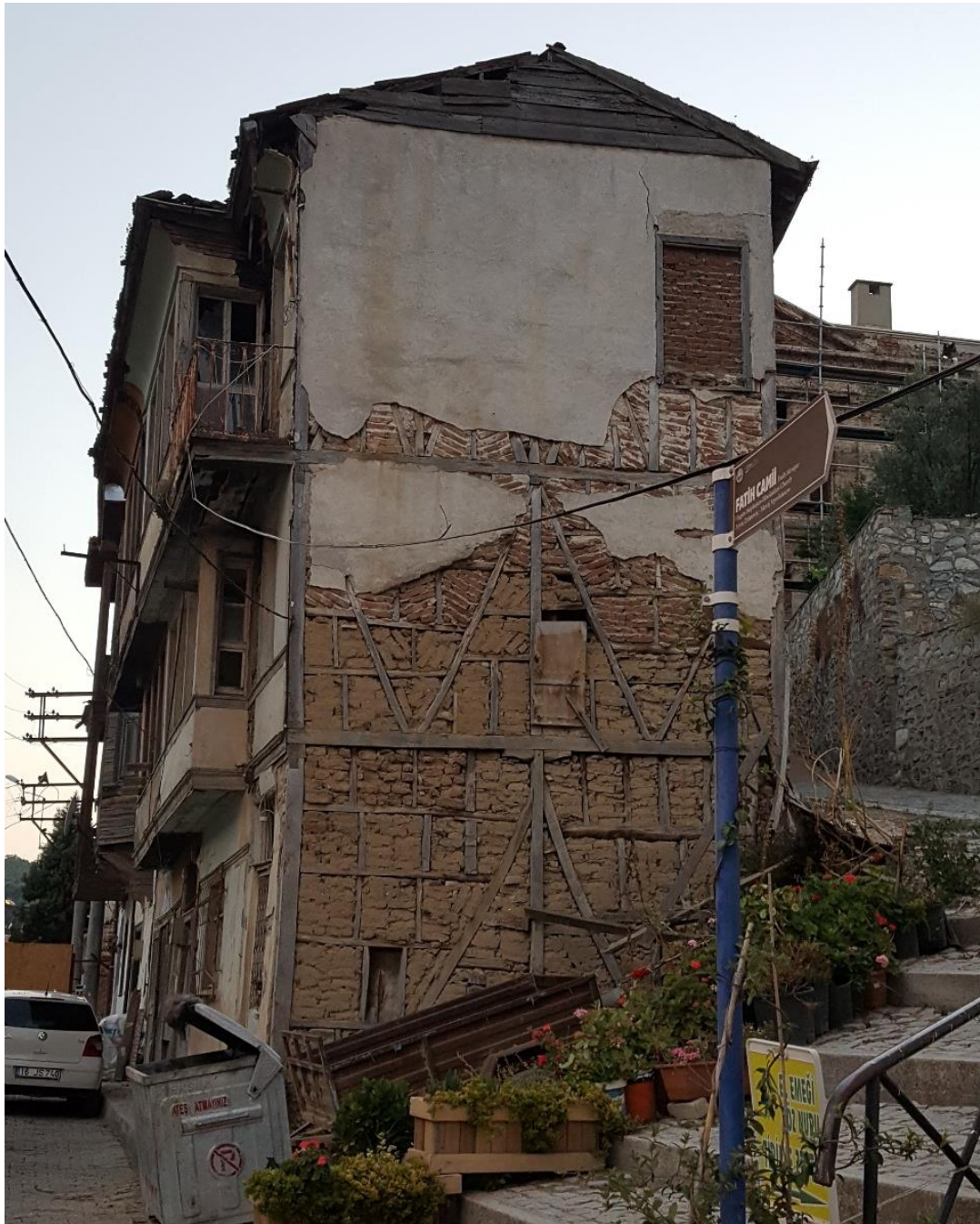
Figure 3.17. An example for timber frame wall usage on the ground, mezzanine, and top floors (House No:2, Eskipazar St, Lot no: 2188/7)
