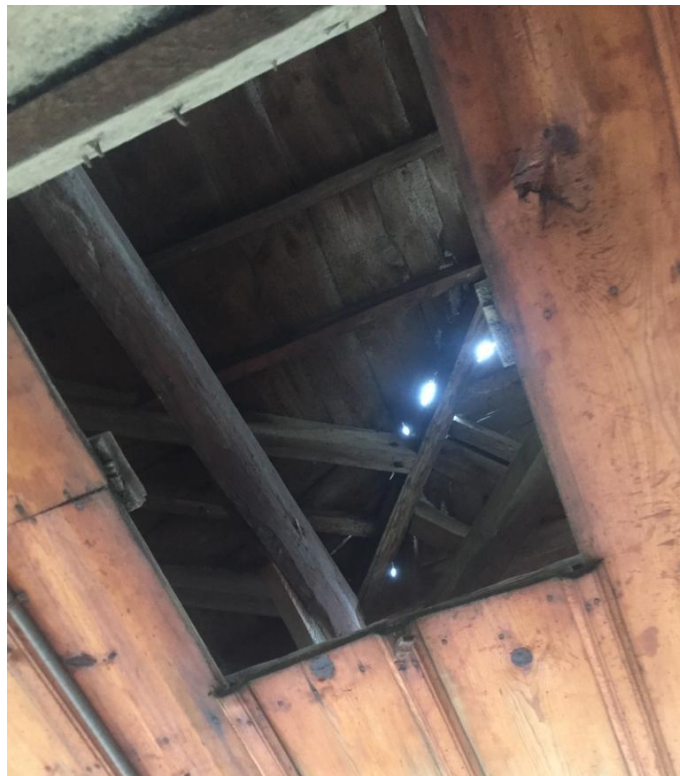
Figure 3.46. The roof structure of House No.1 is seen from the opening at the top floors' timber ceiling
