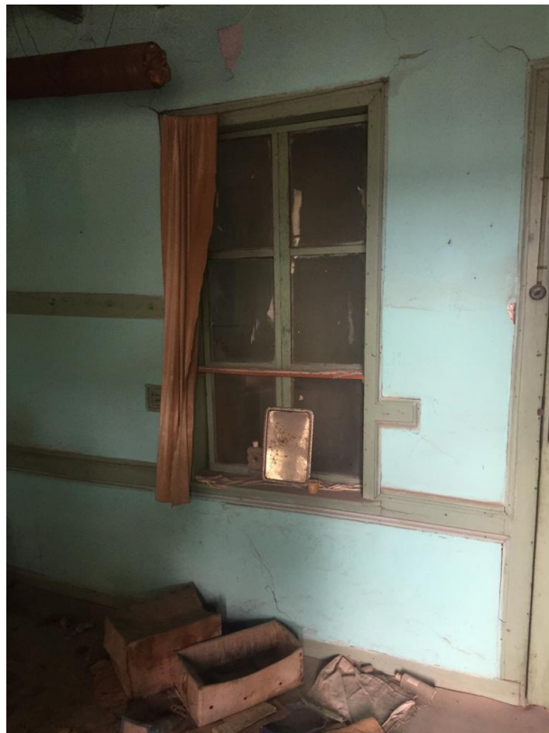
Figure 2.69 Interior window opening on partition wall of the room in the first floor (F2 space) of House No:1 (Eskipazar Street, lot no: 2192/5)
