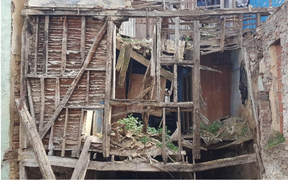
Figure 3.23. Highly deteriorated example of a timber frame wall, with timber lath covering on the interior face with plaster (House No:10, Eskipazar St, Lot no: 2245/11)
