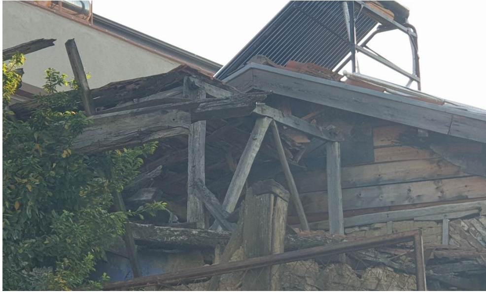
Figure 3.44. Highly-deteriorated roof structure and the connection of king posts, ridge purlin, and braces
