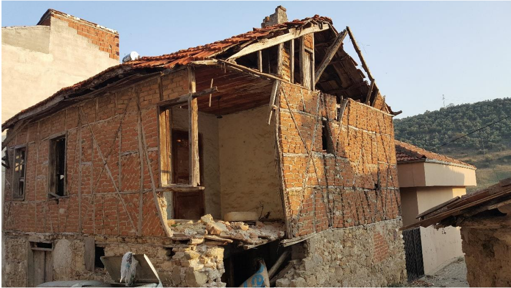
Figure 3.40. An example of the deteriorated gable roof structure
