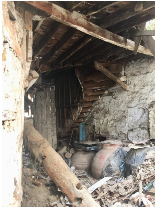
Figure 2.48. Taşlık space of the House No:10 is seen through the collapsed back façade (Eskipazar St, Lot no: 2245/11)
