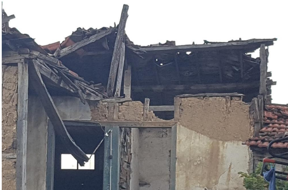
Figure 3.45. Highly deteriorated timber roof structure, purlins are below the rafters
