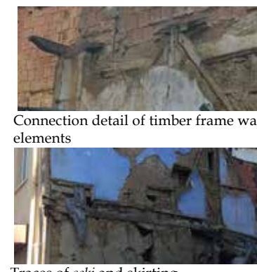
Traces of seki and skirting, gap between wall plate and skirting shows the missing floor girders
