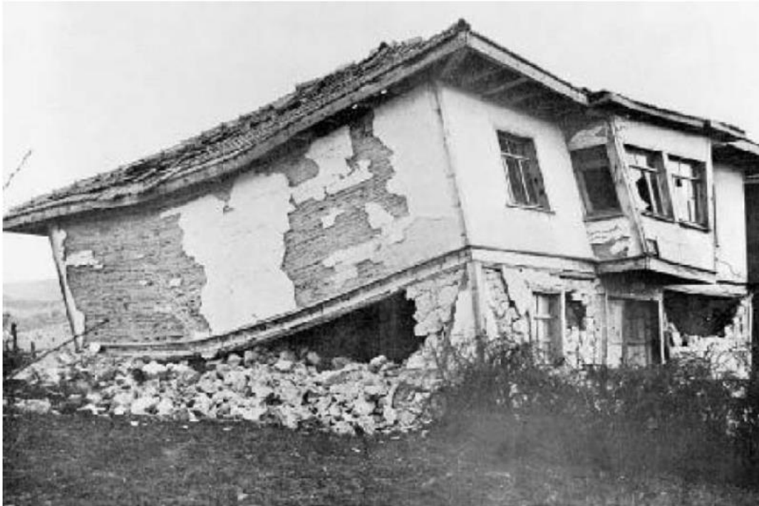
Figure 4.1. Traditional house in Iğdiş village after 1970 Gediz earthquake, destruction of ground floor masonry wall of a traditional house while the timber-frame upper floor still preserves its integrity (Şahin Güçhan, 2007, p.843, fig no:1)
