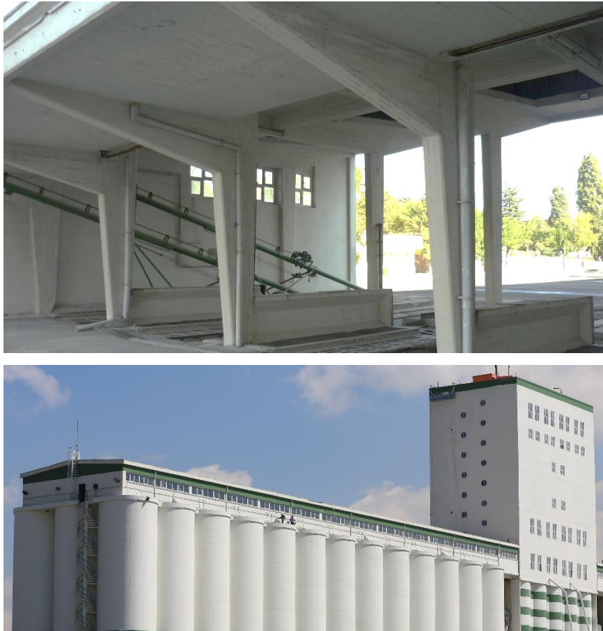
Figure 3.45. Photographs show modern forms on structural elements (top) and windows in horizontal, circular, and vertical forms with spiral fire escape (bottom) (Author, 2020).
