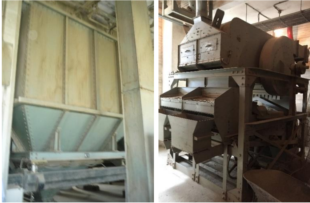
Figure 4.24. Examples of fixed equipment to be preserved in the central core. Weighers in the weigher floor (left) and sieves in the cleaner floor (right) (Author, 2020).
