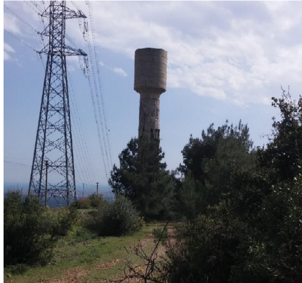
Figure 5.2 Surge Tank of Kepez – I HPP
