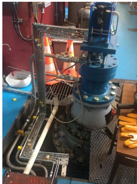
Figure 2.6 Photograph of PRV in KEPEZ - I HPP
