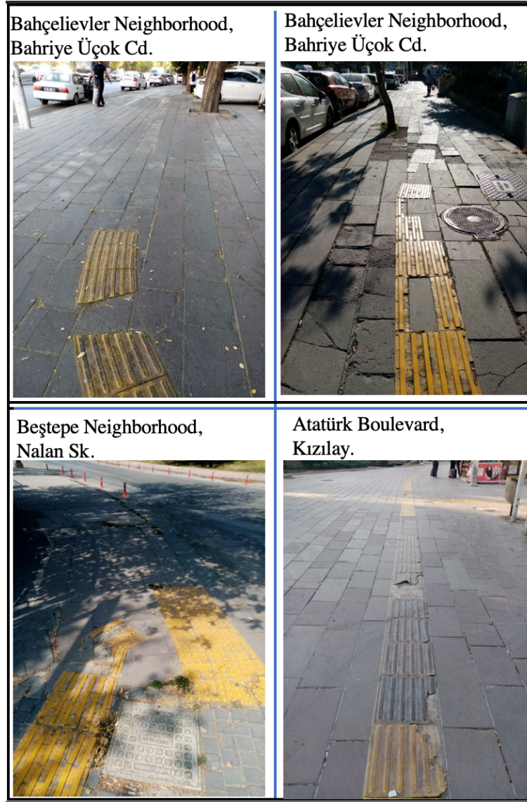
Figure 5.20. Problematic Implementation Examples of Tactile Pavement (Photographs Taken During Fieldwork)
