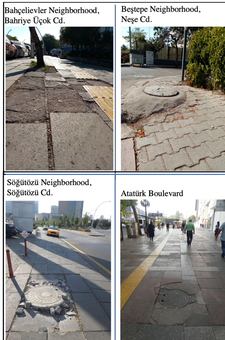
Figure 5.10. Surface Problems on Sidewalk (Photographs Taken During Fieldwork)
