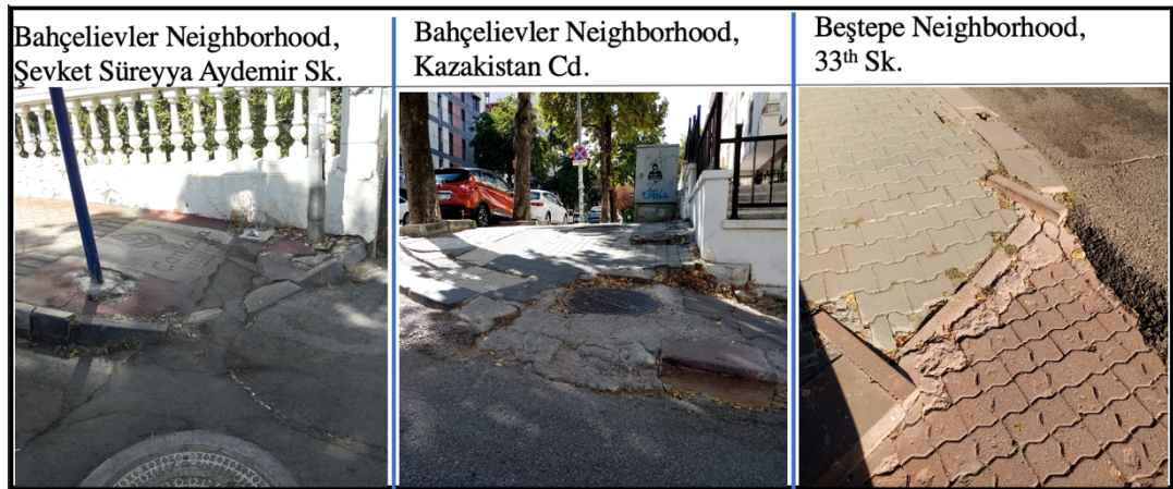
Figure 5.34. Example Images from Problematic Ramp Surfaces in Case Study Areas (Photographs Taken During Fieldwork)
