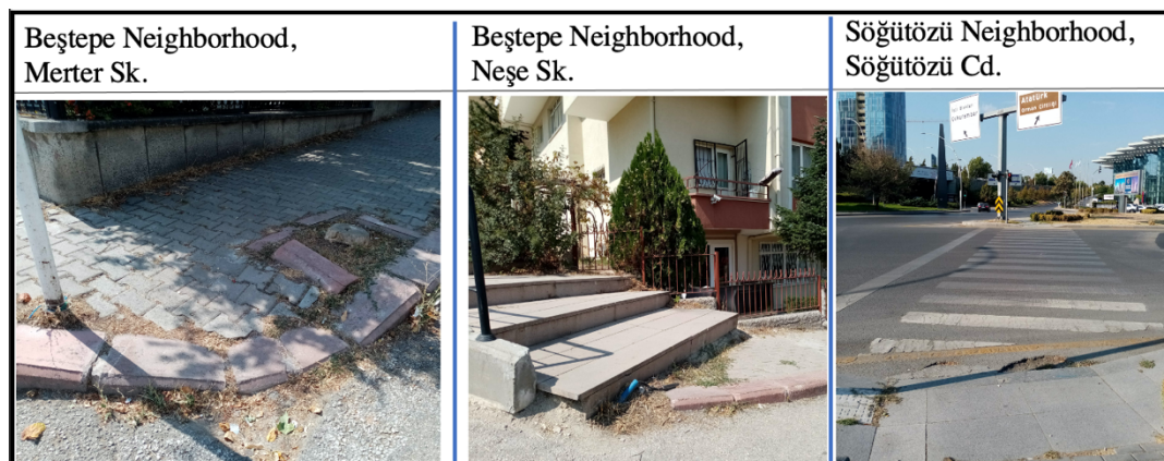
Figure 5.36. Example Images from Problematic Ramps at Crossings (Photographs Taken During Fieldwork)
