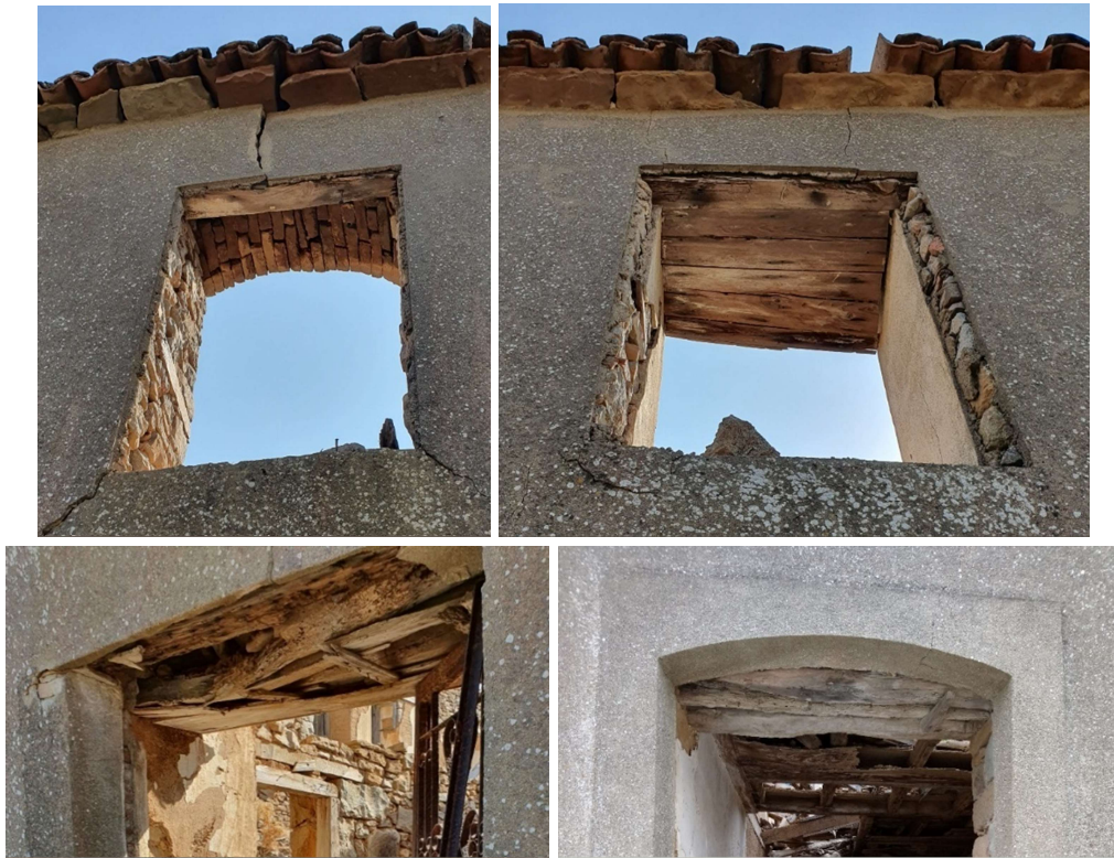
Figure 3.52. Dereköy, a brick arch above a window opening (above left); the linteled opening with wooden laths (above right); a linteled opening (below left); the combination of an arch and a lintel (below right)
