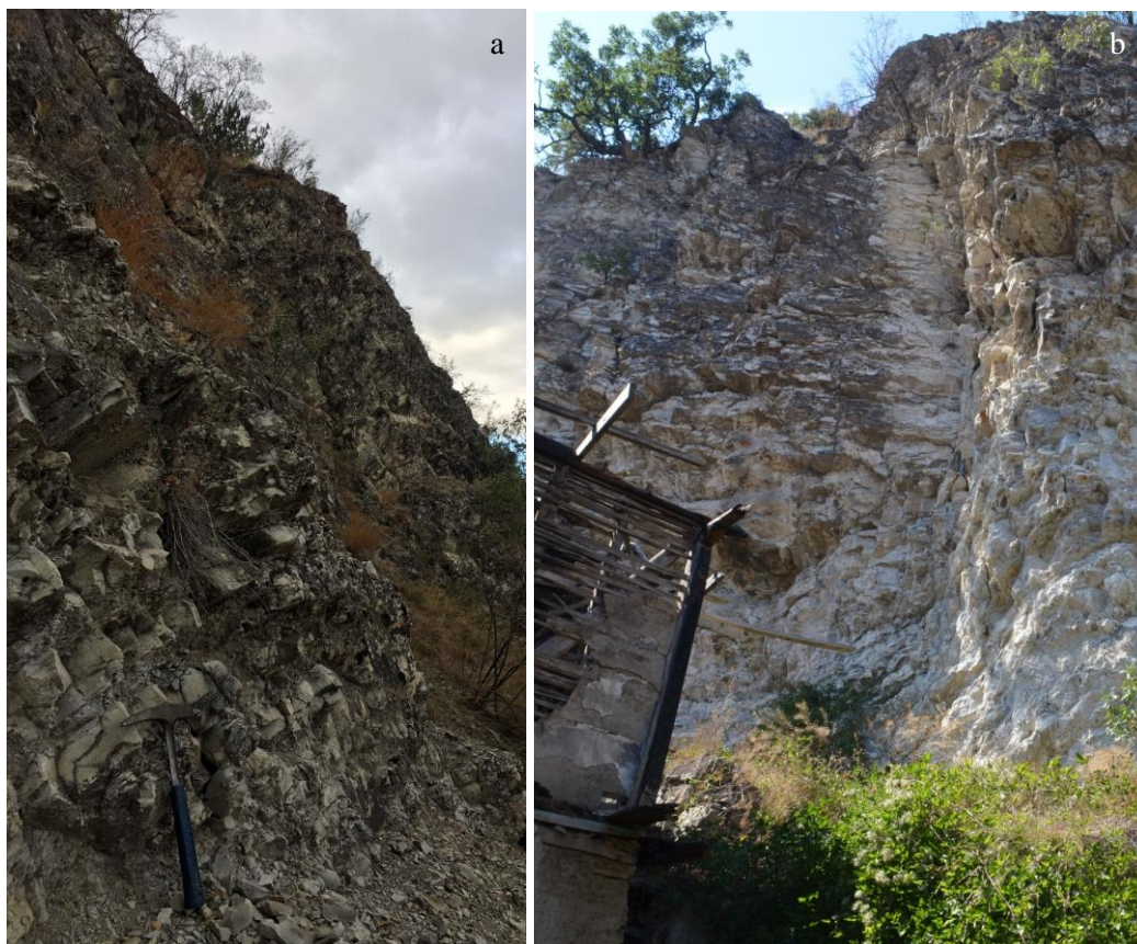
Figure 99: Example images for different failure types possible on the western side of the Mudurnu valley. a) Toppling (lower leftern side) and planar (upper part) failures, b) wedge failure
