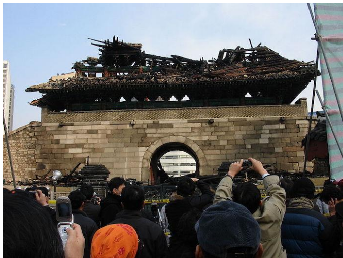
Figure 3 The Namdaemun gate in Seoul, South Korea, after a fire in 2008 [URL 6]
