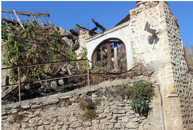
Figure 8 Some samples of burnt traditional buildings that were investigated during the site survey conducted in October 2020
